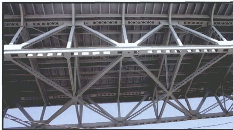
Image 4: Detail of Warren deck truss and I-beam grating, Image courtesy of EHT Tracerics, May 2006
