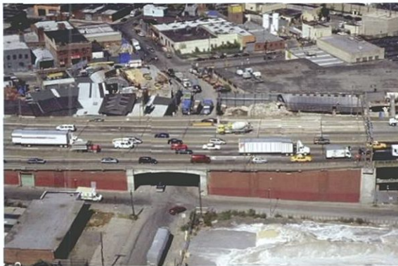
FIGURE 3: AERIAL VIEW OF THE BROOKLYN CONNECTOR (CONCRETE VIADUCT AND CLOSURE WALL) AT VARICK AVENUE
