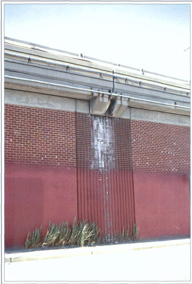
Photo V-21. Detail of sawtooth brick elements on exterior of bridge abutments, on the Brooklyn side
