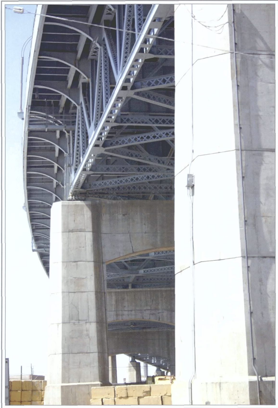
Photo 6: Detail of concrete piers and substructure, looking northeast from Greenpoint, Brooklyn, New York
