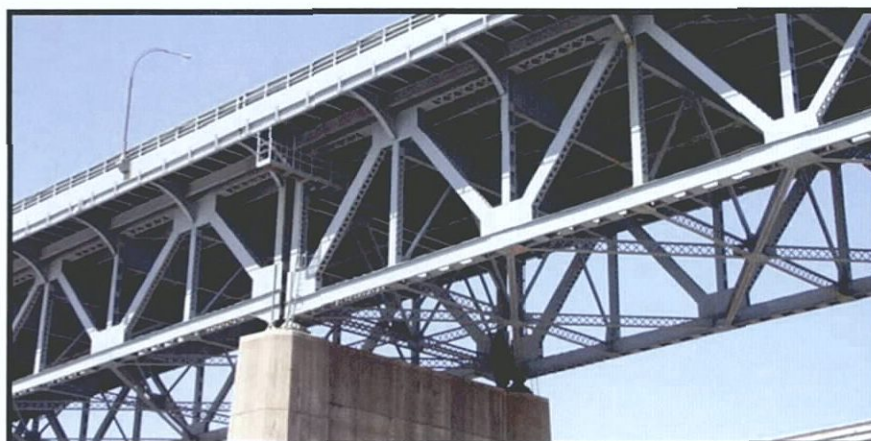
Image 25: Detail showing Warren deck truss of the Kosciuszko Bridge EHT Traceries, May 2006
