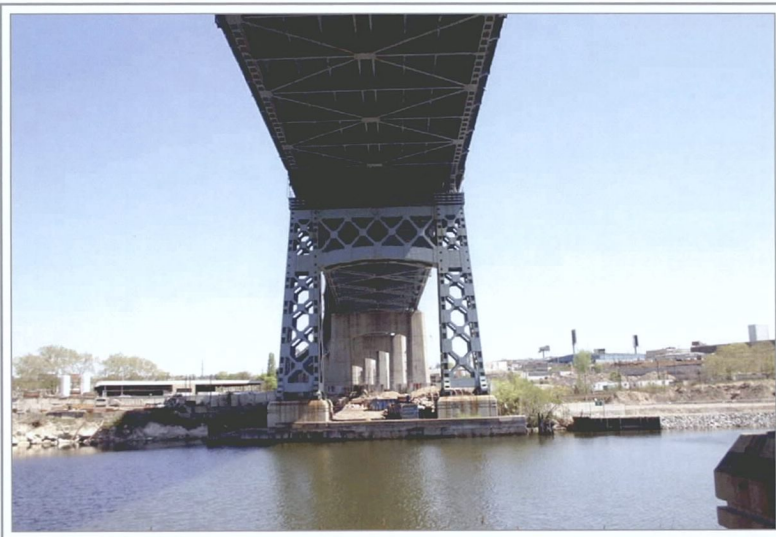
View of Kosciuszko Bridge supports over Newtown Creek, looking northeast from Greenpoint, Brooklyn, New York
