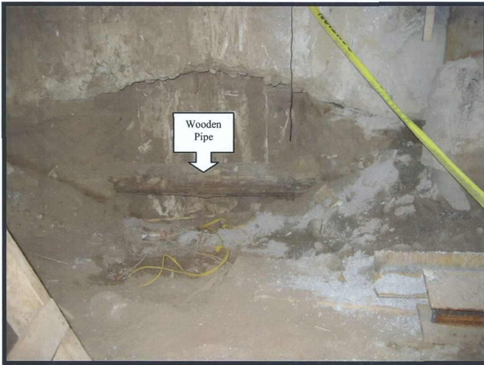
Photograph 5.18 Closeup of exposed wooden water pipe section, looking north.
