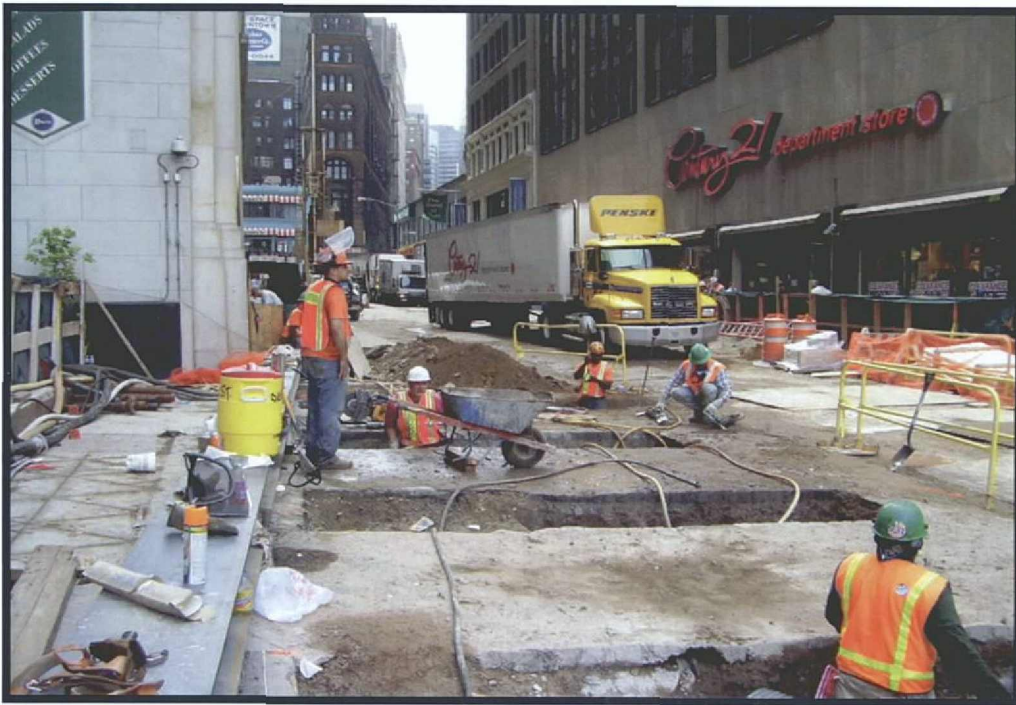
Photograph 5.1 Hand excavation of initial deck beam trenches along north side of Dey Street, looking east
