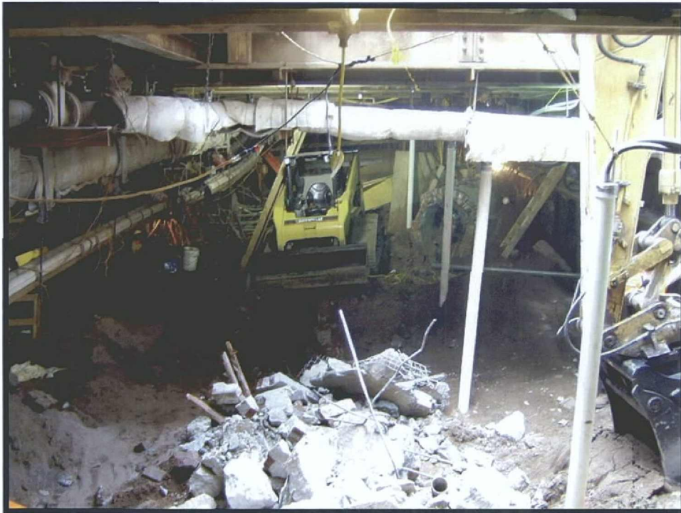
Photograph 5.12 Below decking excavations in the western half of Dey Street, showing utility disturbances.
