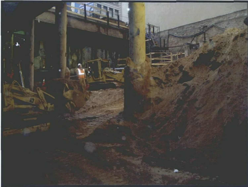
Photograph 5.19 Excavations beneath eastern end of Dey Street West, looking southeast toward the former location of 189 Broadway.
