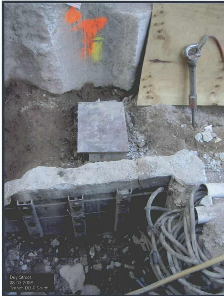
Photograph 5.8 Utility disturbance in Trench DB-6S, looking south.
