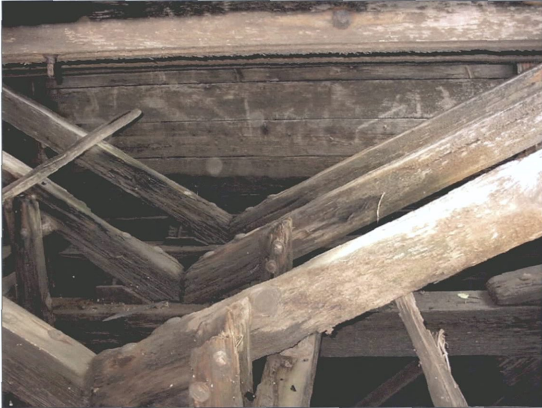
Figure 5-105. Port wing trusses, with bulkhead in background. View to the north (forward).
