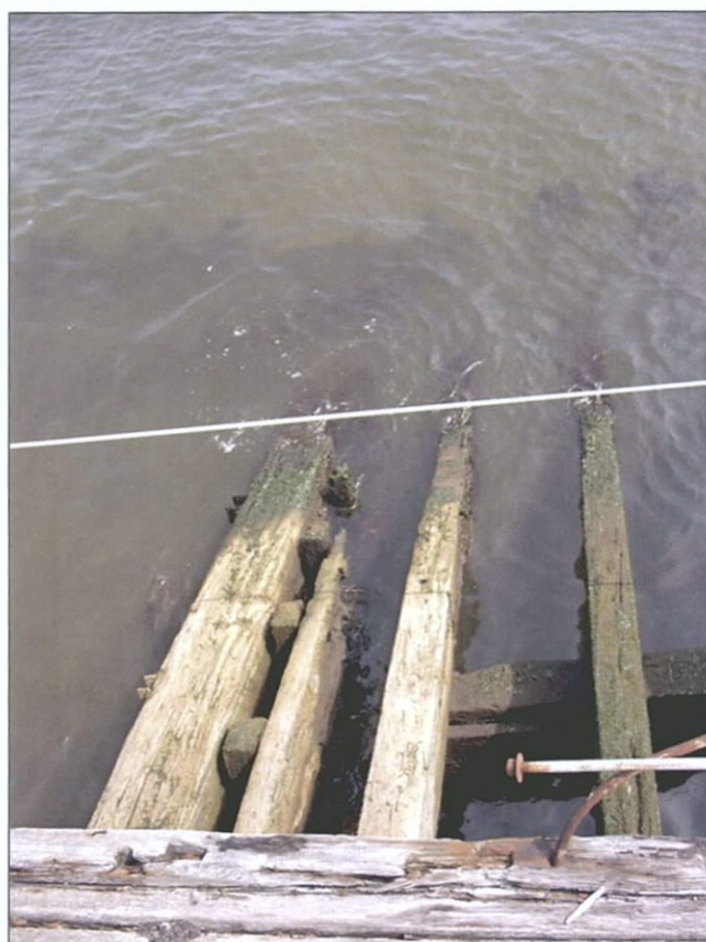
Figure 7-66. Detail of top of aft bulkhead showing support beams and stanchion tops, looking port (east).
