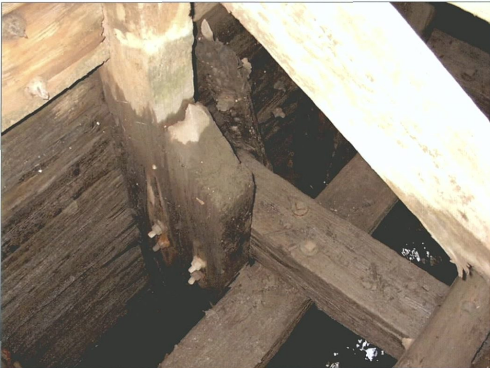
Figure 5-56. Side frame detail just above main deck, port wing. Note termination of inner futtock.
