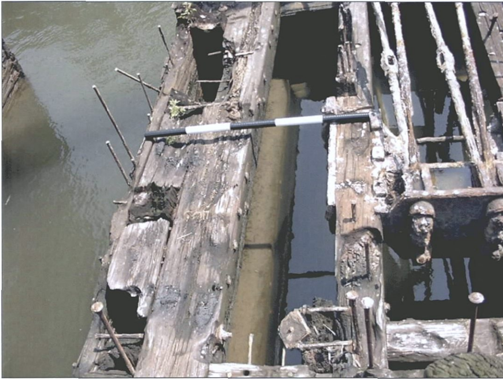
Figure 5-53. Vessel end frames on northern exposed end of V1. Note spacing and chocks. View to the east.
