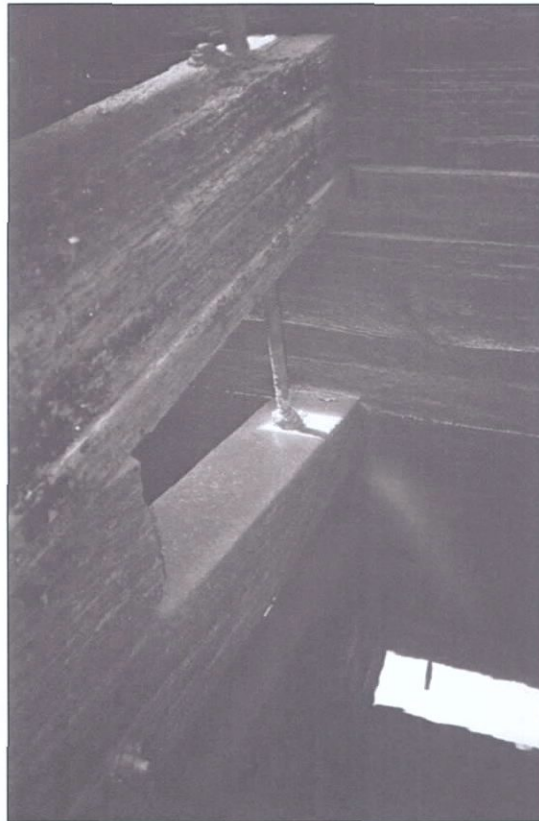
Figure 5-64. Main truss (T1) (top) and secondary truss (T2) meeting longitudinal bulkhead. The third truss (T3) is barely visible below the water. View to the south (port side).
