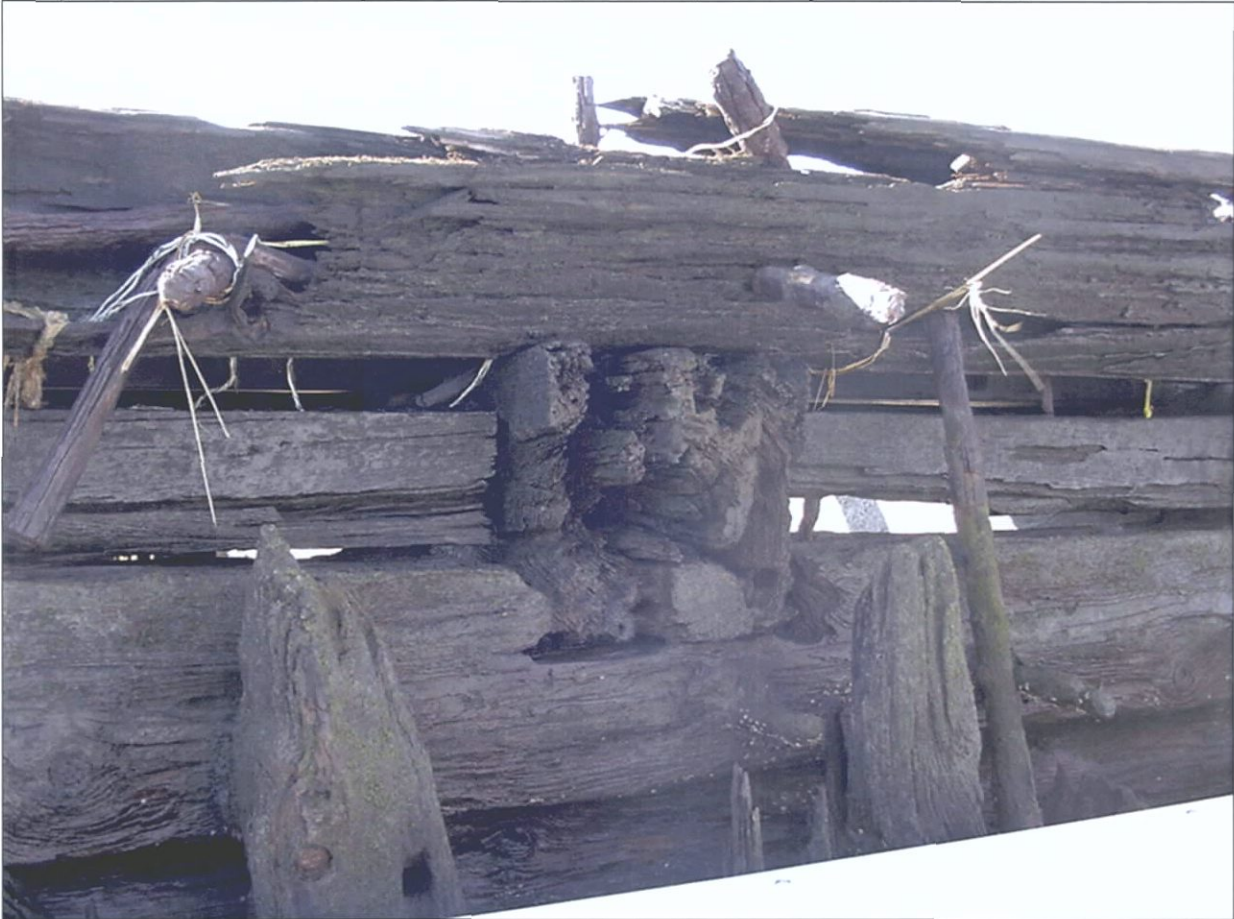
Figure 6-87. Starboard midships showing cargo deck beams in relation to clamp and frames. View to the south.
