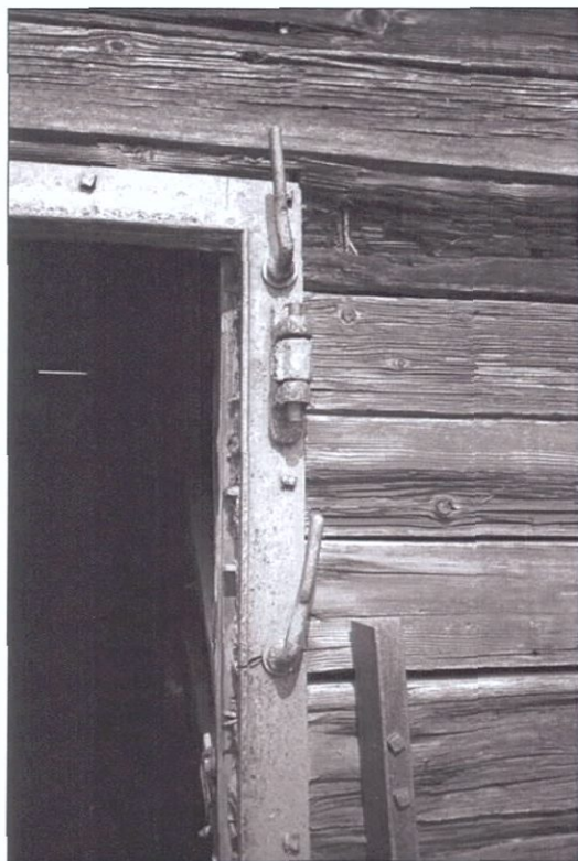
Figure 5-138. Hatch frame detail. Note hinge, hatch dogs, and fasteners. Port wing, view to the west.
