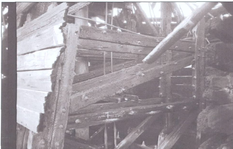
Figure 5-101. Wing truss above main deck level. Starboard wing. View to the northeast.
