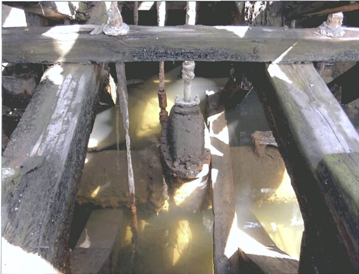
Figure 5-151. Gate valves in inlet (below) and outlet (center) pipes. Port side, view to the west.
