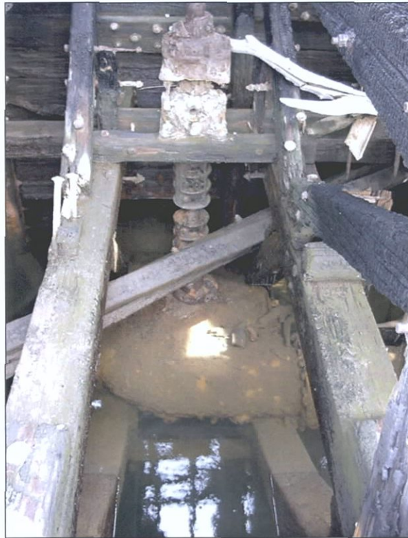
Figure 5-149. One of two impeller casings with vertical drive shaft connected to electric motor on top deck of wing. Port wing, view to the west (port).
