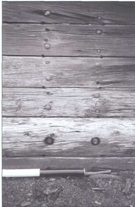
Figure 5-124. Wing chine and wing plank fastener pattern at bulkhead location. Note two types of fasteners. View to the west (port).
