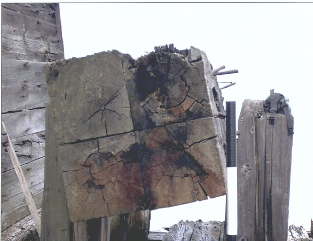
Figure 5-69. Section of remaining coupling timber in port forward bitt. View to the north.
