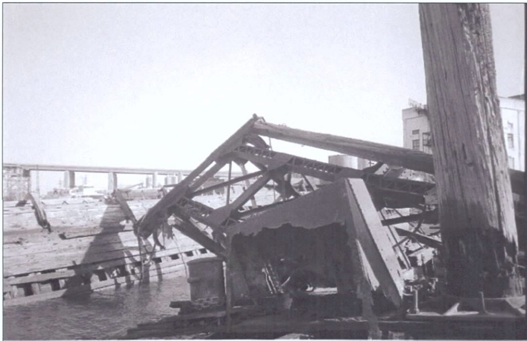
Figure 4-61. Spud box and a pole, and collapsed A-frame at the aft end of the vessel. View to the southeast (forward).
