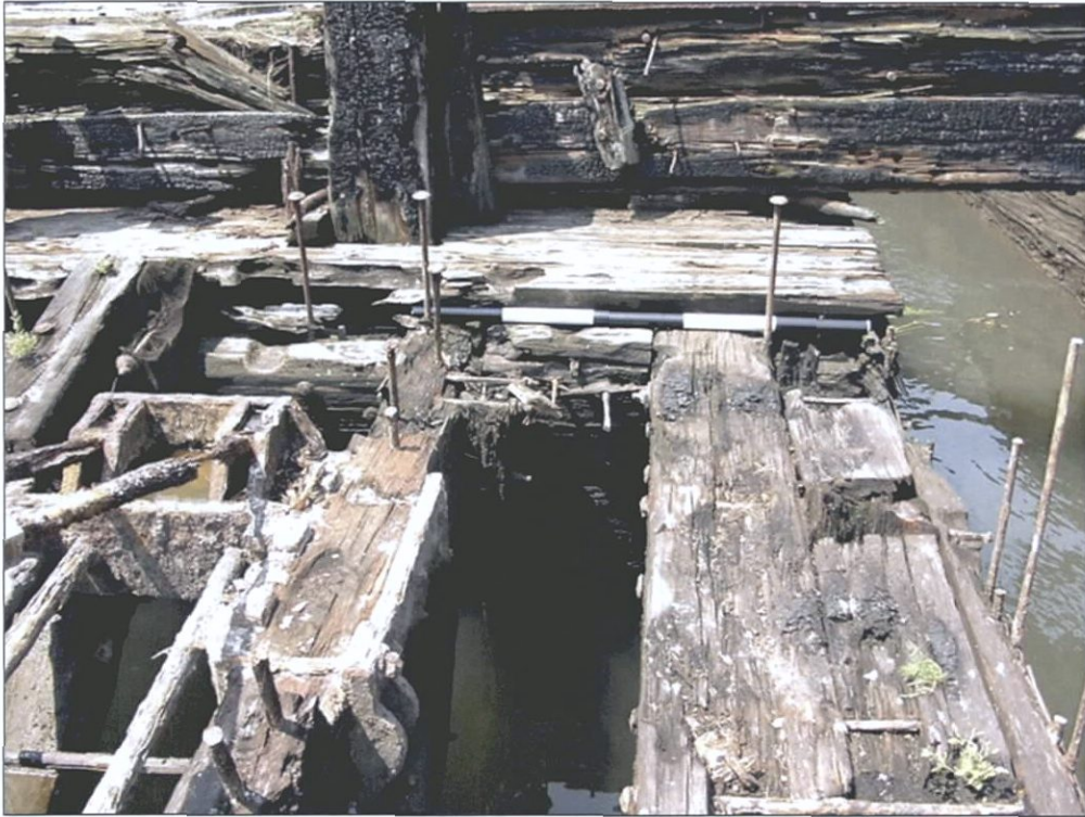
Figure 5-37. Northern exposed end of V1, showing top end log (right of center) and chocks between frames. View to the west (port).
