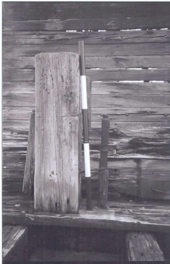
Figure 5-71. Cinch bolt on forward port bitt. Cradle has eroded or been removed. Lag bolt extends to framing below. View to the west.
