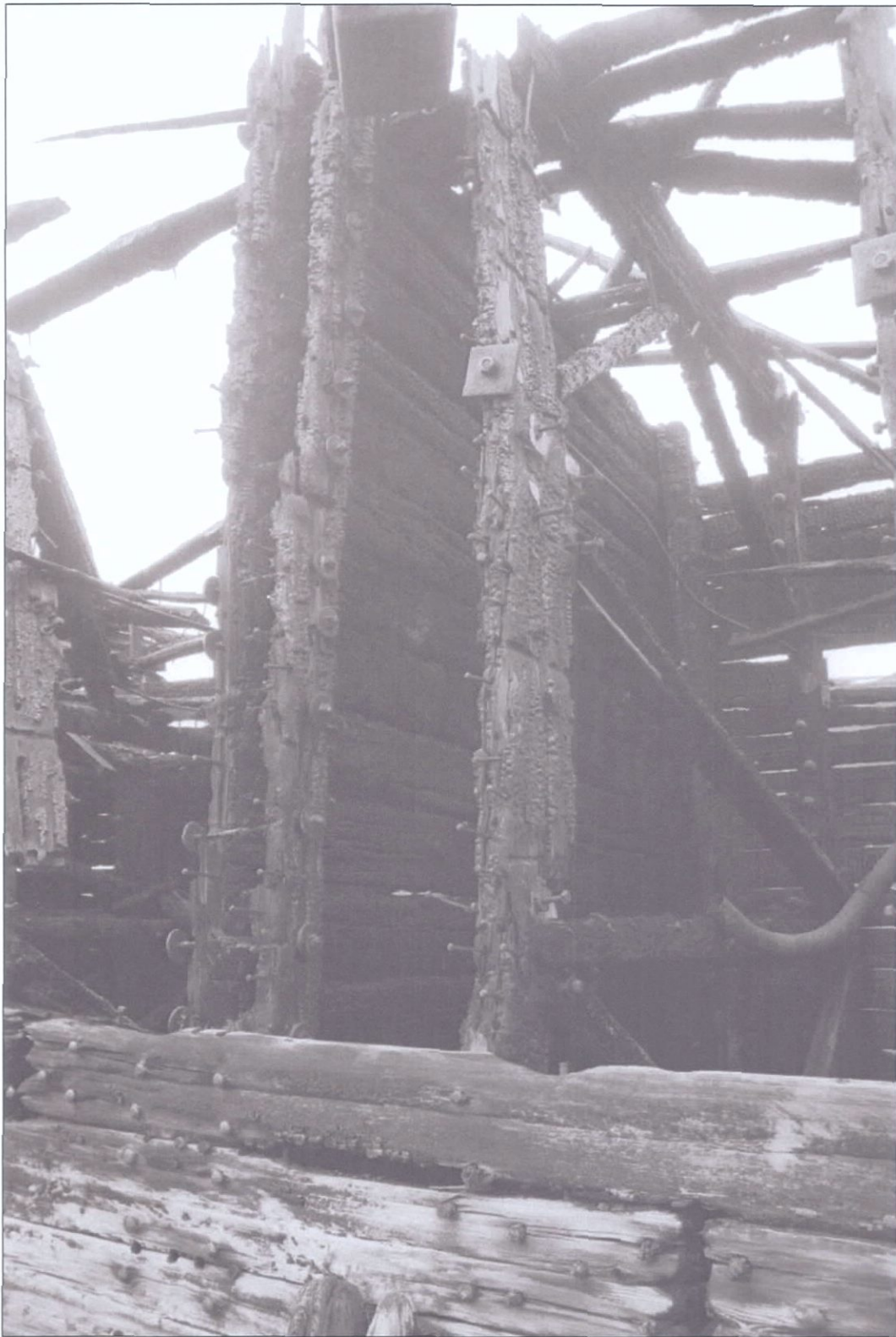
Figure 5-44. View of forward side of watertight bulkhead in starboard wing. Pontoon bulkheads are of similar construction.
