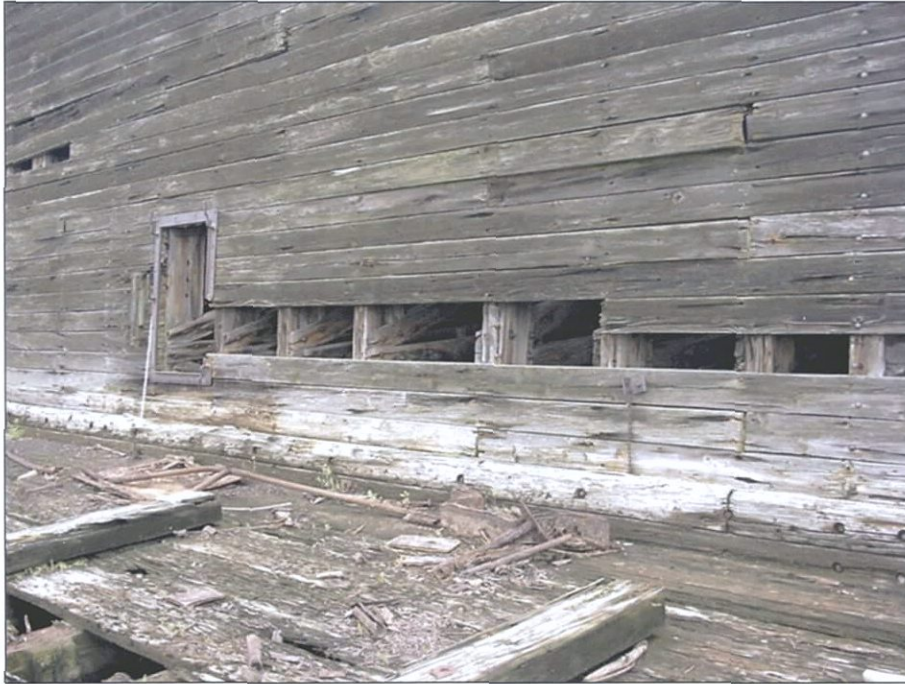
Figure 5-119. Port wing showing wider inner wing plank below level of middle deck. Note also chine logs. View to the southwest.
