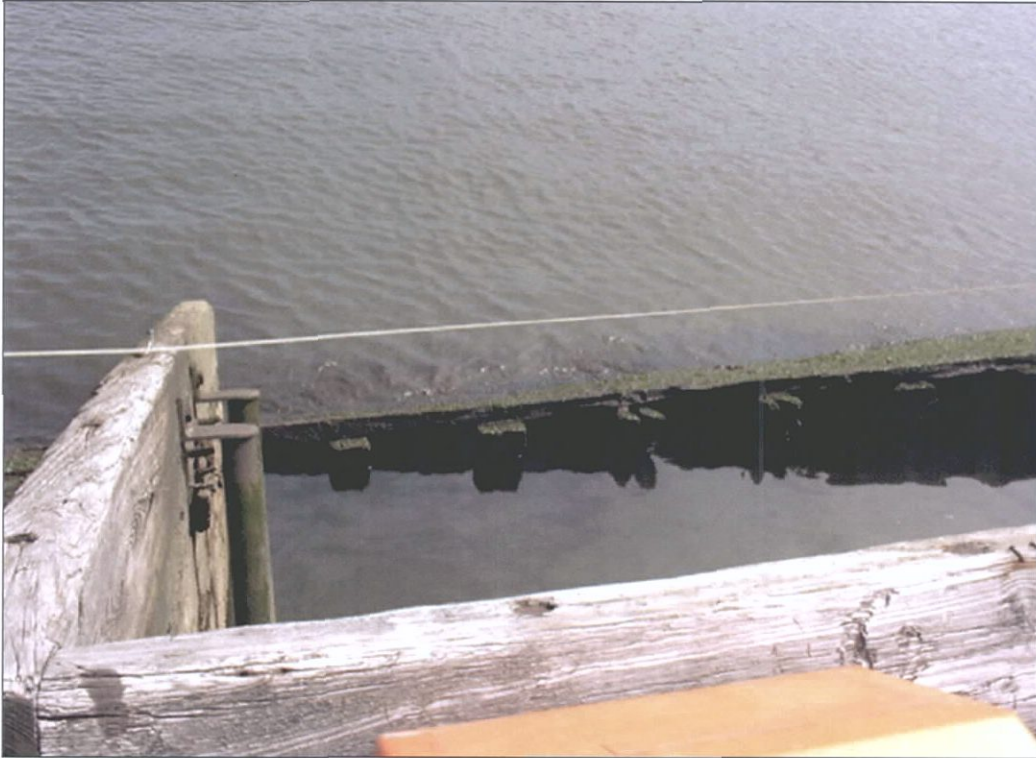
Figure 7-59. Exposed main deck beams along port side of main cargo hatch, looking east.
