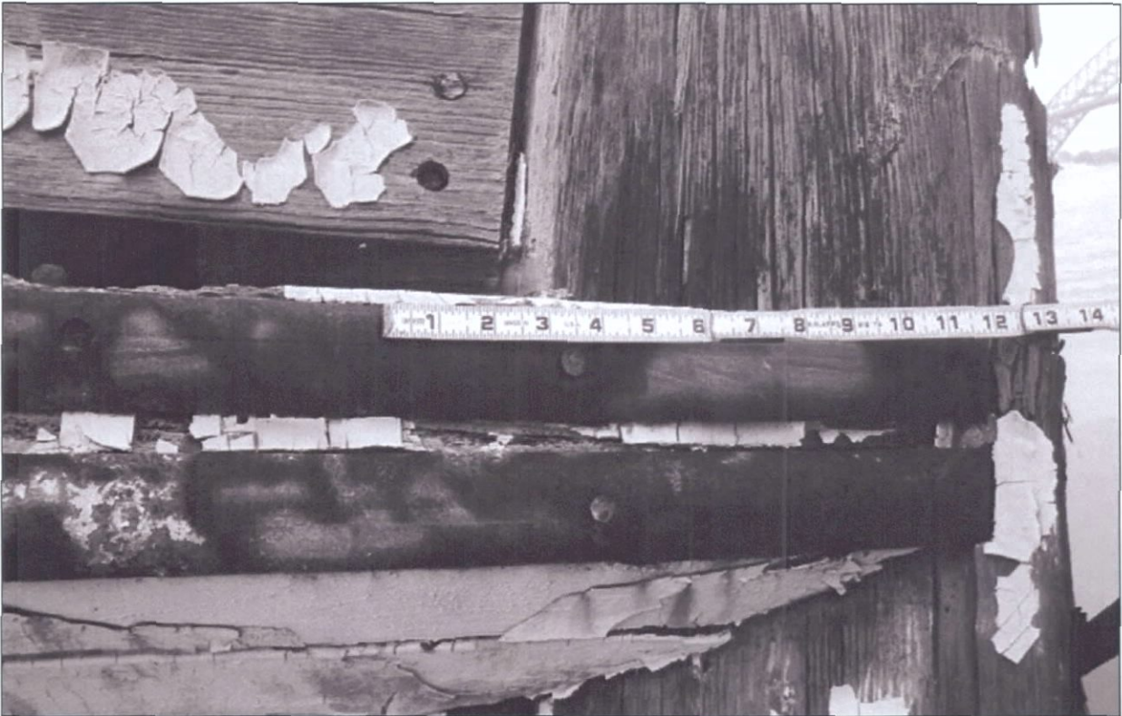
Figure 7-57. Main rub rail where it meets the starboard side of the stem. Note iron half-round caps.
