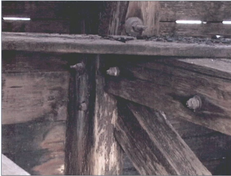
Figure 5-98. Outer wall wing framing at upper deck, port wing. Note deck planking.
