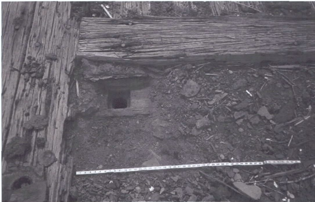
Figure 5-85. Deck drain with cover and straining screen removed. View to the south (aft).
