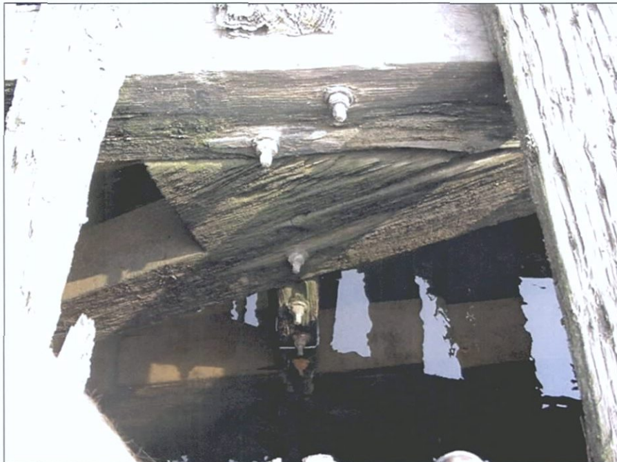
Figure 5-60. Truss 6 at main deck beam. Note triangular chock between truss and beam, and narrow vertical chock below truss opposite stanchion. View to the north (forward).
