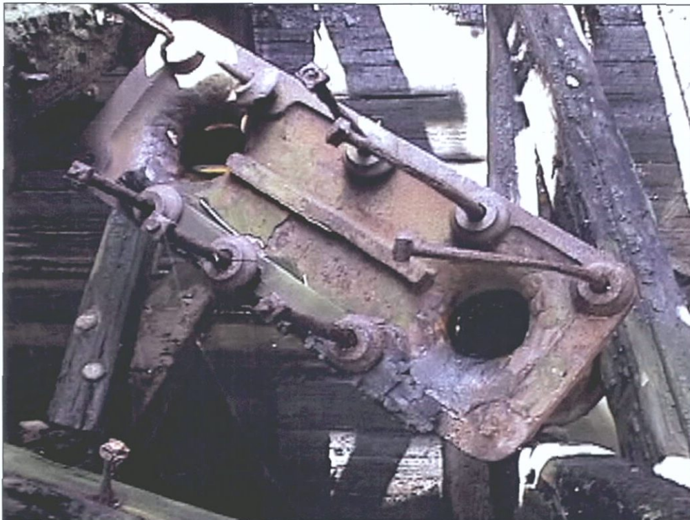
Figure 5-147. Underside of a bollard that has fallen through the upper deck. Starboard wing, view to the south (aft).
