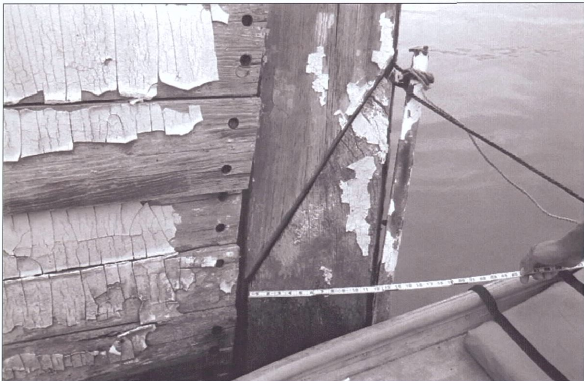
Figure 7-44. Close-up of stern showing scarp joint. Also note stem band. View to the east (port).
