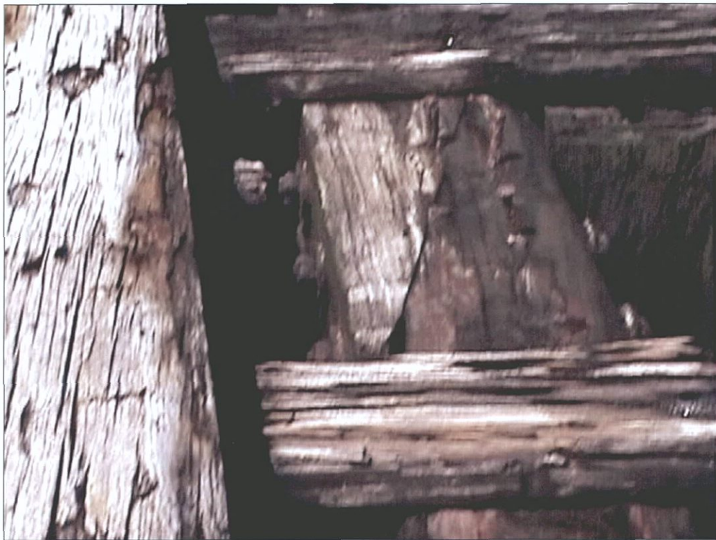
Figure 5-39. Top end log scarph joint, fastened with four bolts. View to the west (port).
