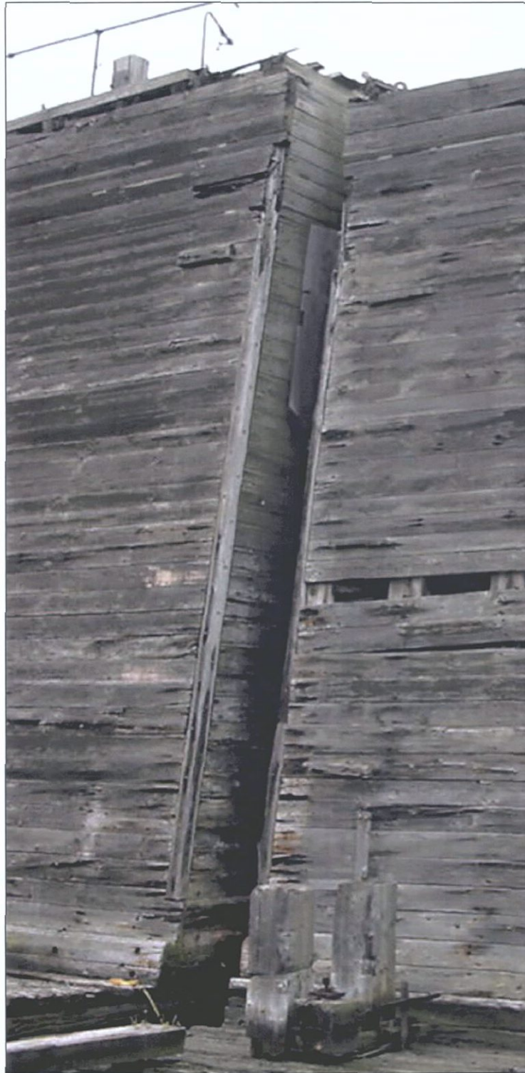
Figure 5-143. Aft area of port wing showing remnants of ladder mount. View to the southwest (port).
