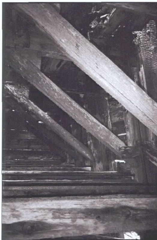
Figure 5-115. Upper diagonal wing truss beams. Note chocks at joint with second deck beams, upper left. Port wing. View to the north (forward).
