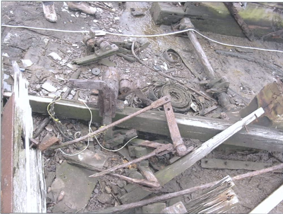
Figure 4-68. Pile of miscellaneous debris and machinery parts noted on the deck of V36.
