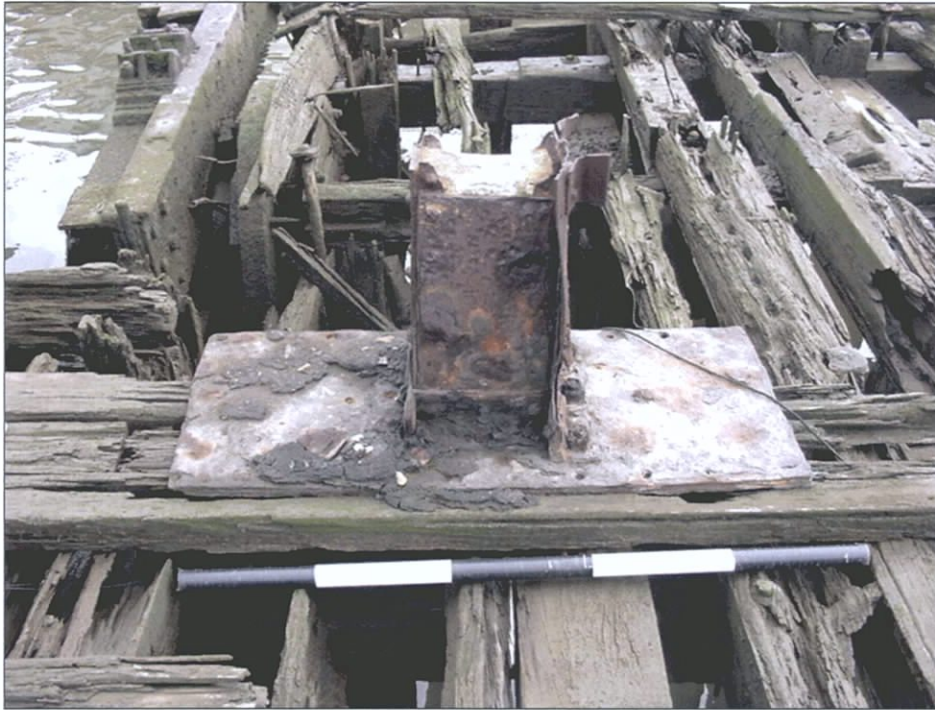
Figure 4-48. Starboard H-frame mount. View to the south (forward).
