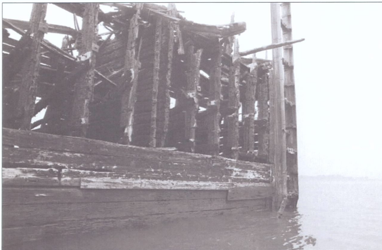
Figure 5-104. Outer wall of starboard wing. View to the northwest. Note locations of wing trusses and bulkhead.
