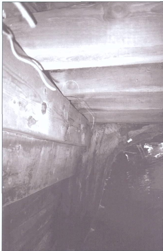
Figure 7-64. Detail of deck beams resting on the clam and shelf along with a hanging knee. Looking aft (north).
