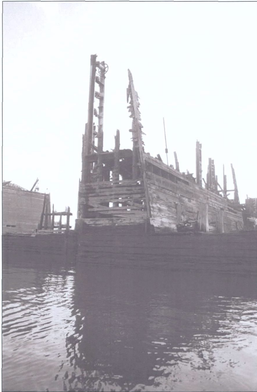
Figure 5-164. Starboard wing showing spuds. The rightmost spud belongs to another dock. View to the northeast (starboard forward).
