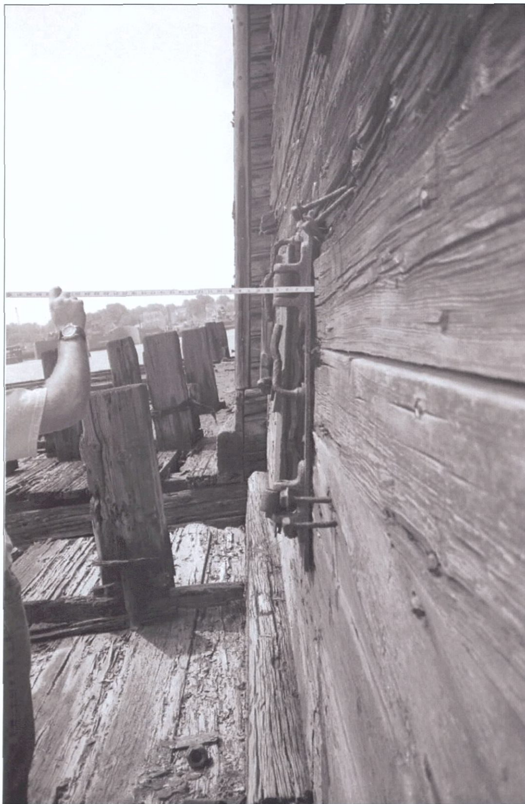
Figure 5-142. Aft small hatch, port wing side detail. View to the south (aft).
