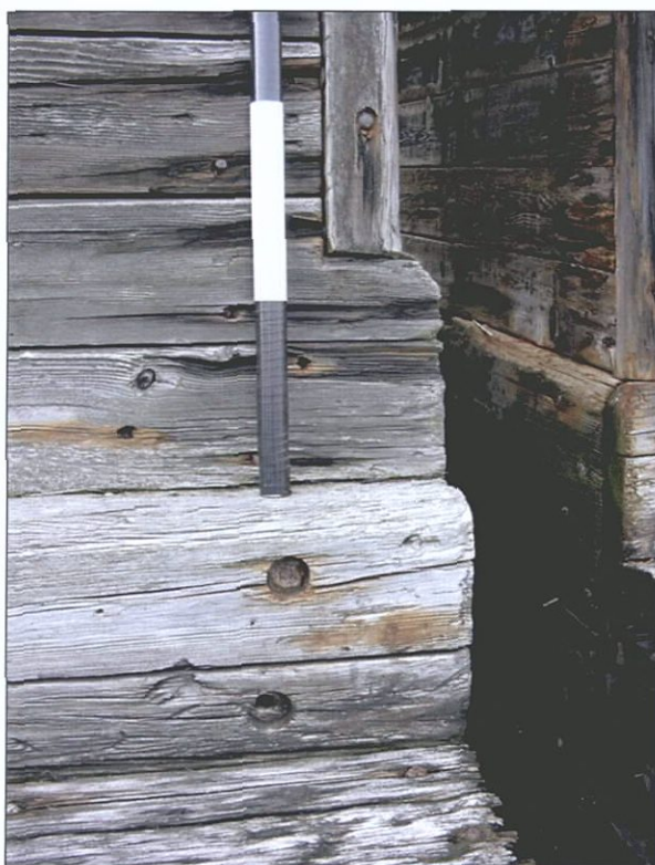
Figure 5-130. Close-up of forward inner corner of port wing, V1. View to the west (port).
