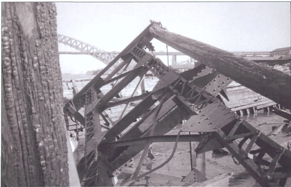
Figure 4-63. Close-up of collapsed A-frame. View to the southeast (port).
