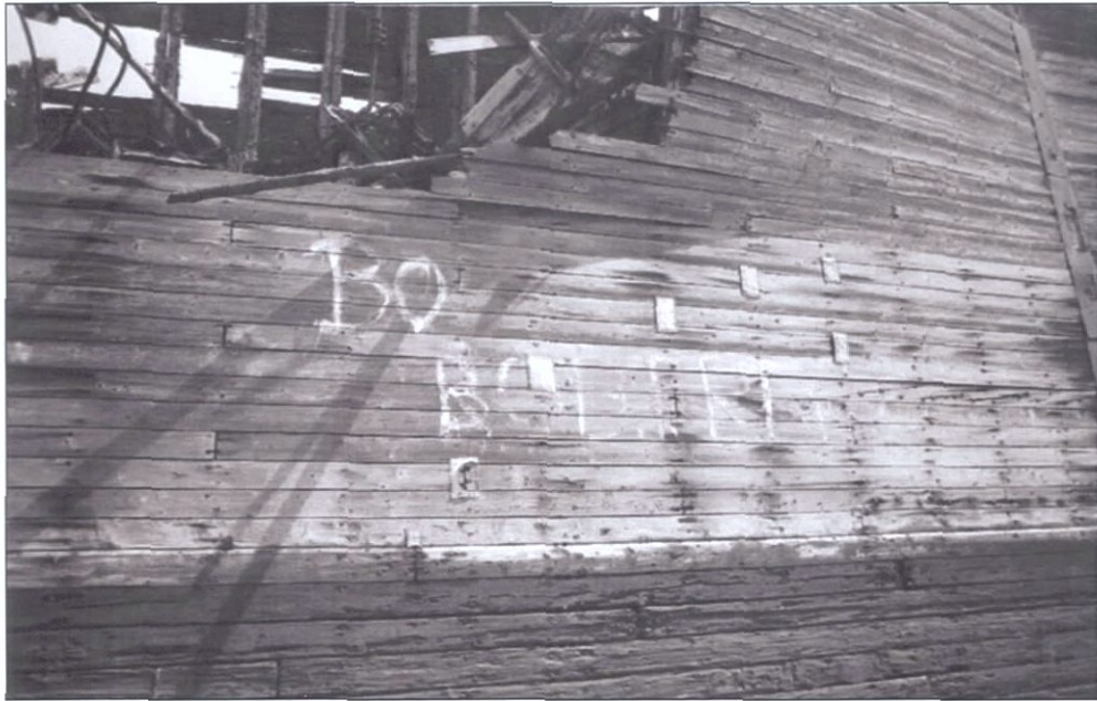
Figure 5-127. Detail of port wing, aft corner. Note change in plank sided dimension similar to the inner wing wall. View to the east (starboard).
