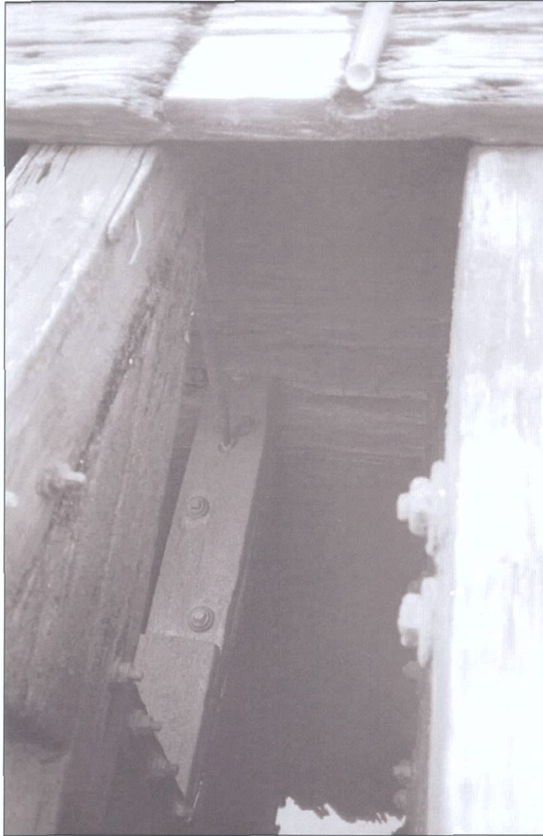
Figure 5-65. Third longitudinal bulkhead (L4) showing Truss 1 and Truss 6. View from port toward centerline of vessel.
