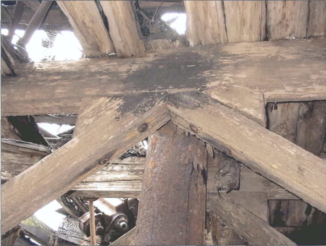
Figure 5-116. Second wing deck beam. Note chocks and fasteners. Starboard wing. View to the north (forward).
