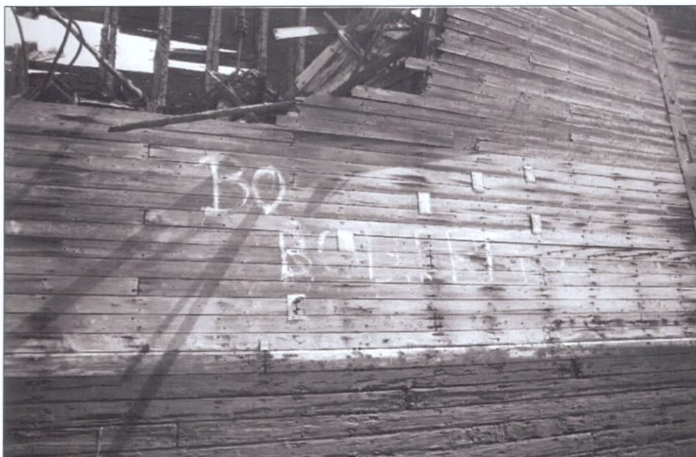
Figure 5-170. Port wing showing tin patches covering plank joints. View to the southeast (starboard).
