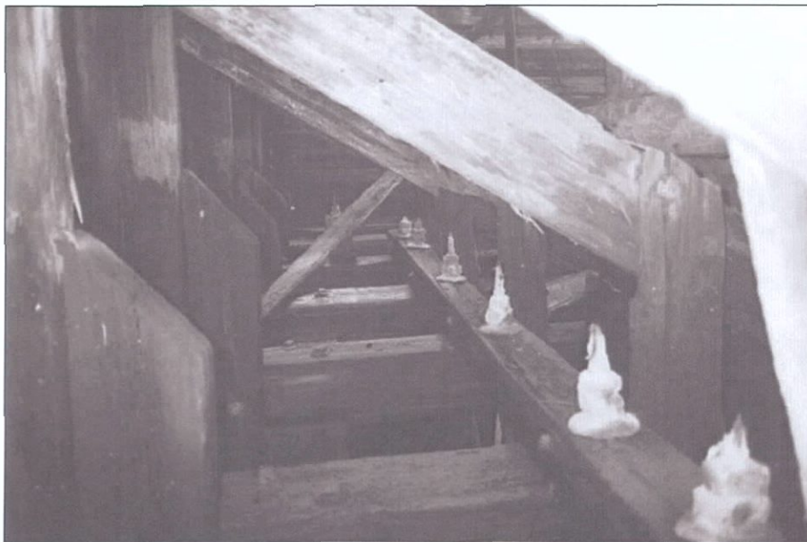
Figure 5-159. Longitudinal stringer providing stability to vertical supports, which, bolted to the wing truss, support the weight of the vertical discharge pipe. Note vertical tie rods, which fasten the stringer to the pontoon framing. Port wing, view to the north (fore).
