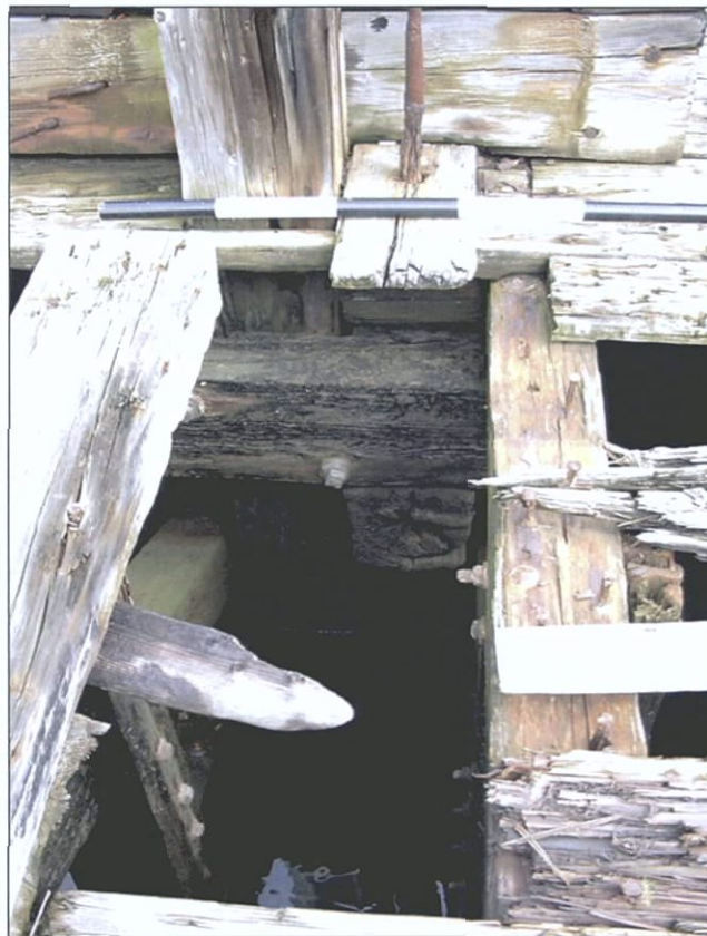
Figure 5-74. Detail of structure of aft starboard bitt showing stringers and, directly below, transverse bracing. View to the east (starboard).
