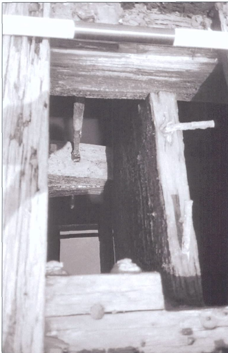
Figure 5-49. Top of longitudinal bulkhead showing exposed fasteners.
