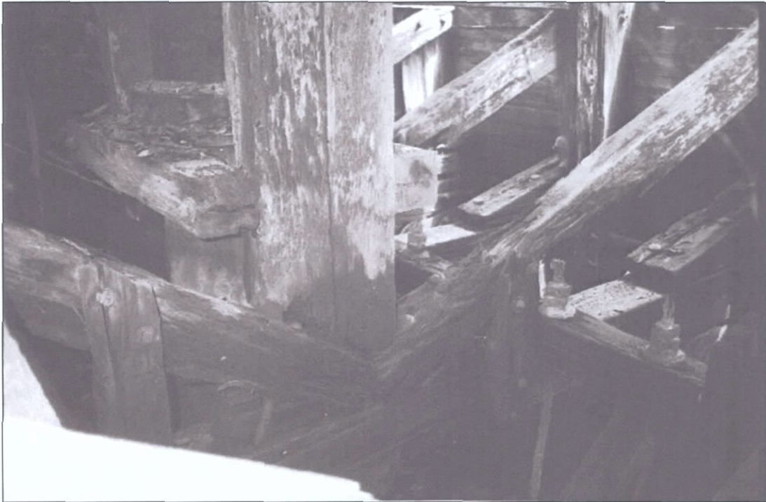
Figure 5-160. Longitudinal stringers spanning one pair of wing frames provide platform to support the vertical discharge pipe. Extra vertical timbers distribute weight of pipe to other horizontal timbers in the wing truss system. Longer longitudinal stringers like that shown in Figure 5-156 provide lateral support to vertical timbers. Port wing, view to the north (forward).
