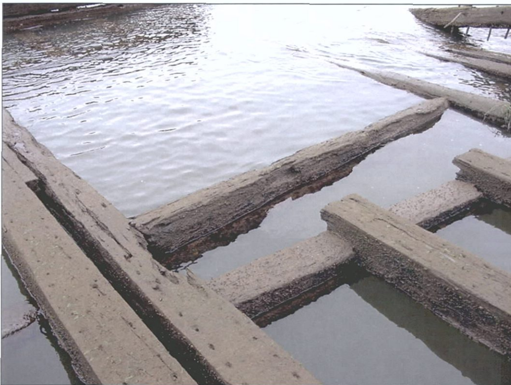
Figure 6-91. Detail of foreword cargo hatch with separated carling. Note notching of partial deck beams into carling and over rider carling. View to the northwest.
