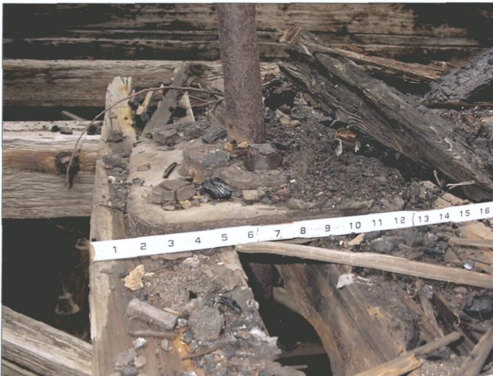
Figure 5-163. Close-up of support structure for gate valve drive shaft.
