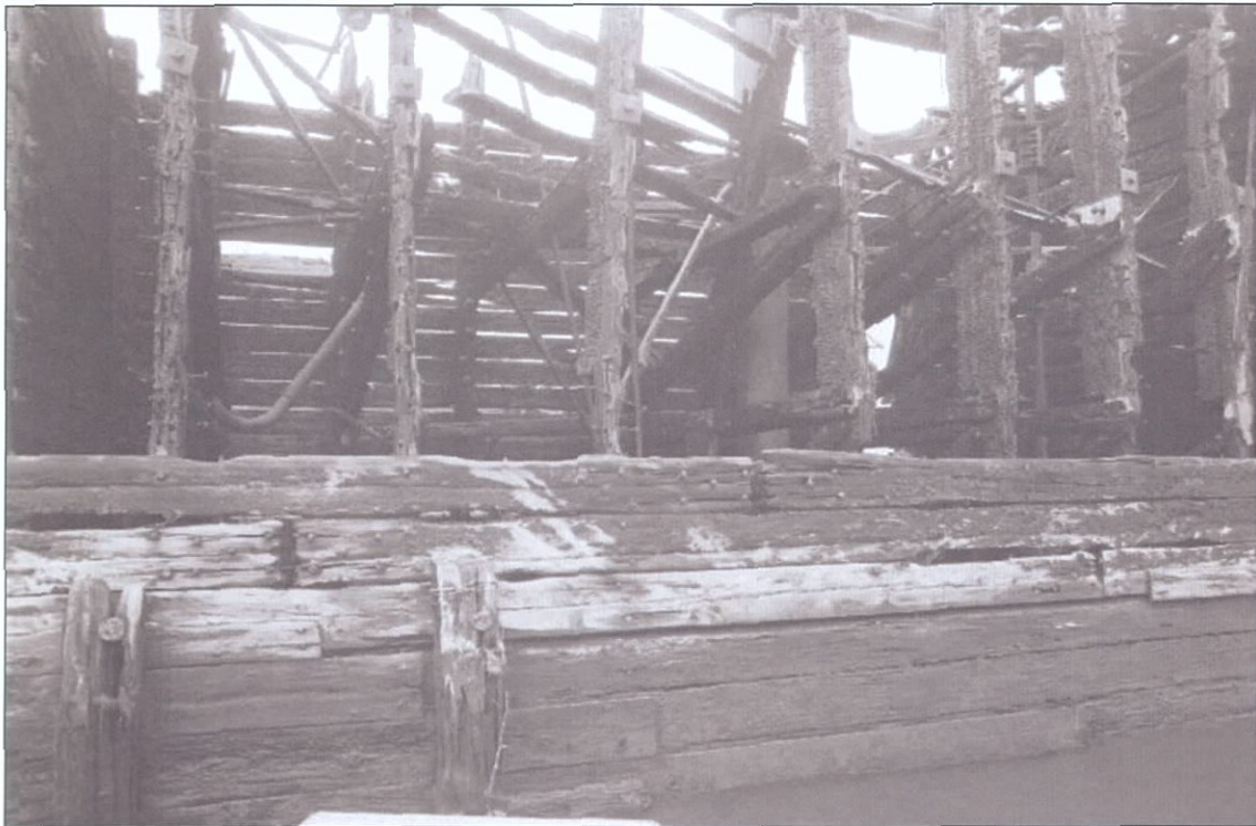
Figure 5-148. Remnants of starboard wing, showing pump, valve, and floodgate actuator rods.
