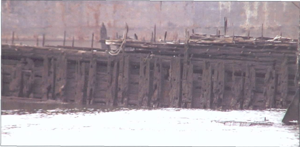
Figure 6-105. Port side, amidships, showing arrangement of futtocks and frames. View to the southwest.
