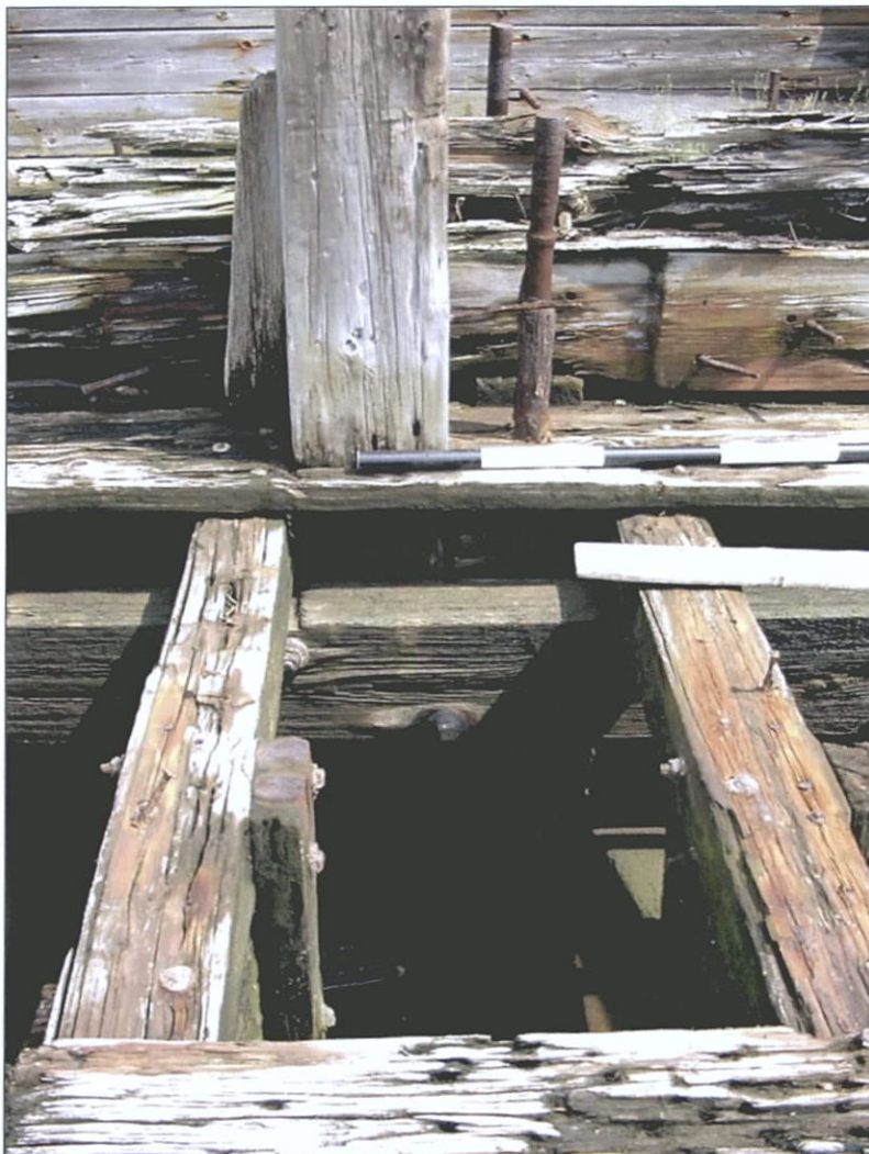
Figure 5-72. Starboard aft bitt structure showing vertical bitt and longitudinal stringer. View to the east (starboard).
