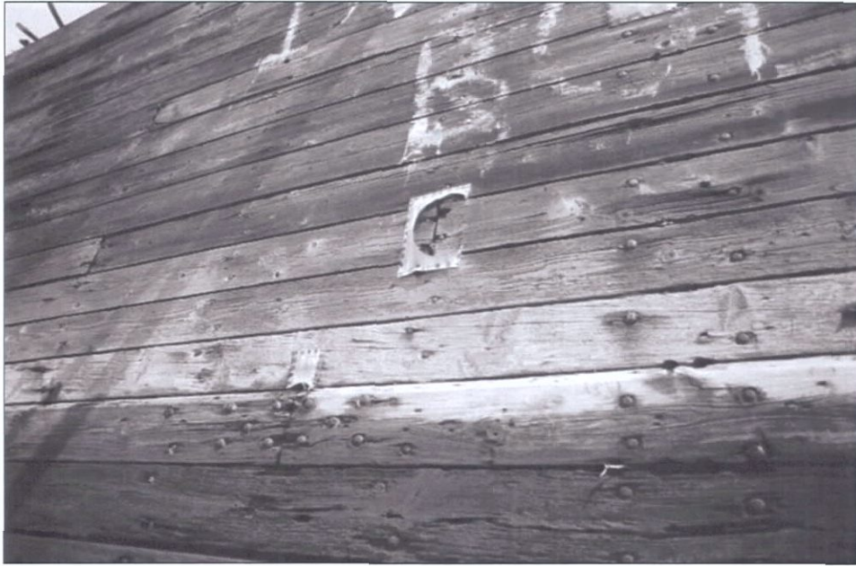
Figure 5-177. Port wing outer surface, showing carriage bolts at bulkhead (right) and the inter-frame plank joint (reinforced by a chock on the interior of the vessel). View to the northeast (starboard forward).
