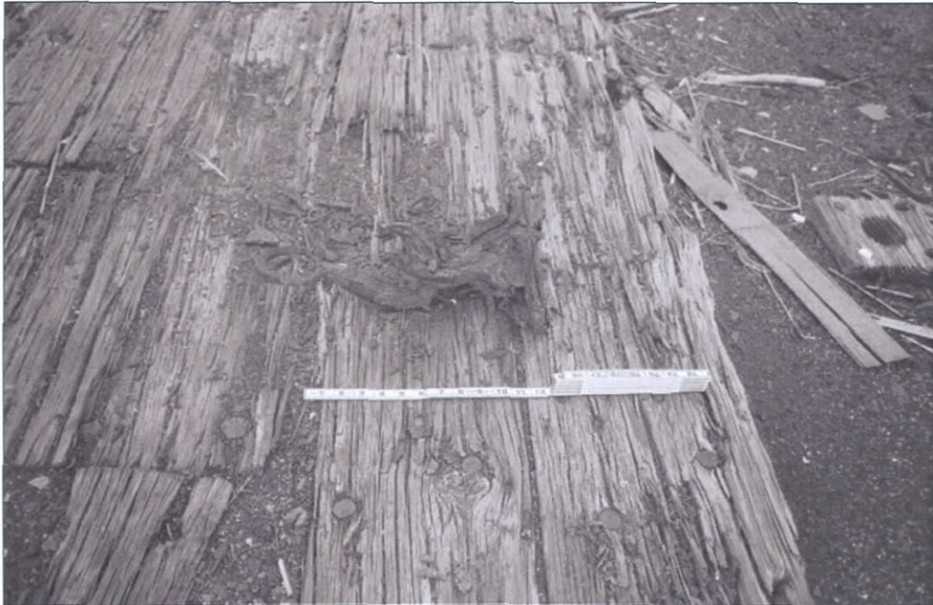
Figure 5-89. Loose hook and eye, highly deteriorated and concreted.
