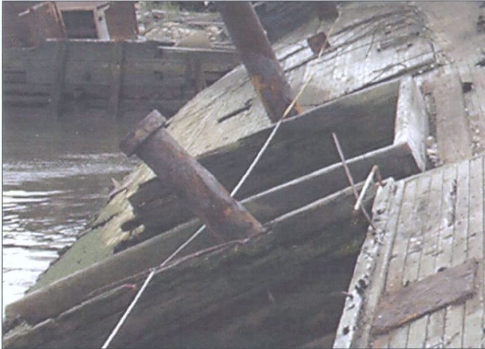
Figure 7-92. Fish Hawk from port side looking forward (south). Note remaining vent stack and main mast.
