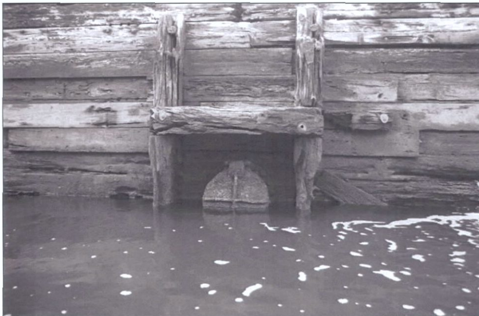
Figure 5-150. Pump outlet on outer hull.
