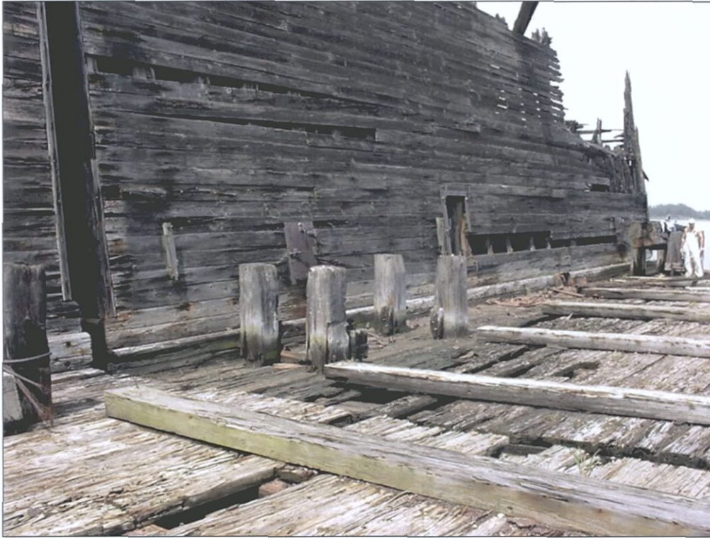
Figure 5-80. View from aft looking toward port bow, showing placement of bilge block stringers and port aft bitt.
