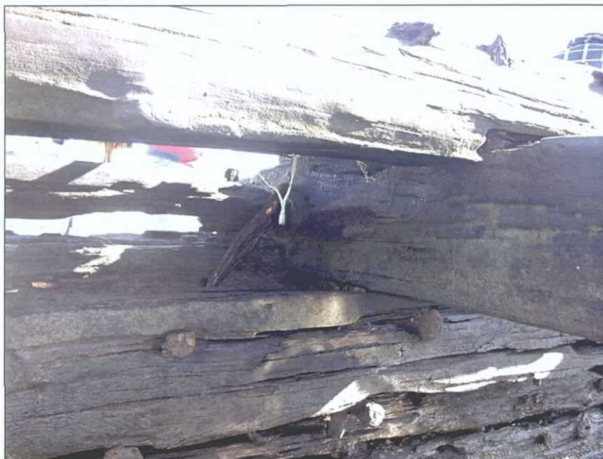
Figure 6-95. Port side view looking port (east) showing deck beam, waterway, and clamp.
