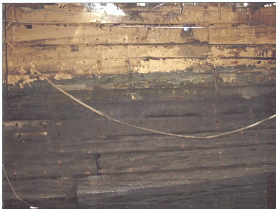
Figure 6-67. Close-up of ceiling planking in crew compartment, looking starboard (west). Note tan paint.
