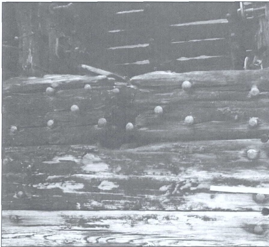
Figure 5-33. Close-up of butt joint. Note array of fasteners joining chock on inboard side of joint.
