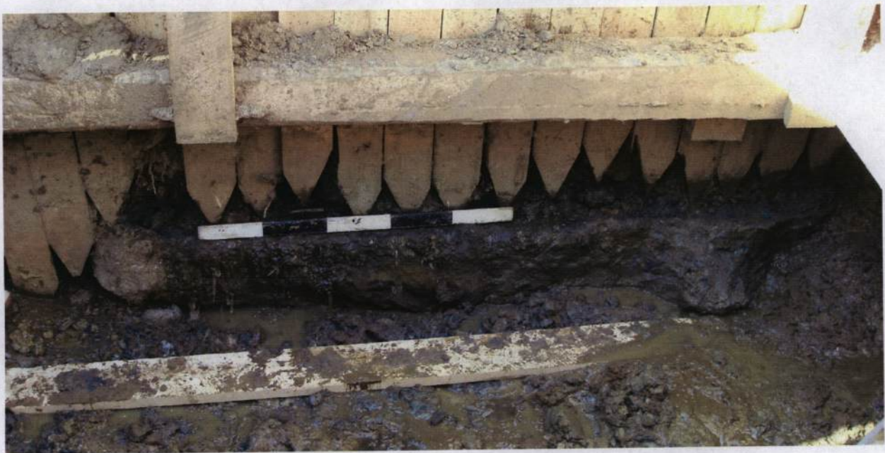
Figure 10: West view of the concrete platform exposed in the fuel tank excavation pit at about 7.5 feet below the surface. A close inspection of the feature revealed modern rebar and threaded rods that may have been used to secure a former tank since removed. Scale bar 5 feet.
