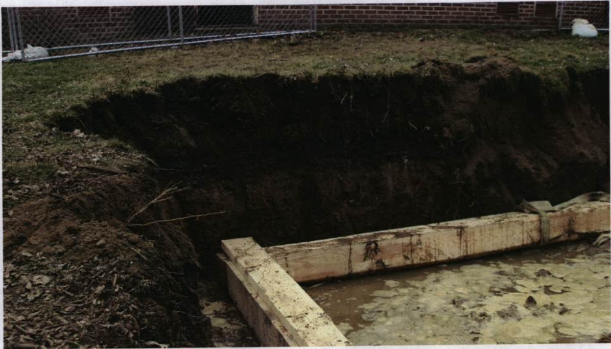
Figure 9: West view of the excavation for the underground fuel tank adjacent to building #430 (in background). Note the flooding within the cribbing. The profile of the west wall of the excavation pit shows extensive fill layers associated with prior construction activity.
