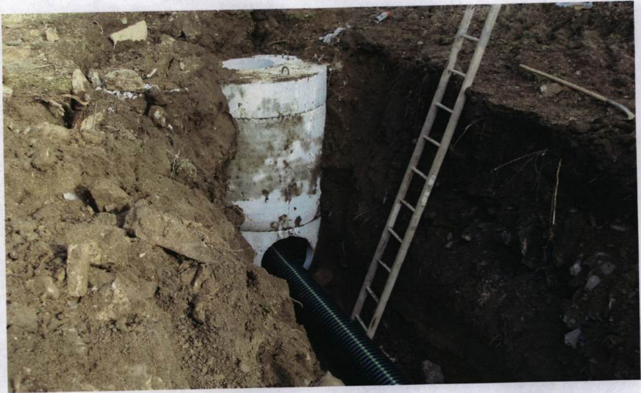
Figure 13: Northeast view of the northeast bottle dump feature, visible in the eastern wall of the trench several feet below the surface. Overall depth of the trench is approximately 9 feet, excavated for the installation of a drainage system.
