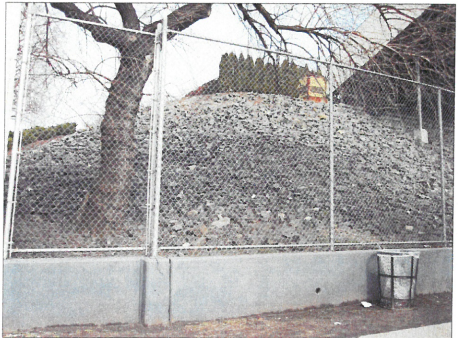
Looking west from West 218th Street at rip-rap covered hill between maintenance building and soccer field bleachers (at right)
