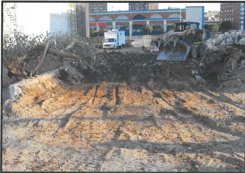
Photograph 3.2 Block 1127, Lots 48 and 50 post-demolition and removal of up to 24 inches of rubble fill.
