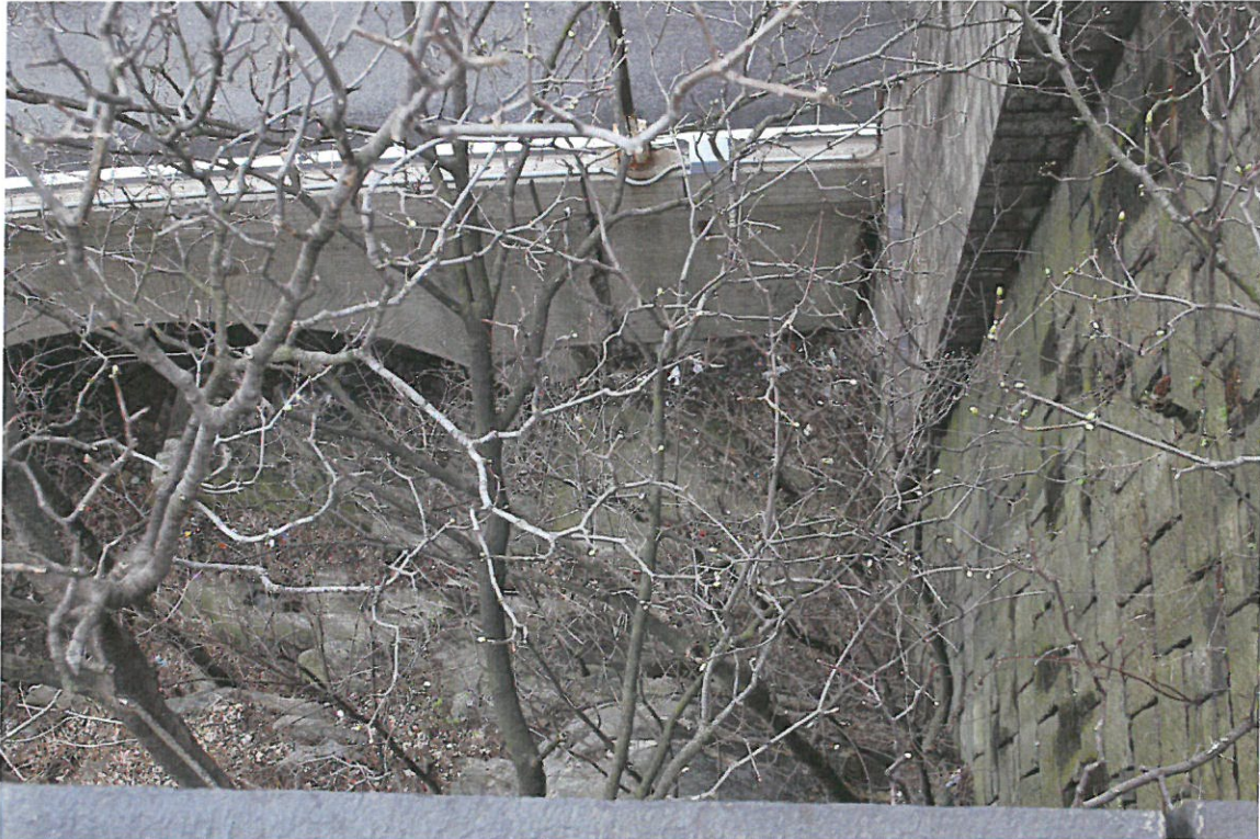
Photograph 4: Manhattan terminus showing detail of an arch supporting the Harlem River Drive. View looking east from bridge approach on north side of APE.
