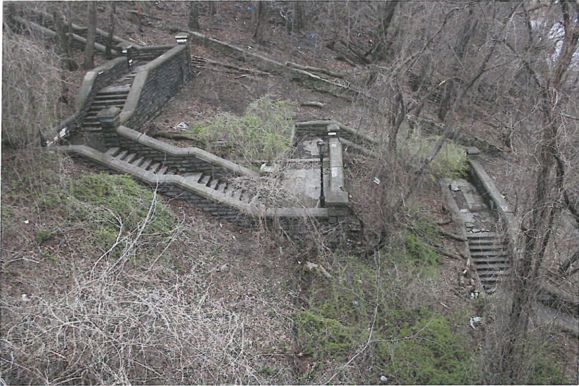
Photograph 11: Detail of ashlar stairway south of Bronx touchdown. Note stone wall marking southern edge of property. View looking south from bridge.
