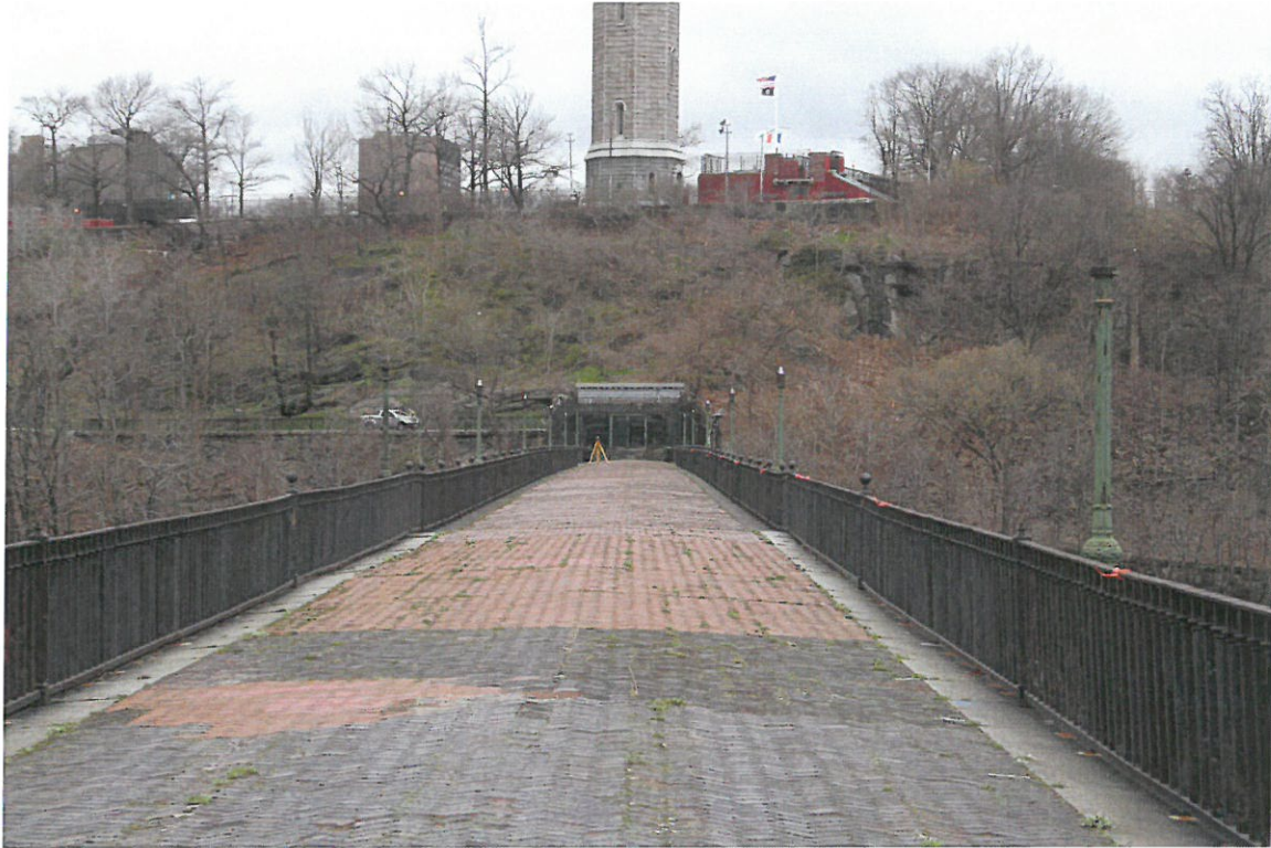
Photograph 8: High Bridge and Manhattan terminus showing the area east of the gate house including a steep incline with exposed bedrock that rises up to Highbridge Tower and a recreation area with a pool (formerly a reservoir for the OCA). View looking west from bridge.
