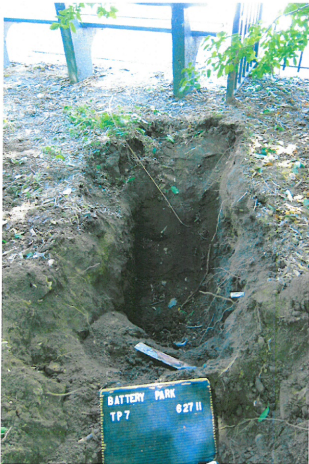
Photo 9. Test Pit 7 (TP7) looking north with the Battery Place sidewalk in the background. (Geismar 6-27-11)
