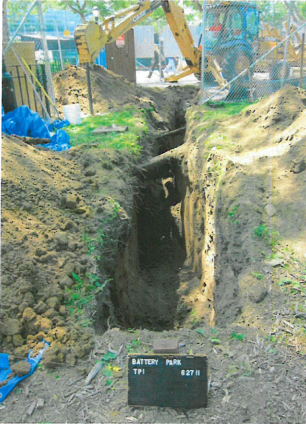
Photo 1. Test Pit I (TP1) looking south. The deepest of the planned test pits at 6.2 feet BGS, it comprised a mixed fill and was crossed by several utility pipes. (Geismar 6-27-11)
