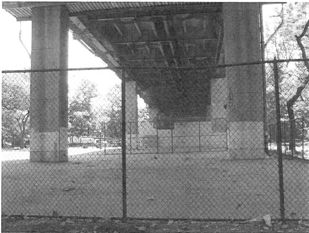
Photo 4. View southeast toward existing Francis Lewis Park ballcourts under the bridge approach.
