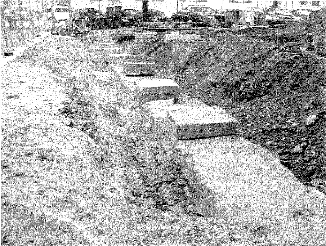
Figure 1A: Wall A, the foundation wall in the southeast corner of the site, looking south towards Leonard Street.
