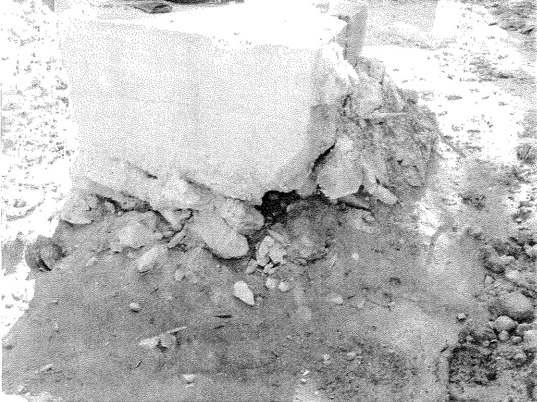
Figure 2A: A concrete block with iron rebar on top of Wall A.
