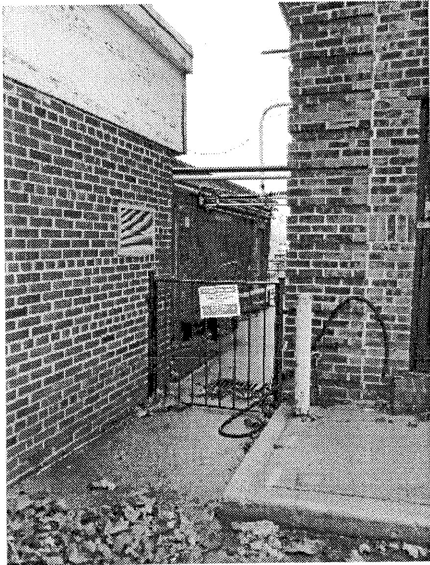
Photo 1 Space between Building #s 146 (left) and 148 (right) showing overhead utility lines, facing northeast (November 22, 2011).
