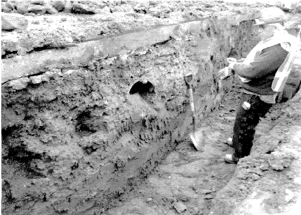
Photo 1 Trench from CB 1.04 to MH 1.14 showing coal ash deposit around defunct pipe, facing northeast (February 17, 2012).
