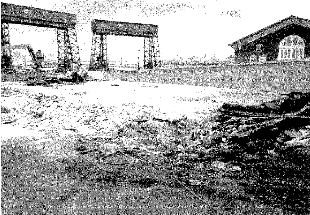
Photo 6 Concrete slab foundation of Building #148 after the superstructure was demolished, facing northeast (May 10, 2012).
