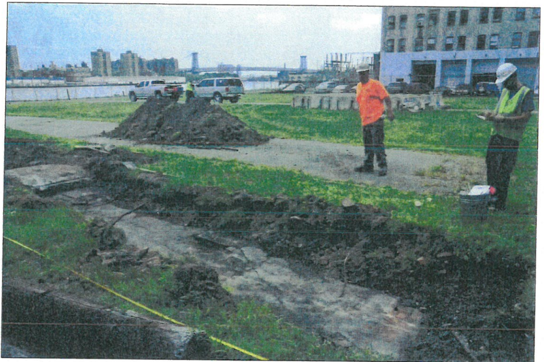
Facing northeast from southwest corner of project area showing location of Trench 1. 1 Trenches 2 and 3 are located behind building to the far right
