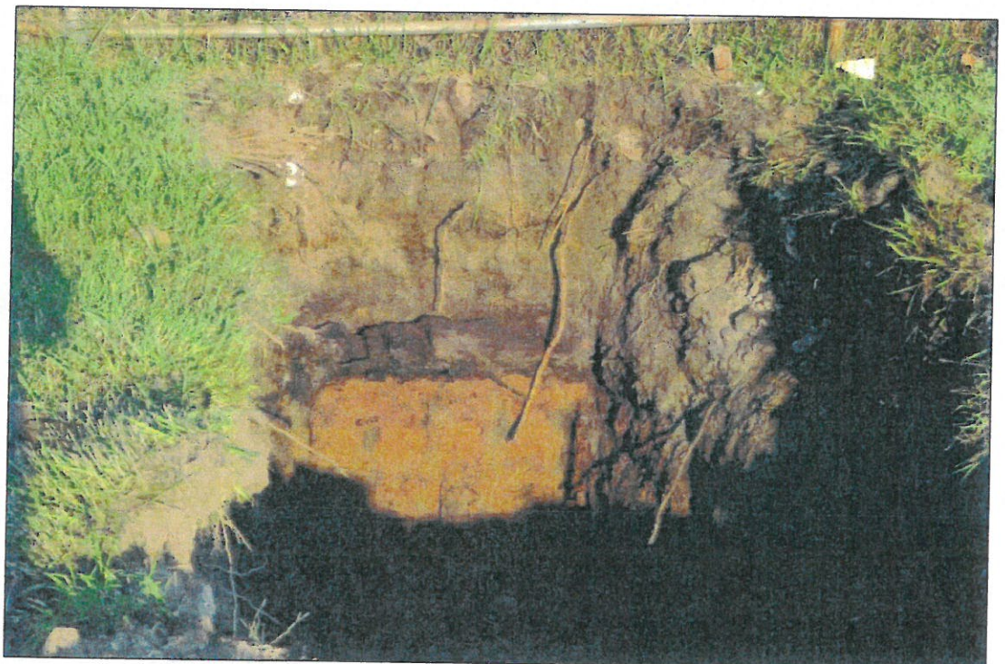
Facing west toward the west wall of Trench 3 showing the soil layers encountered in Trench 4. A concrete pad and compacted soils were encountered in the upper three feet of the trench, 13 followed by loose sands. The dark horizontal object is a piece of wood and tar
