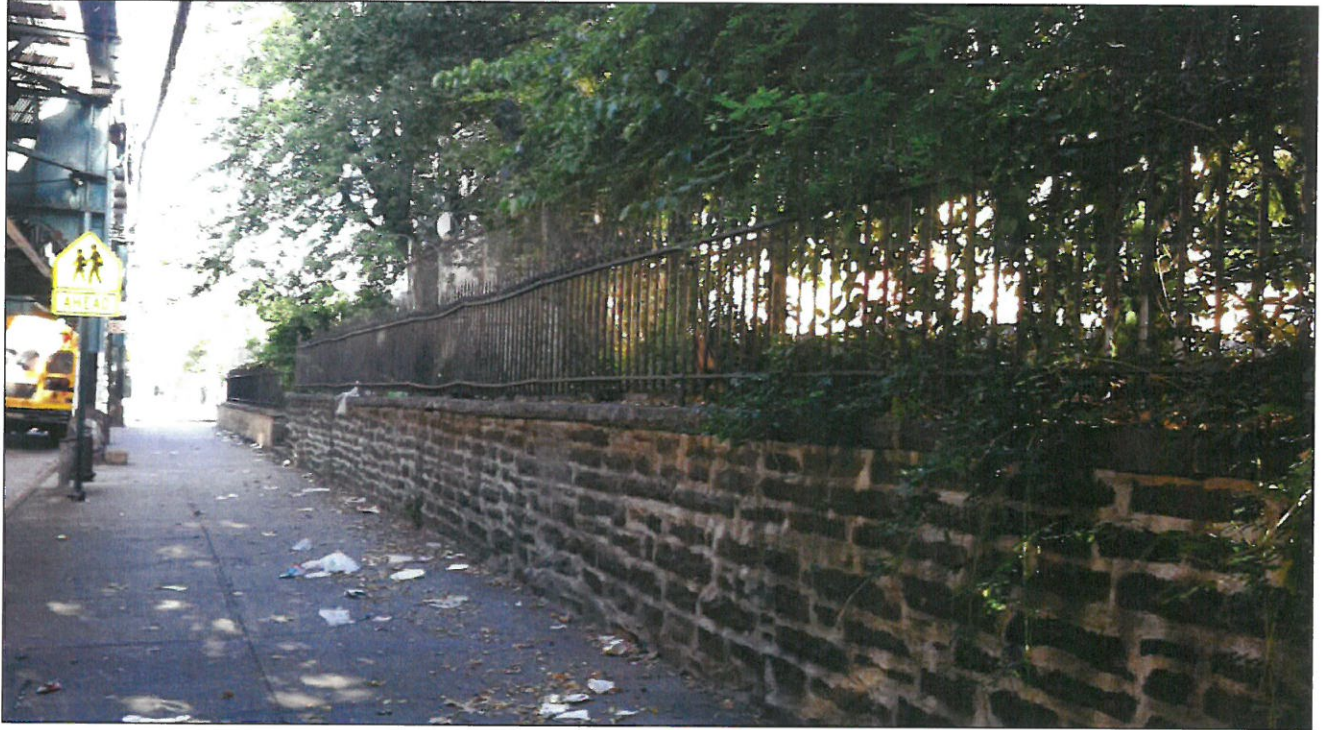
The stone retaining wall that lines the project site along Broadway. The elevation of the project site is several feet higher than the sidewalk below
