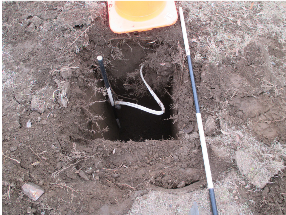
Photo 25 Hole left after removal of light post footing across from Soissons Landing on National Park Service property, facing north (Image 4067: March 25, 2014).
