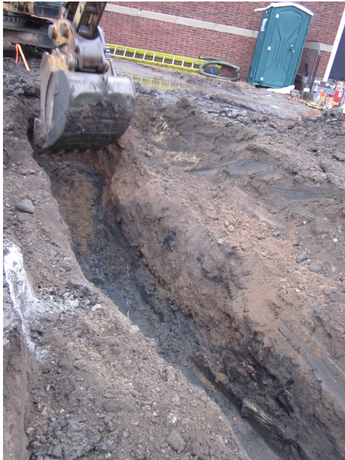
Photo 12 Part of a horizontal wooden member initially thought to be part of a landfill-retaining structure seen at the bottom of the photograph in the base of excavation, facing northwest (Image 1886: January 16, 2013).
