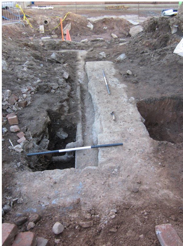
Photo 6 Feature 2 after the completion of excavation units showing the exposed foundation, facing north (Image 1764: January 7, 2013).
