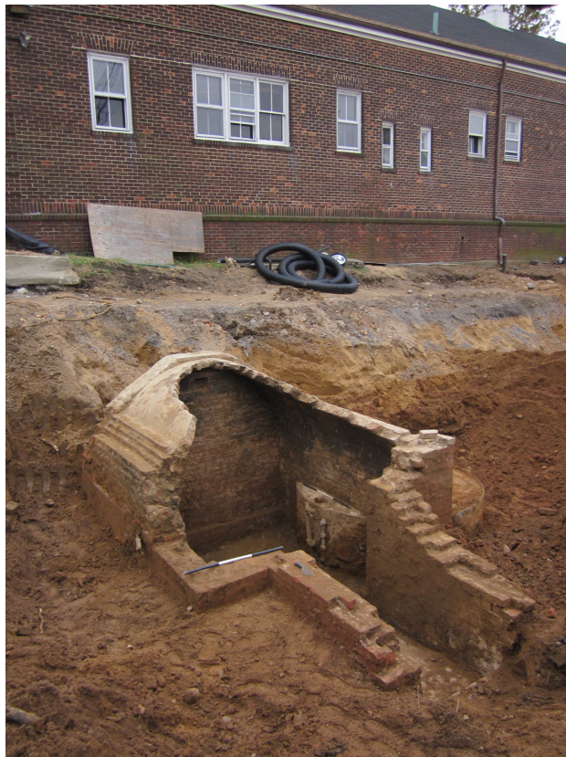
Photo 4 Feature 1 after removal of the interior fill showing the intact fuel tank partially inside and partially outside of the brick structure, facing southwest (Image 1490: October 25, 2012).
