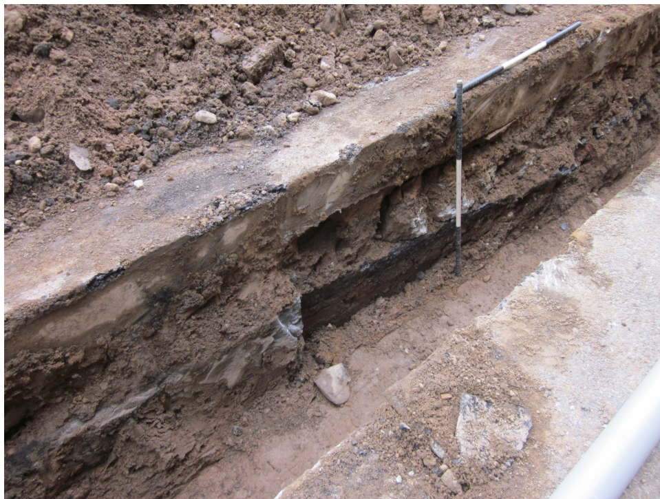
Photo 24 Former curb exposed toward the bottom of the electrical line trench excavated in Andes Road between Building #s 111 - 112, facing west (Image 2210: February 28, 2013).
