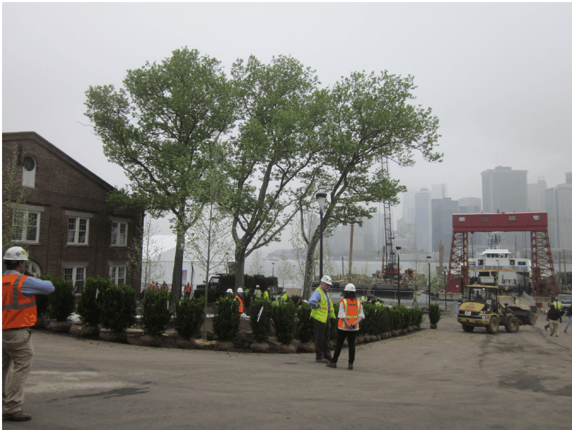
Finishing touches to Soissons Landing in preparation for opening day, facing northwest (May 22, 2013)
