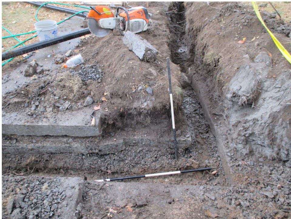
Photo 26 Former concrete surface exposed in the irrigation line excavation in Tile 13 - Parade Ground Zone, facing north (Image 3682: November 7, 2013).
