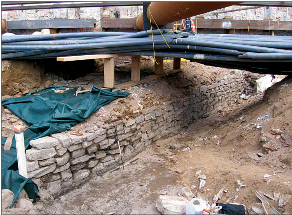
Figure 21. When the southern face of Wall 4 was completely exposed beneath numerous utilities, it was nearly 40 feet long.
