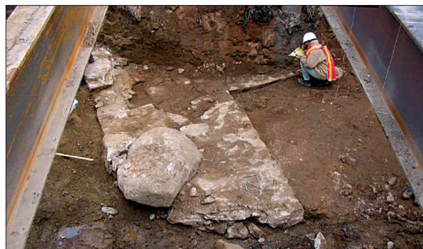
Figure 4. Wall 1 was the first section of Battery Wall discovered during the South Ferry Terminal construction project. Note the large boulder incorporated into the Wall.
