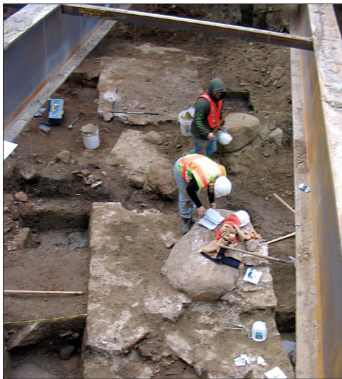
Figure 6. Archaeologists from Dewberry-Goodkind, Inc. were assisted by those from URS Corporation to complete Wall 1 excavations as quickly and efficiently as possible so as not to delay construction of the new South Ferry station.
