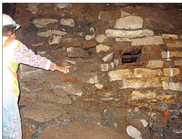
Figure 46. Stone retaining wall at the head of the Slip. Note the drain in the center of the wall which would have funneled water from the street into the Slip.
