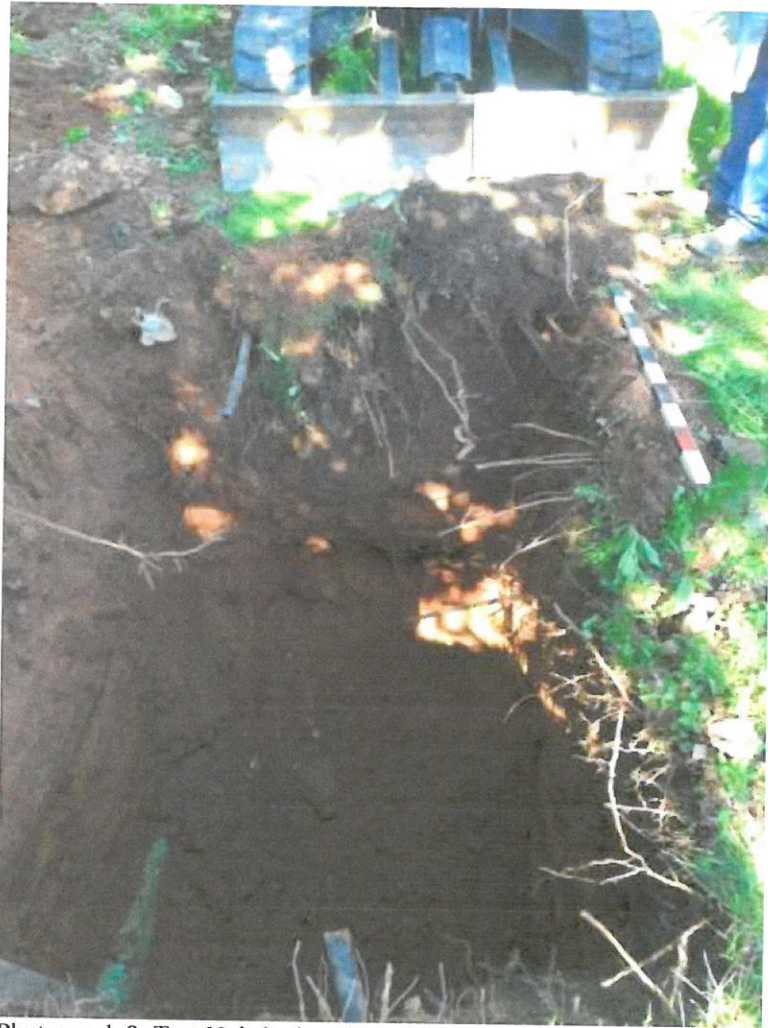
Photograph 8: Test Unit 3, showing Verizon conduit (green casing) at base of pit adjacent to sterile subsoil. View looking east.
