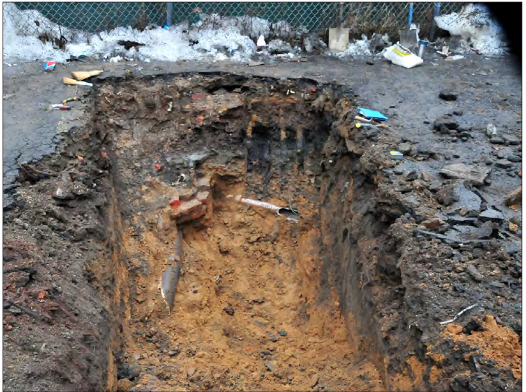
View south of the brick and terra cotta pipe drainage feature observed in Trench 16 8
