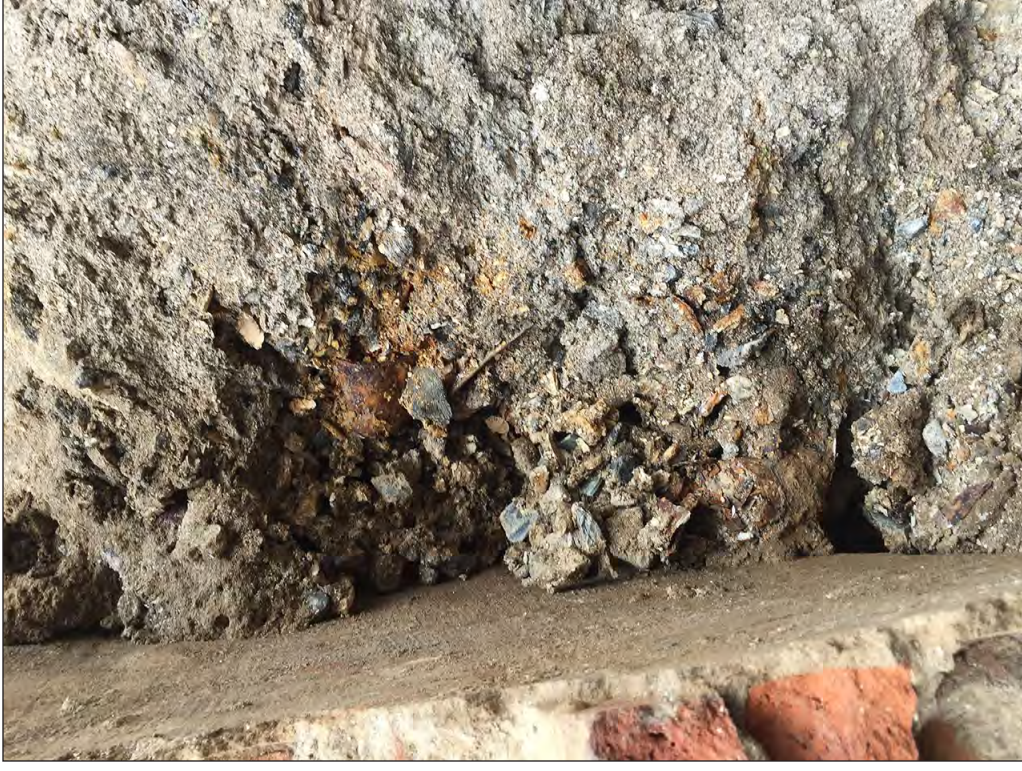
Close-up of the loose gray and brown ash with rusted metal making up the fill within the East Feature on historic Lot 44 18
