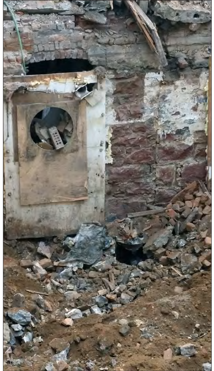
Same, showing the view from the west. The circular iron void is noticeable to the right of the plywood covering the arched doorway
