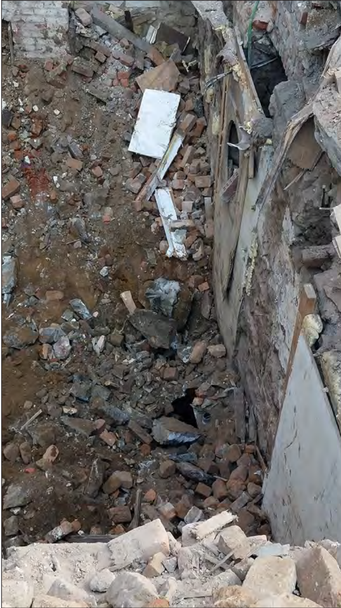
Looking north at the stone rubble and iron pipe or tank (the circular void) at the base of the arched doorway in the east wall of the building formerly at 233 Duffield Street
