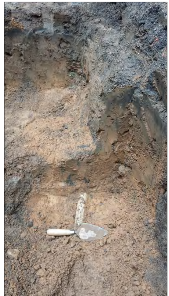
Lead pipe within apparent subsoil within Trench 6 in the rear yard of Lot 12 4
