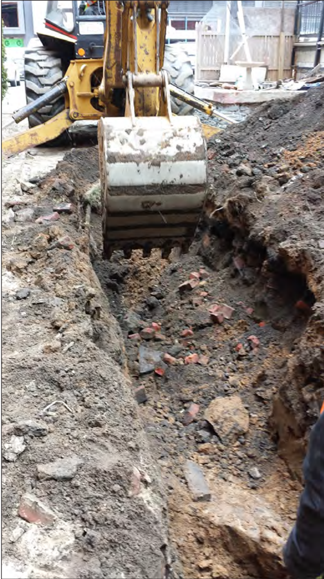
Looking east as brick rubble is excavated from the center of the rear yard of Lot 12 within Trench 7 5
