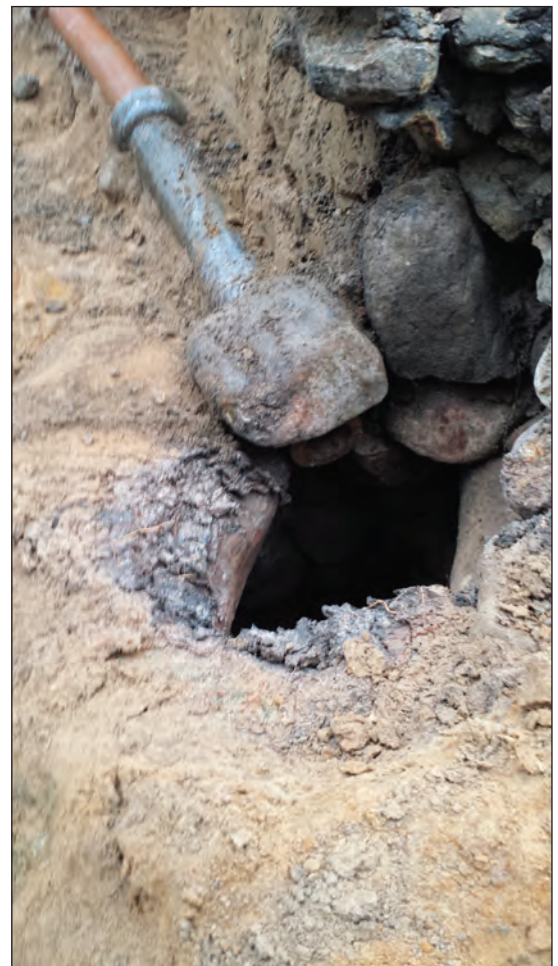
Drainage improvements made to connect terra cotta pipes to the stone well 24
