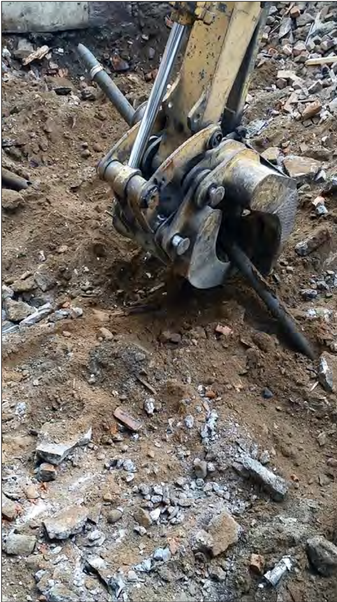
Large pipe being removed from beneath the slab during the demolition of the sub-cellar floor A
