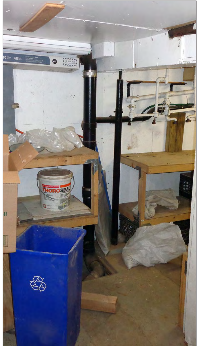
The sub-cellar before demolition; showing an extension of the same pipe extending vertically down the west wall of the building from the basement and then extending beneath the slab via an unpaved section of the floor B
