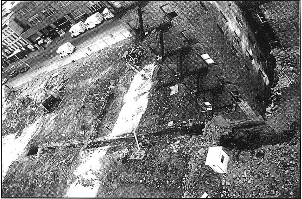
Plate 2. Trench 1 parallel to the rear wall of the standing structure on Lot 29. Facing south.
