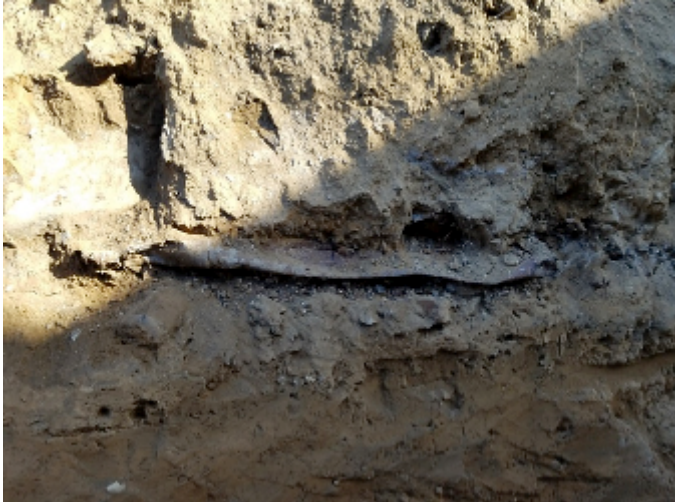
Photograph 5. View of a section of the east wall of Trench 3 and the section of utility pipe after exposure.
