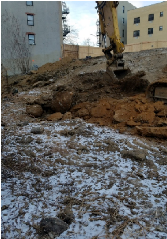
Photograph 2. View of Trench 1 during excavation at the east end of the trench. Note the extremely rocky soil.
