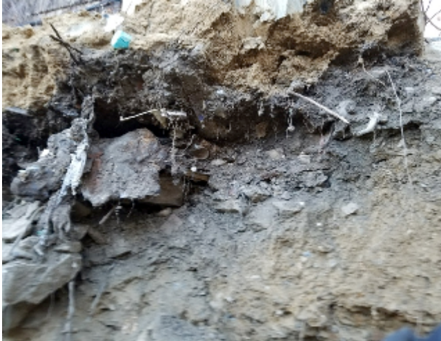
Photograph 3. View of a section of the west wall of Trench 2 during excavation. Note the distinct fill soil stratigraphy.
