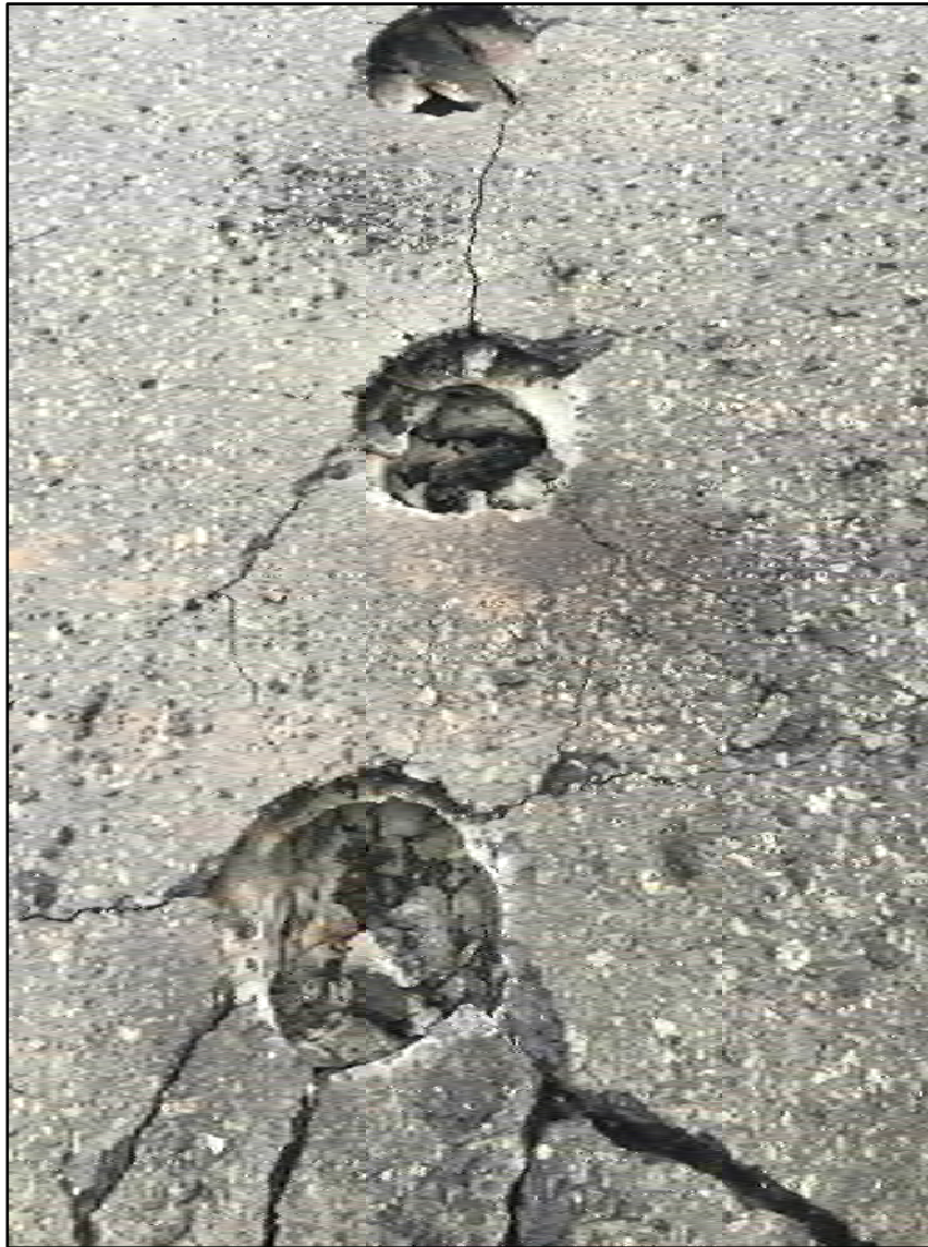
Photograph 4.6 Postholes from southern half of construction fence line, underlying concrete encountered, view to the north.
