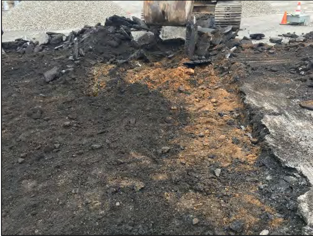
Photograph 4.9 Lighter soil exposed in the northeast corner of the western entranceway, at the time thought to be potentially natural, view to the north.
