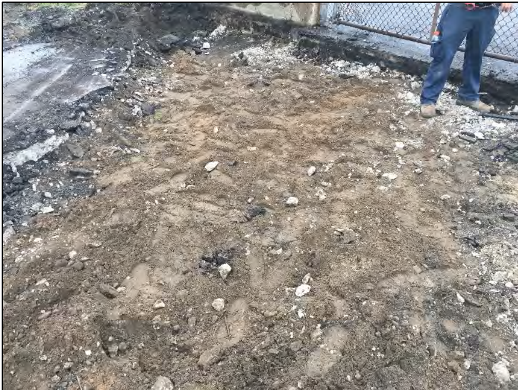
Photograph 4.3 Eastern construction entranceway fill soils underlying removed concrete slab, view to the southeast.
