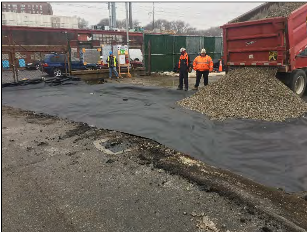
Photograph 4.4 Eastern construction entranceway covered in filter fabric and gravel, view to the south.
