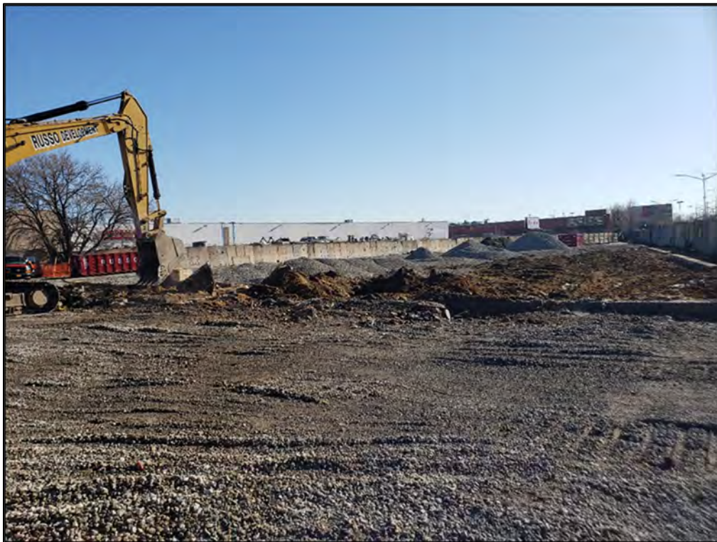
Photograph 4.19 Final grading and graveling of warehouse building footprint, view to the east.
