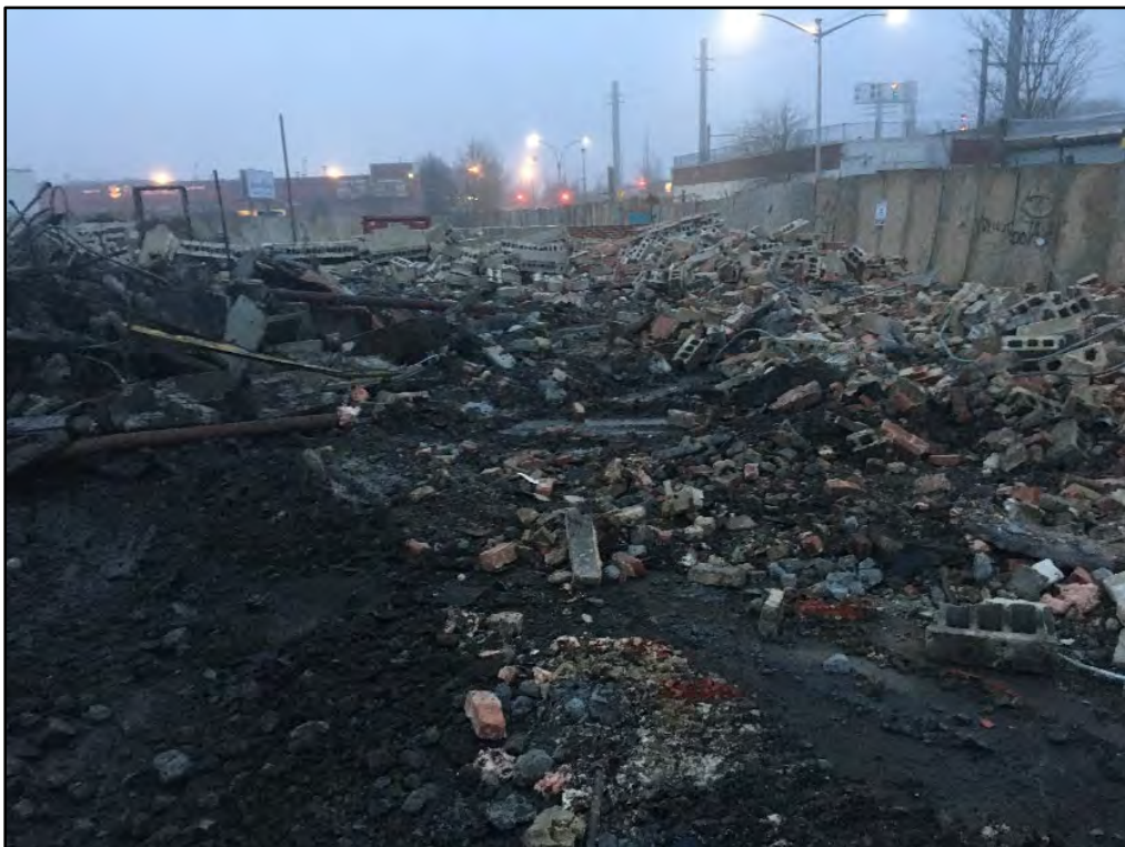
Photograph 4.12 Rubble pile from the aboveground demolition of the warehouse building, view to the northeast.
