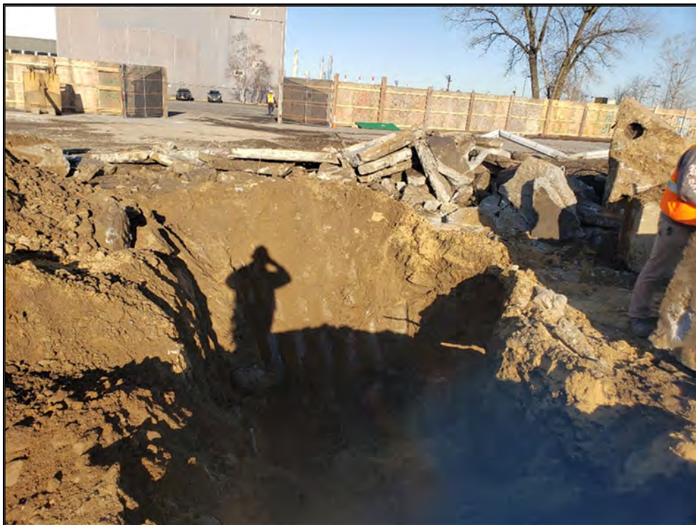
Photograph 4.17 Base of EX2 at approximately 7 feet below grade with fill soils still observed, view to the west.
