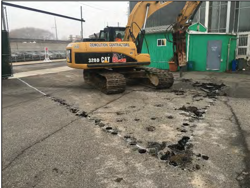
Photograph 4.7 Western construction entranceway outline being cut out in asphalt, view to the southwest. Note the NYCDEP trailer and church in the background.
