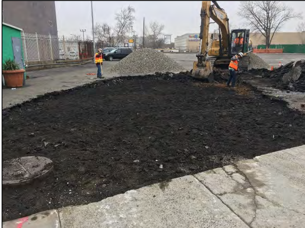
Photograph 4.8 Western construction entranceway with fill soils underneath, view to the north. Note the lighter soil near the excavator bucket, at the time thought to be potentially natural.
