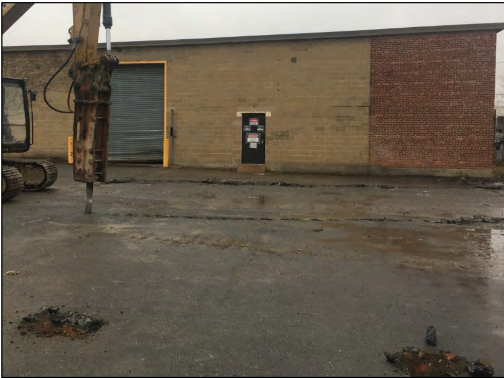
Photograph 4.1 Eastern construction entranceway outline being cut out in asphalt, view to the northeast. Not the standing warehouse building in the background, and two postholes for the planned construction fence line in the foreground.
