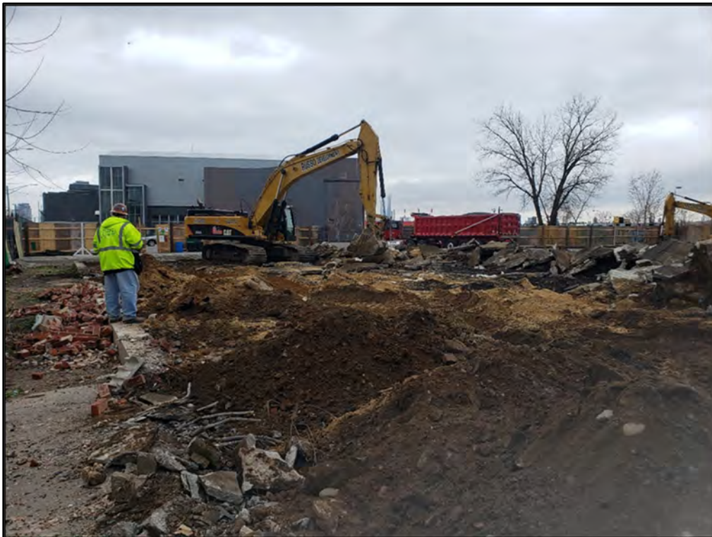
Photograph 4.14 Overview of support pillar removal beneath warehouse slab foundation, view to the west.
