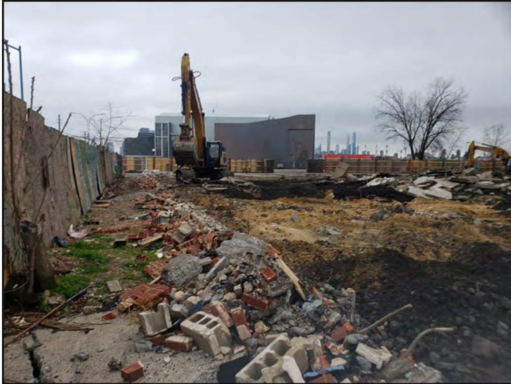
Photograph 4.13 Overview of the slab foundation removal for the warehouse building, view to the west. Note the bright yellow leveling sand.
