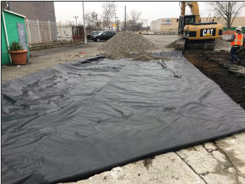
Photograph 4.10 Western entranceway covered with filter fabric prior to gravel spreading, view to the north.
