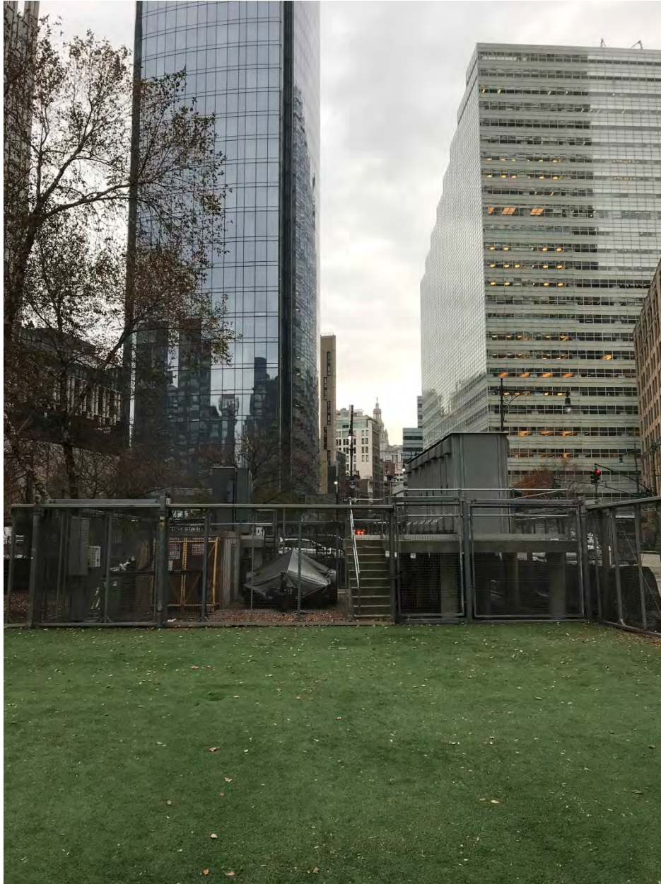
Photograph 6: Close up of utility boxes at the southeastern corner of the Battery Park City Ballfields, facing east from just north of Murray Street.
