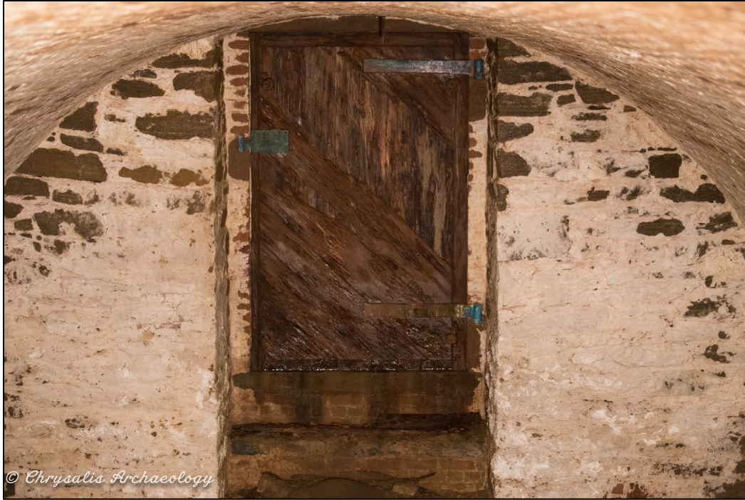
Image 14: Detail of door of Burial Vault 2 showing water seepage, facing west.
