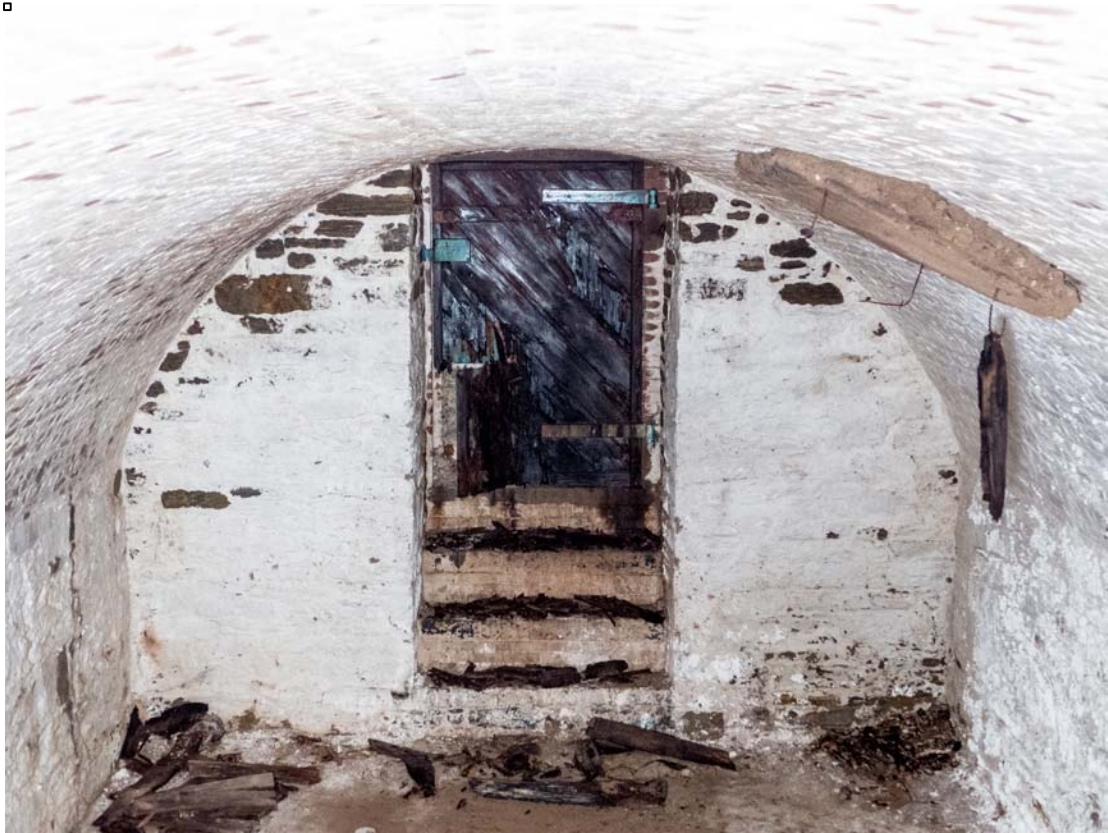
Image 01: Burial Vault 01 showing vault construction and patch on the roof of the vault.
