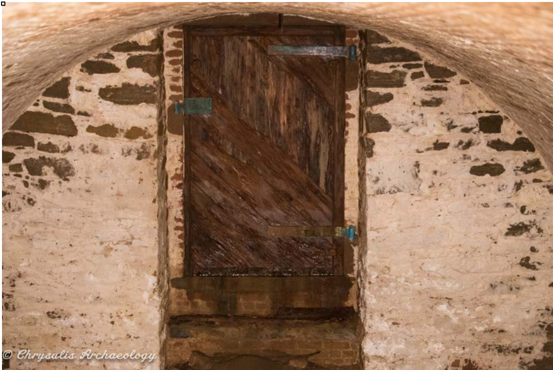
Image 04: Door of Burial Vault 02 showing water seepage.
