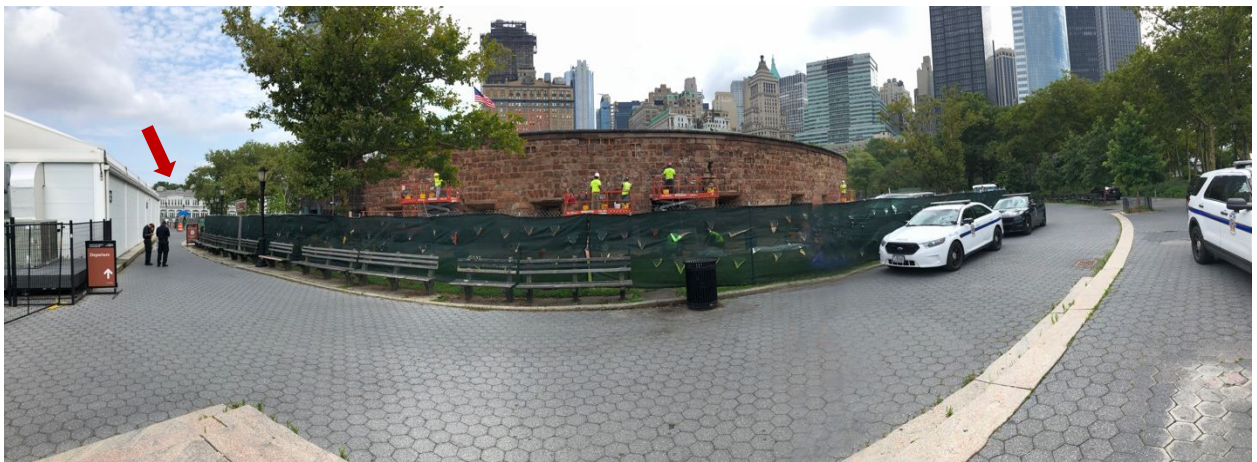
Photo 2. Castle Clinton is seen undergoing repair of its exterior wall in this panoramic view taken from the walkway (left) in the APE. Pier A (arrow) is in the far left background. (Photo: J. Geismar 7/28/21)
