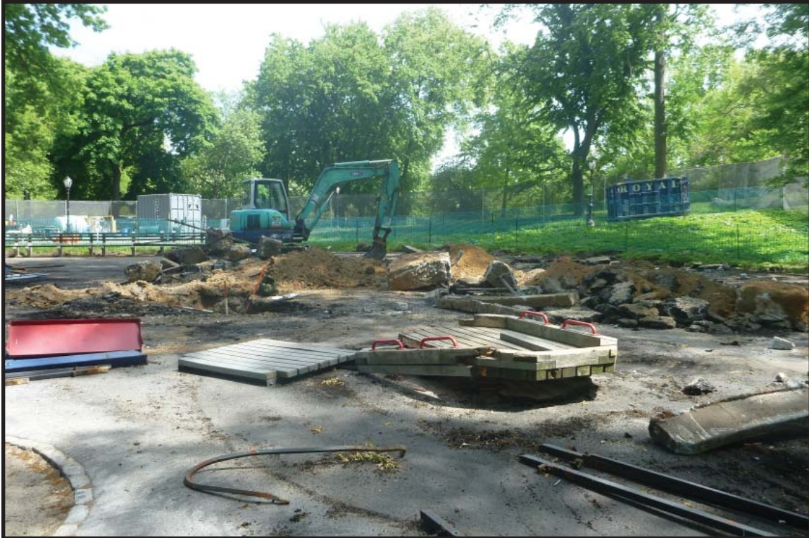
Photograph 3.4. Mariners' Playground, general view facing southeast showing the southern end of the playground during demolition (Photographer: James Lee, May 2016) [HRI Neg.#16020/D1:030].
