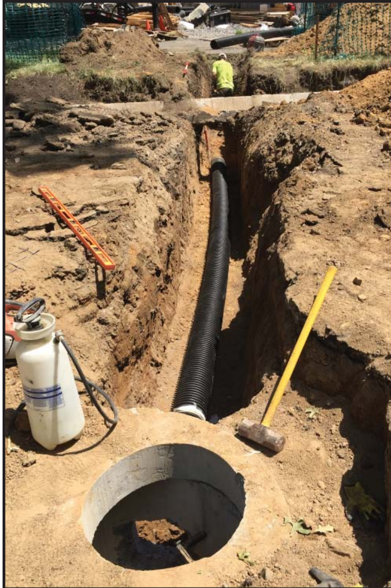
Photograph 3.14. Mariners' Playground, view facing southeast showing Contractor Excavation 6, a trench extending from a newly installed concrete manhole inside the playground to an existing storm drain outside of the playground (Photographer: James Lee, June 2016) [HRI Neg.#16020/D2:011].
