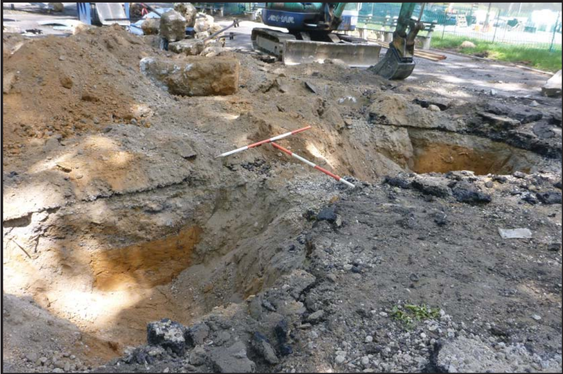
Photograph 3.6. Mariners' Playground, view facing east showing the Contractor Excavations 1 and 2 (right to left) at the southern end of the playground. These excavations were conducted in order to remove the footings of a swing set. Scale rods are in feet (Photographer: James Lee, May 2016) [HRI Neg.#16020/D1:020].
