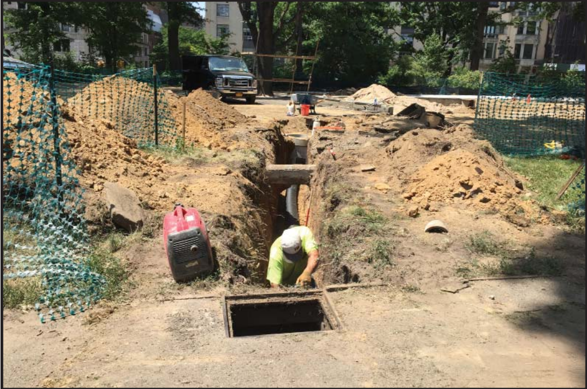
Photograph 3.15. Mariners' Playground, view facing northwest showing Contractor Excavation 6 extending from an existing storm drain outside of the playground to a newly installed concrete manhole inside the playground (Photographer: James Lee, June 2016) [HRI Neg.#16020/D2:004].
