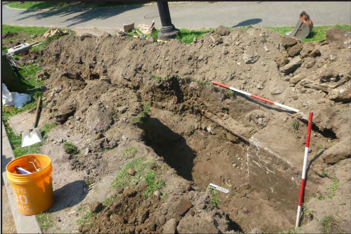
Photograph B.11. View facing southwest showing completed excavation and partial installation at SLB #12 and SLF #12 (installed top left of frame) (Photographer: Joshua Butchko, May 2021 [HRI Neg.#21036/D2:095]).
