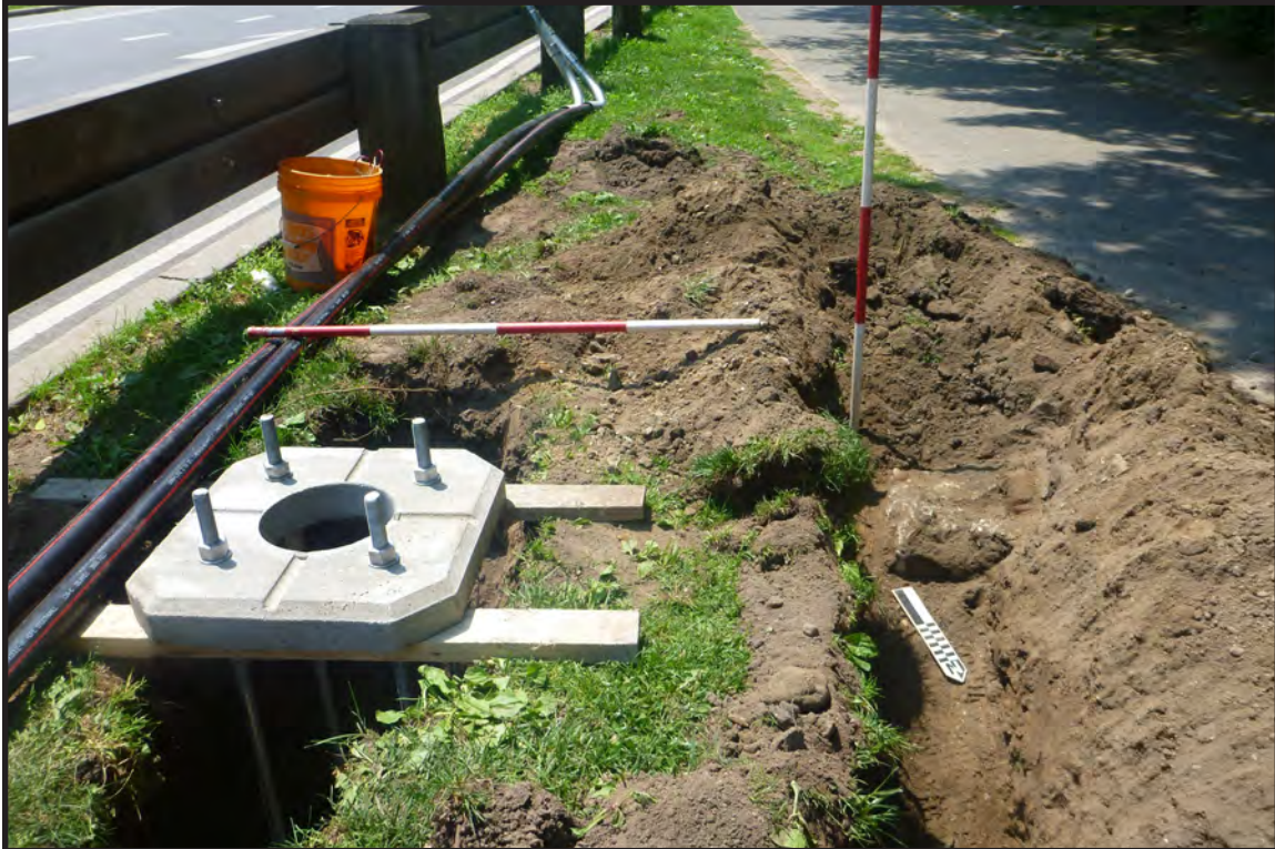
Photograph B.12. View facing southwest showing completed excavation and partial installation at SLF #12 showing concrete footing in connector trench (right of frame) (Photographer: Joshua Butchko, May 2021 [HRI Neg.#21036/D2:105]).
