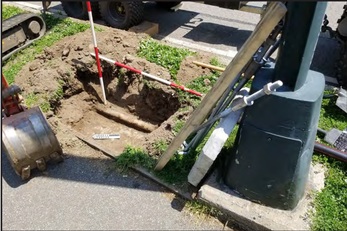
Photograph B.10. View facing east showing utility pipe and concrete surface exposed in SLF #10 (Photographer: Joshua Butchko, May 2021 [HRI Neg.#21036/D1:167]).
