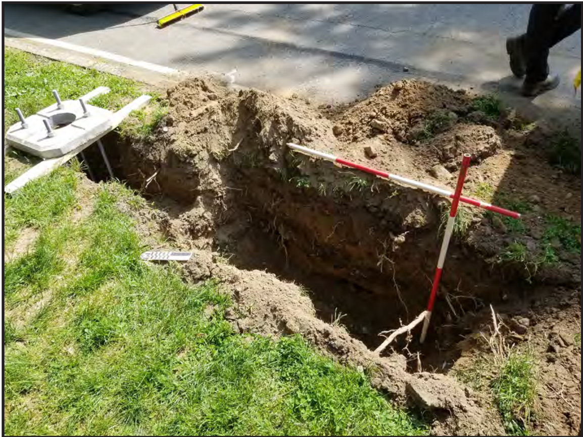
Photograph B.2. View facing southwest showing completed excavation and partial installation at SLB #5 at right and SLF #9 (Photographer: Joshua Butchko, May 2021 [HRI Neg.#21036/D1:156]).
