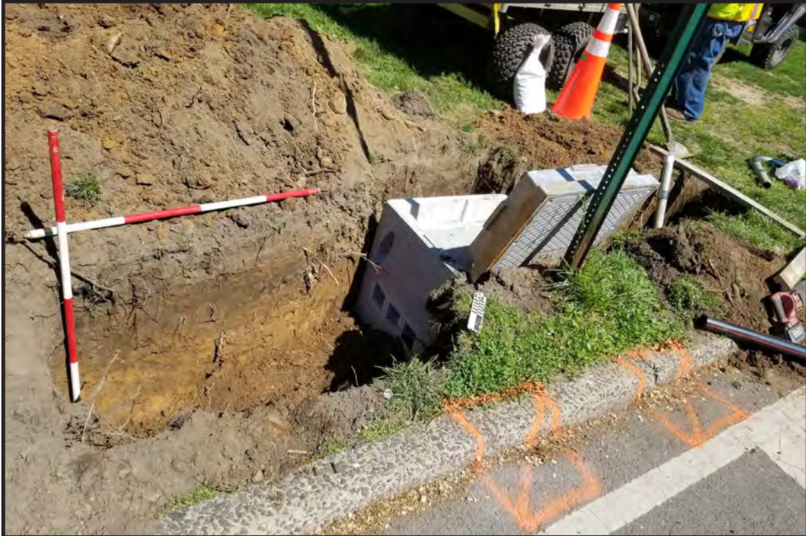
Photograph B.4. View facing north-northwest showing completed excavation and partial installation at SLB #1, SLB #2 (open left of frame) and SLF #2 (Photographer: Joshua Butchko, May 2021 [HRI Neg.#21036/D1:037]).
