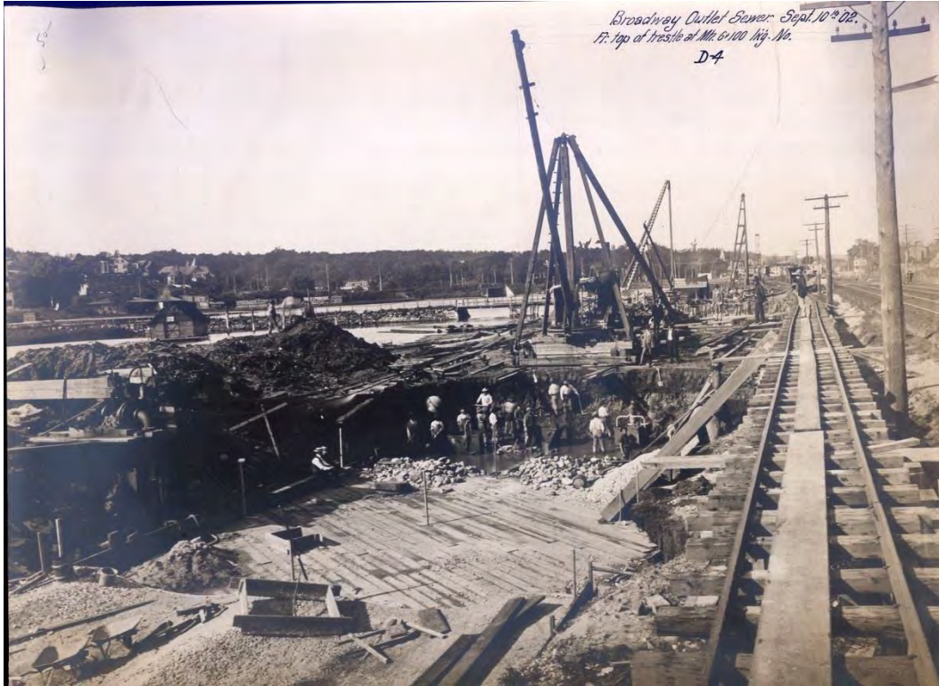
1902 view of the Broadway sewer under construction. The project site is on the far right. Courtesy City of New York Department of Sewers.
