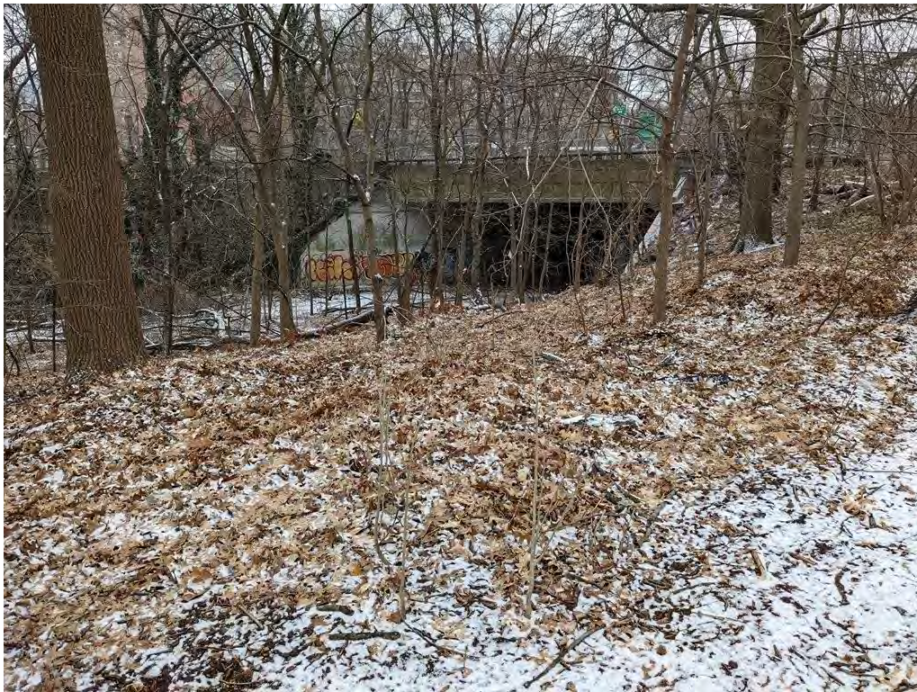
Photograph 12. The APE showing the Van Cortlandt Park South overpass. View looking southeast.
