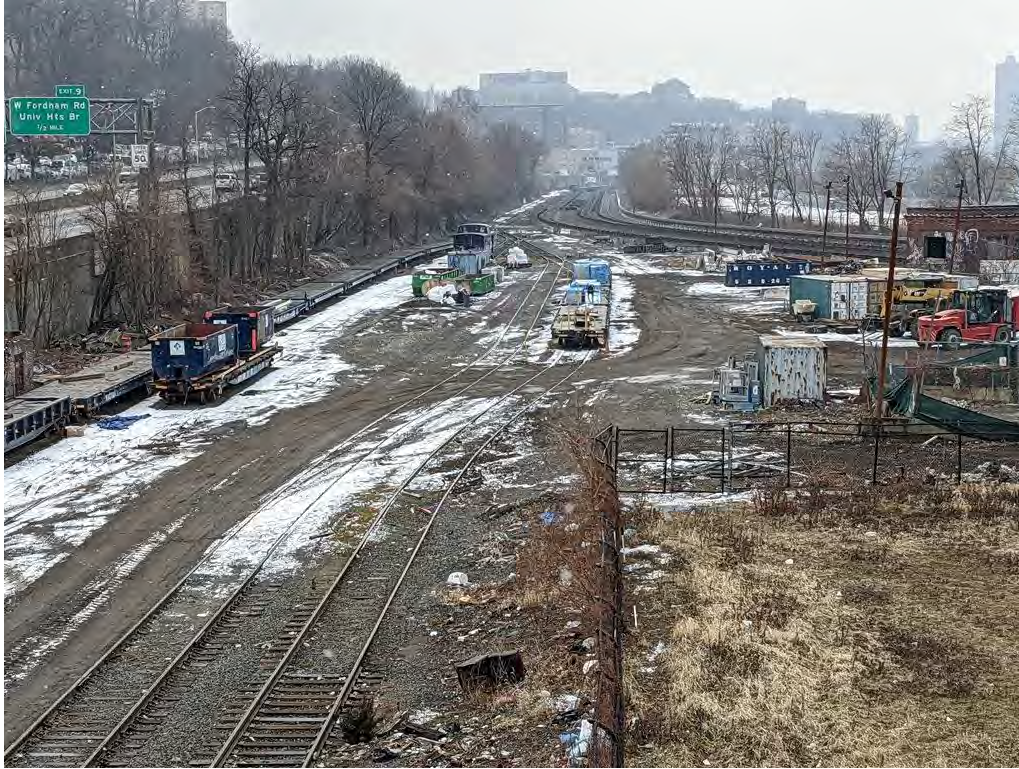
Photograph 29. The MTA Metro-North-owned portion of the APE, looking southeast towards the Harlem River outfall location. The proposed underground conduit would be located between the railroad tracks and Interstate 87 on the left, and the cross under the tracks toward the Harlem River in the far background.
