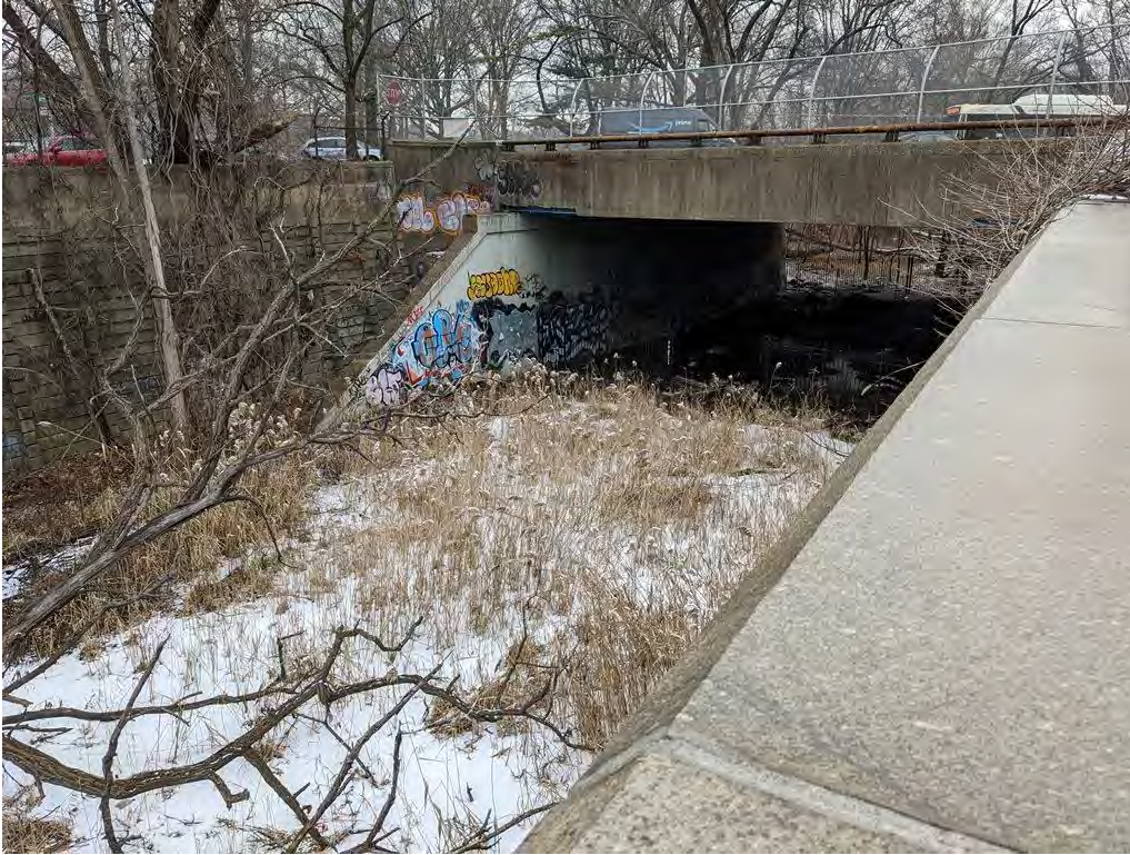
Photograph 13. The CSX-owned portion of the APE, looking north toward the Van Cortlandt Park South overpass.
