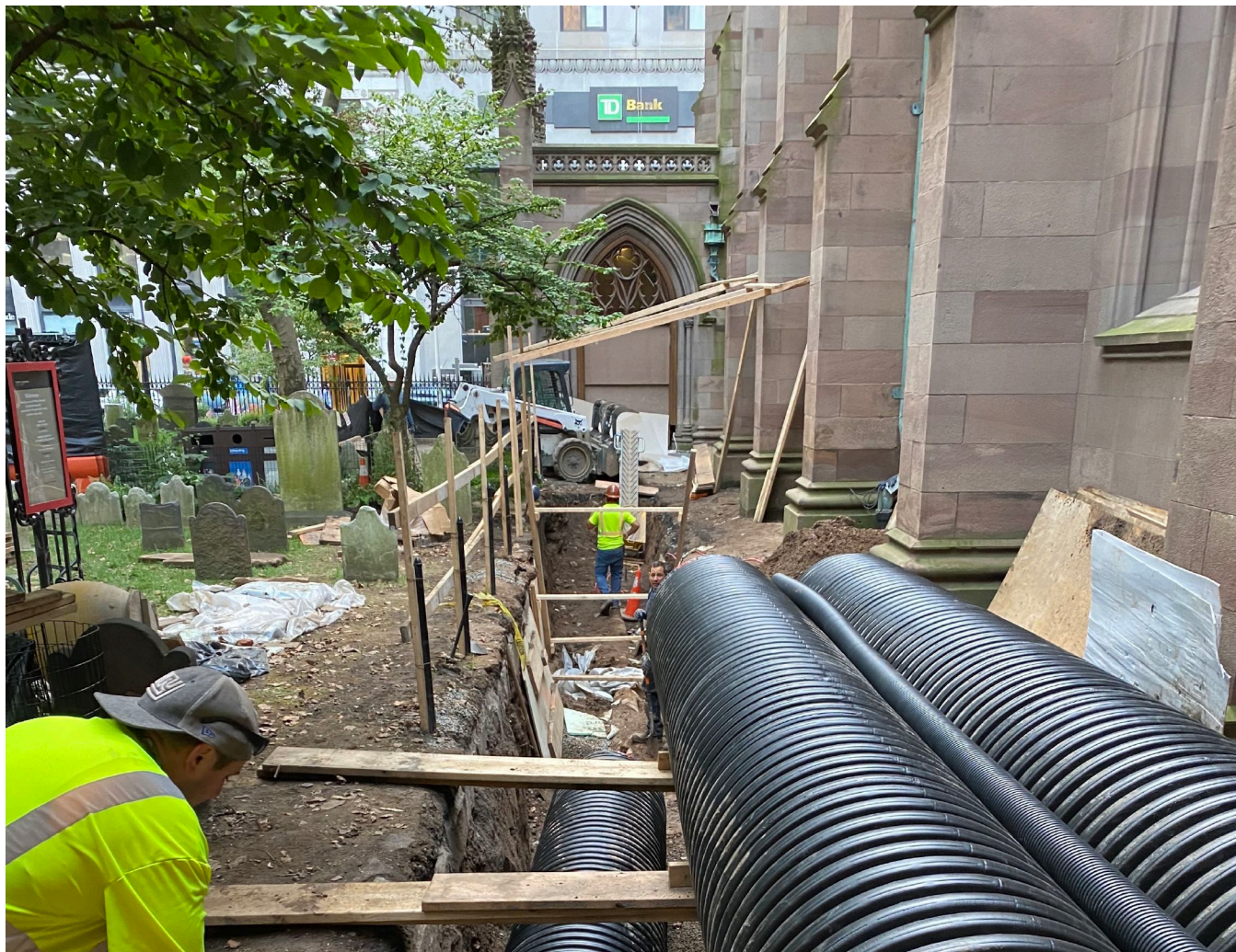
North Pipeline Trench looking east toward the Northeast Vestibule during pipe installation (S. Wiedre 9/15/2022)
