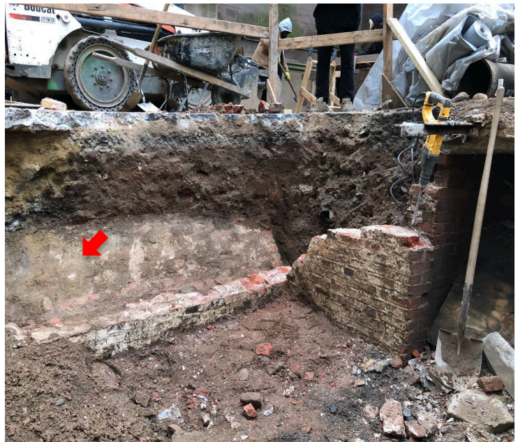
Photo 29. The Van Horne burial vault (foreground) prepared for reconstruction. The view is southwest. The north side of the abutting unidentified vault (arrow) is exposed (see Photo 20). (J. Geismar 12/8/2020)
