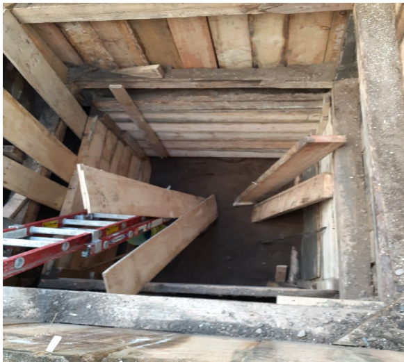
Photo 26. TP with shoring, here at c. 9.5 ft. (3.0 m) bgs. Screened soil from this depth is shown in Photo 27. (S. Spritzer 10/7/2020)
