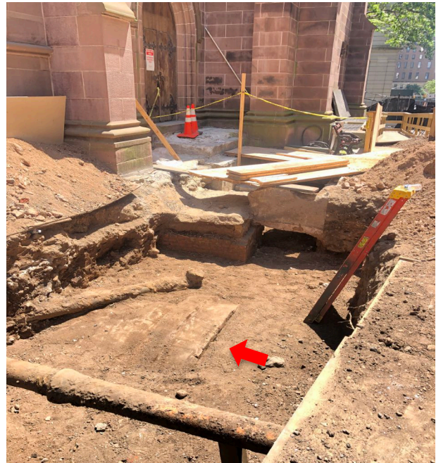
Photo 7. Looking south along the rear (west) wall of the church. The arched dome of a burial vault (arrow) is one of two minimally exposed vaults in the shallow, expanded excavation. The drainage trench is located beyond the photo to the right. (C. Look 6/19/2020)
