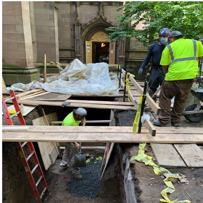
Photo 13. Following the burial service, Richie Fiore, LIC Contractor Superintendent, wrapped Burial 1 and covered it with protective gravel in the North Pipeline Trench where it was discovered. The view is west looking toward All Saints Chapel. (J. Geismar 9/1/2020)
