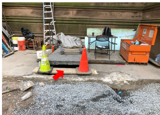
Photo 33. Access to the vault is under the bluestone slab behind the two cones (arrow). The bluestone slab, here propped up, was later installed. (J. Geismar 1/8/2021)
