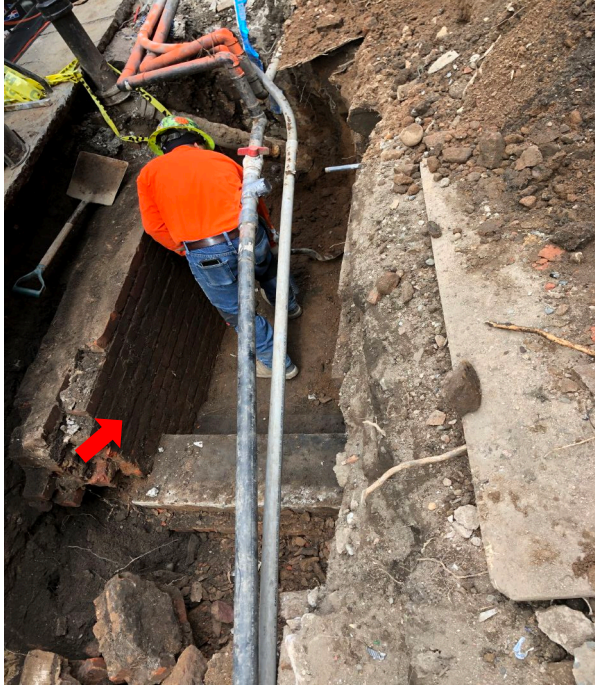
Photo 4. Brick feature (arrow), dubbed “The Boiler Room,” exposed along the west wall of trench. The longitudinal pipes are sprinkler water feeds found throughout the trench. (J. Geismar 3/5/2020)
