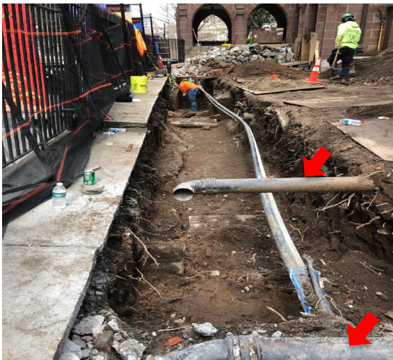
Photo 2. NW Drainage Trench looking north to the loggia in the far background. The Trinity Place wall and fence are to the left. Shallow drainage pipes (arrows) are exposed. The long north-south lines are sprinkler water feeds. (J. Geismar 3/11/2020)
