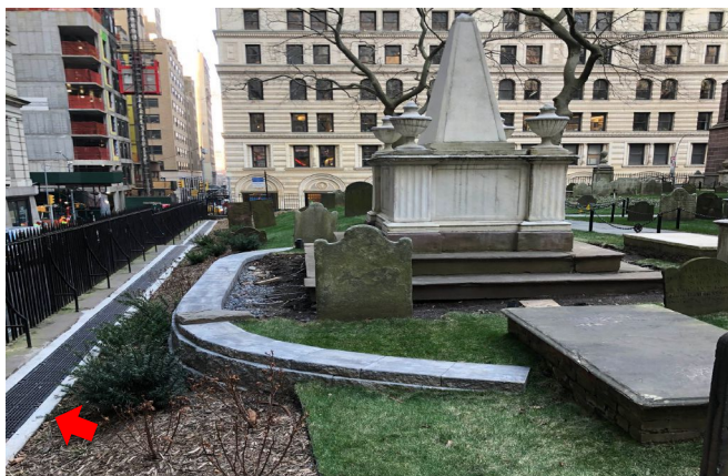
Photo 24. The new stone retaining wall associated with the Alexander Hamilton monument. The view is west. The South Drainage Trench (arrow) is also completed. (J. Geismar 3/23/2021)
