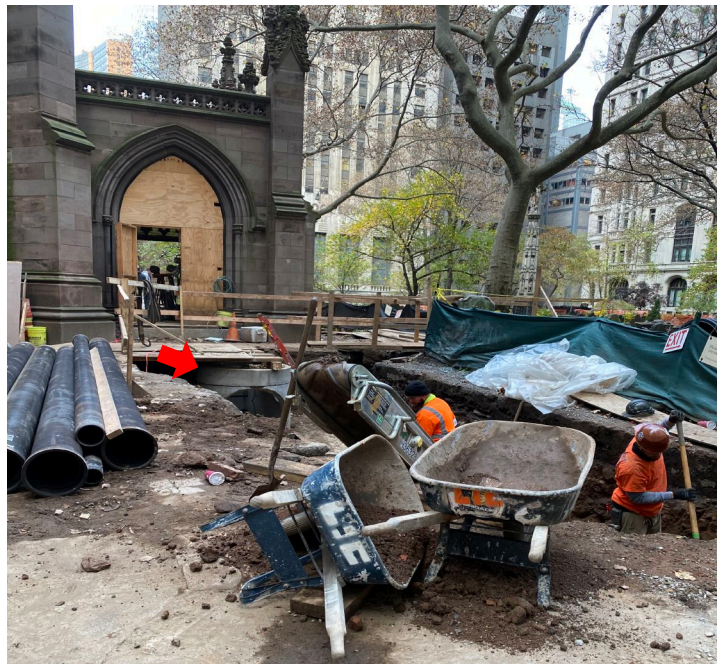
Photo 18. Northeast Drainage Trench, looking west with a catch basin (arrow) east of the Northeast Vestibule. (S. Wierdre 11/17/2020). Wheelbarrows were used to transport
