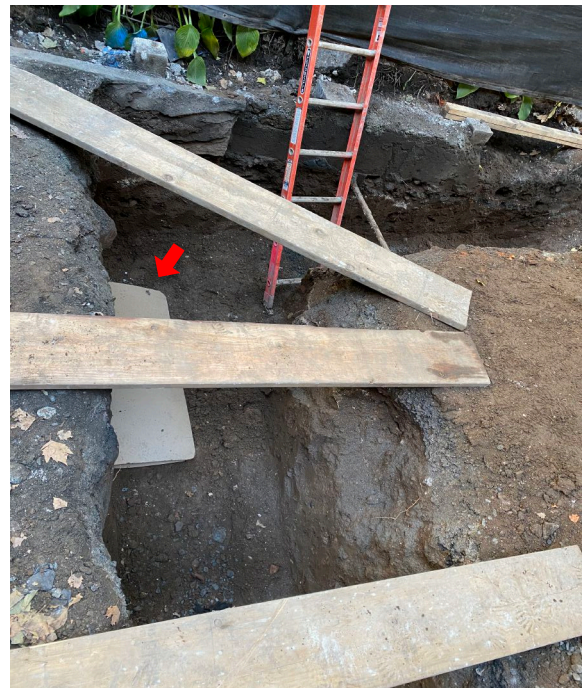
Photo 17. West leg of the Connector Trench where a cache of human bone was found under trashed tombstones (here covered with plywood [arrow]) south of the trench's northeast corner (S. Wierdre 11/5/2020)
