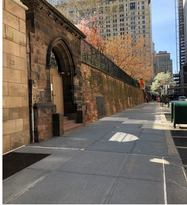
Photo 5. The Trinity Place wall from the street. The NW Drainage trench ran along the stone wall below the iron fence (see Photo 2). (J. Geismar 4/14/2021)
