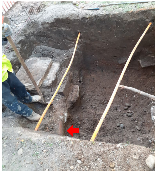
Photo 25. TP in southwest corner of the south churchyard excavated to c. 5.5 ft. (1.7 m) bgs. Note terra-cotta pipe (arrow), a component of a former drainage system found during Phase 1 Oversight. (S. Spritzer 9/22/20)
