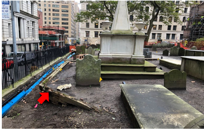
Photo 22. Old tie rod retaining wall (arrow) adjacent to the Alexander Hamilton memorial in the south churchyard prior to its removal. The view is west. Excavation of the South Drainage Trench (far left) is underway (J. Geismar 10/21/2020)
