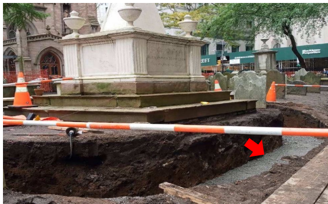
Photo 23. Retaining wall trench after excavation. Gravel (arrow) has been introduced into the trench. The view is east. (D. Howe 10/27/2020).
