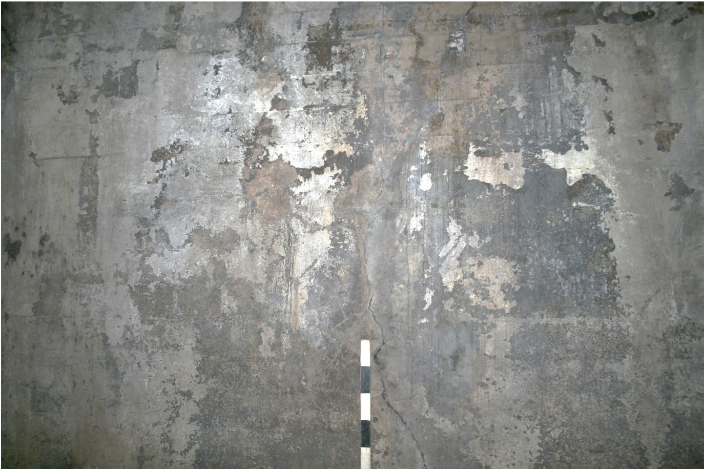
Photograph 10: Facing south to poured concrete south wall in south half of Vault C.
