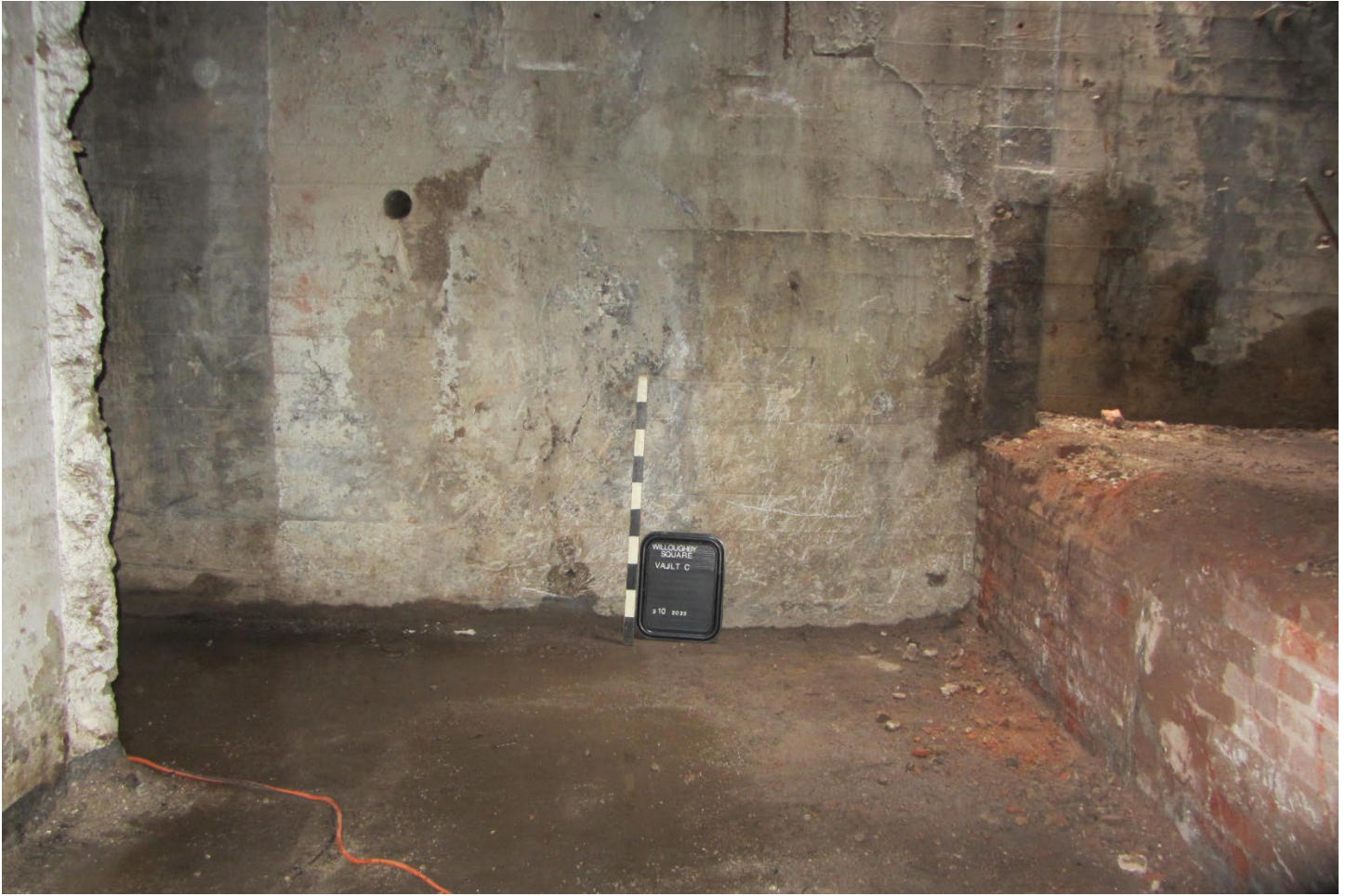
Photograph 17: Facing west to poured concrete west wall in north half of Vault C, with remnants of brick north wall (right). Note: base of Vault C is three feet below the base of Vault B to north (right).
