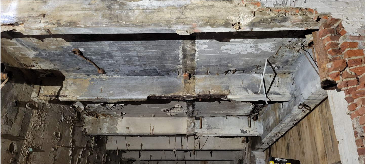
Photograph 1: Facing north to ceiling of Vault B from Vault C. Note: remnant of brick wall between Vault B and Vault C removed as part of this project (right).
