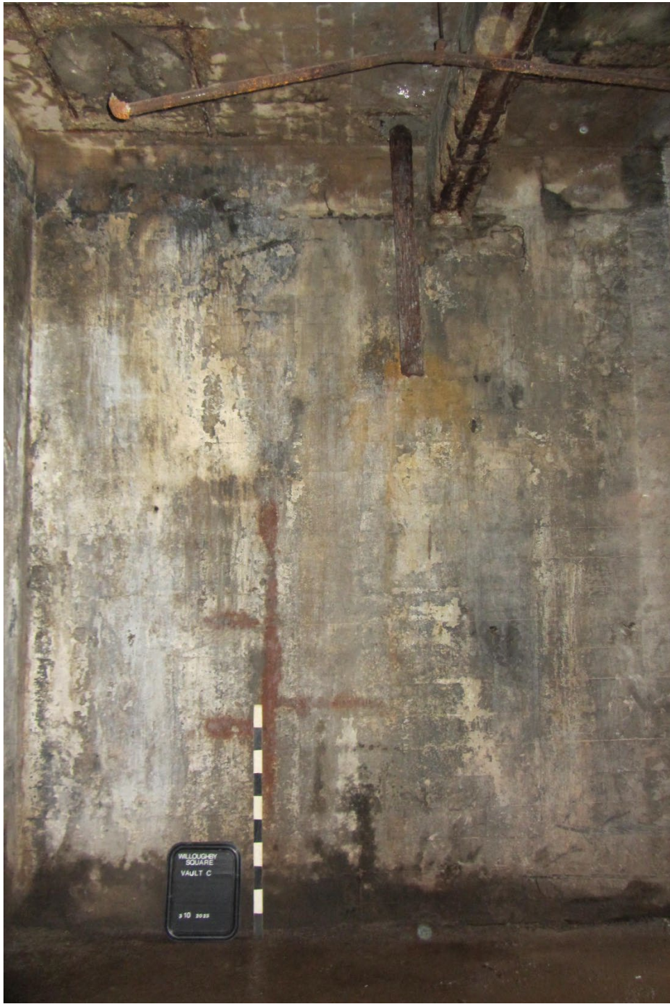
Photograph 12: Facing west to poured concrete west wall in south half of Vault C with formerly bricked in opening between the north and south halves of Vault C at right.
