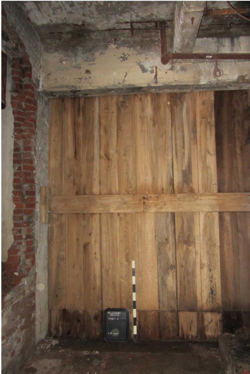
Photograph 16: Facing east to east wall (center) and opening in north half of Vault C with remnants of brick north wall (left). Note: the formerly bricked in opening in the east wall was removed and replaced with wood as part of this project.
