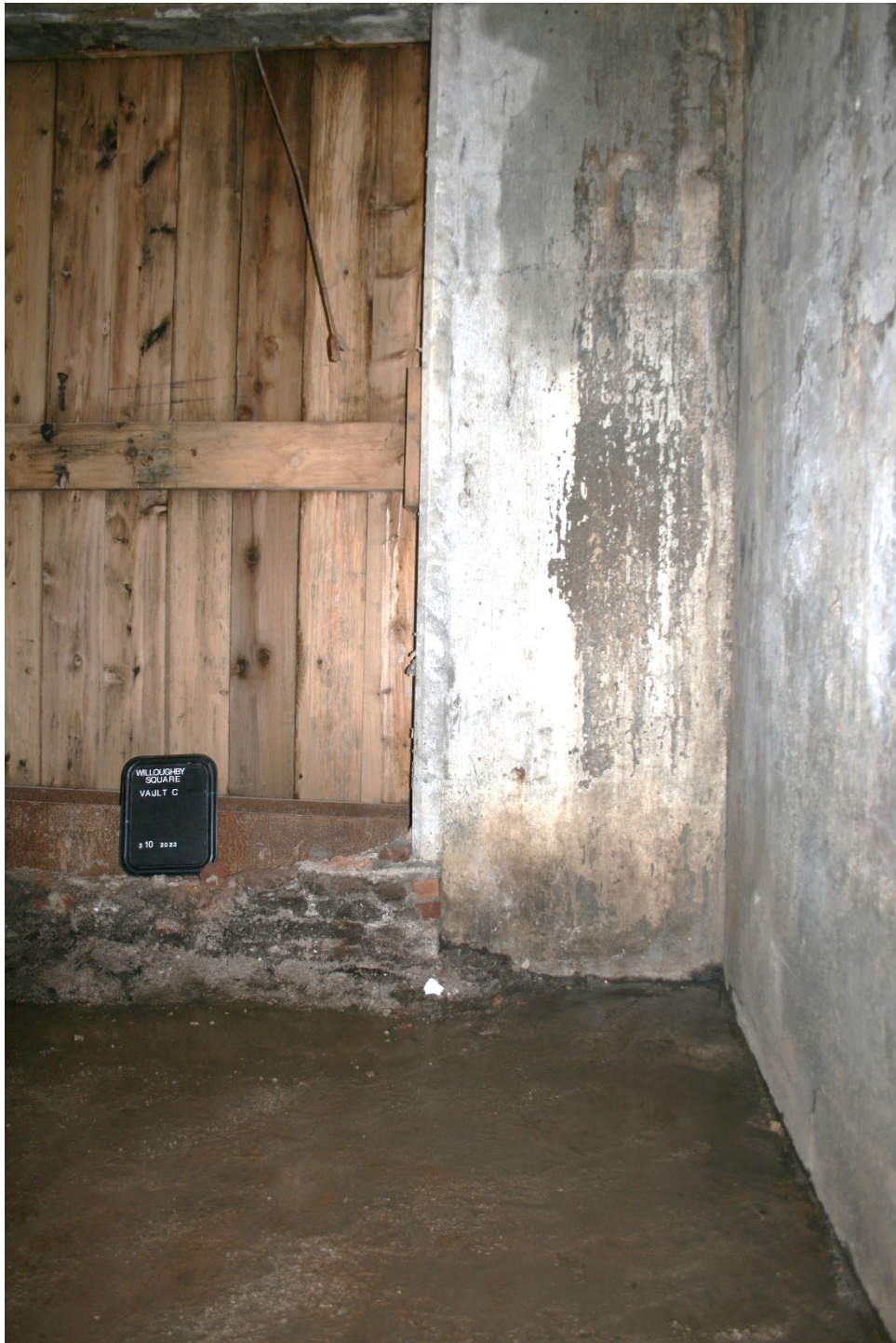
Photograph 8: Facing east to poured concrete east wall and opening in south half of Vault C, with southern wall at right. Note remnants of the formerly bricked in opening (beneath sign) with the remainder removed and replaced with wood as part of this project.
