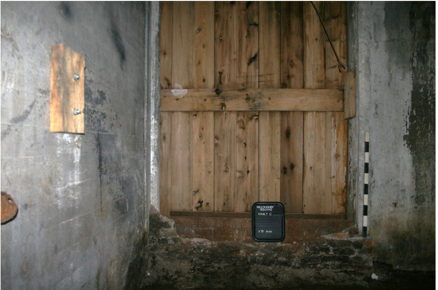
Photograph 9: Facing east to east wall and opening in south half of Vault C with poured concrete north wall at left. Note remnants of the formerly bricked in opening (beneath sign) with the remainder removed and replaced with wood as part of this project.
