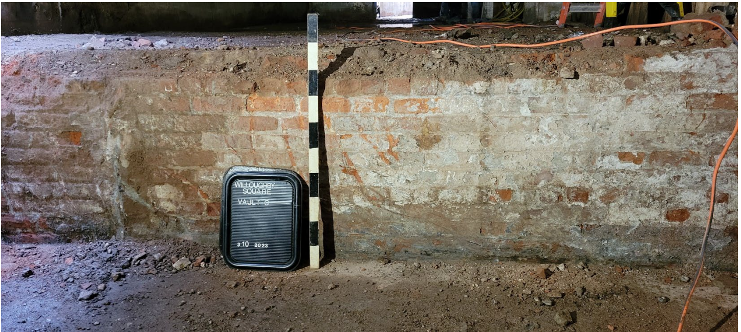
Photograph 18: Facing north to remnant of brick north wall in north half of Vault C. Note: base of Vault C is 3 feet one inch below the base of Vault B to north.
