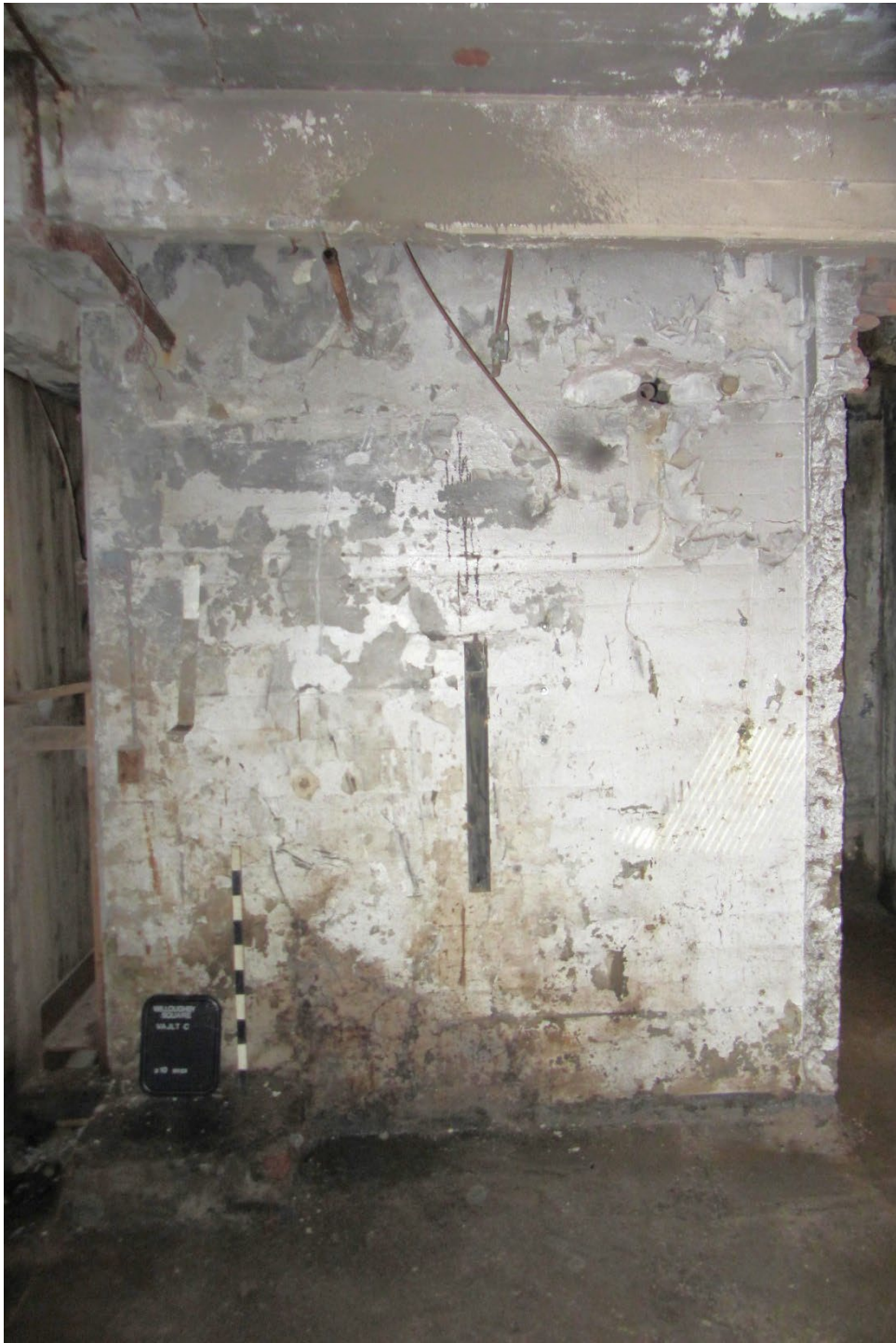
Photograph 14: Facing south to poured concrete south wall in north half of Vault C. Note: this wall divides Vault C in two halves. Formerly bricked in openings at east (left) and right (west) were removed as part of this project.
