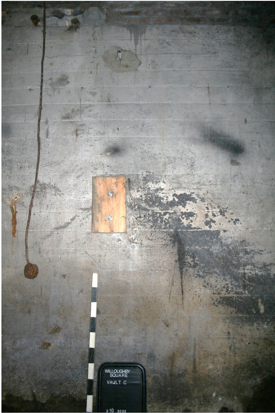
Photograph 11: Facing north to poured concrete north wall with brick infill at top in south half of Vault C. Note: this wall divides Vault C in two halves.
