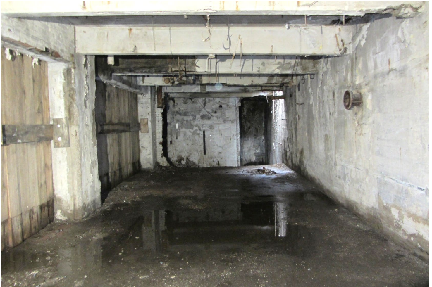
Photograph 3: Facing south from center of Vault B to south end of Vault B and north half of Vault C. Note: the eastern wall of Vault B (left) has two formerly bricked in openings that were removed and replaced with wood as part of this project.
