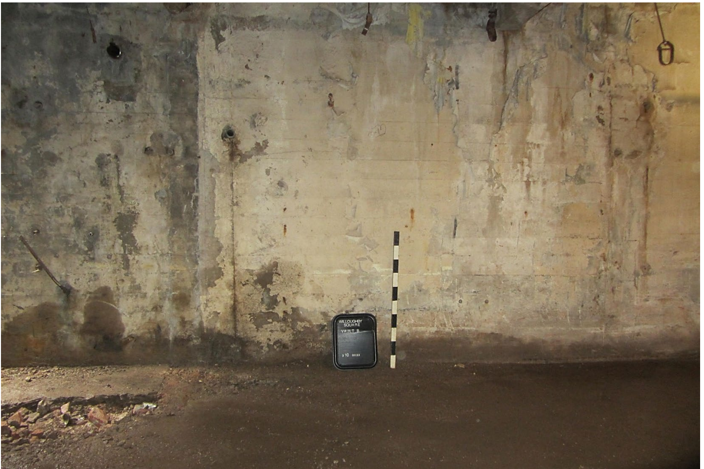
Photograph 2: Facing west to poured concrete west wall of Vault B. Note: break in poured concrete floor (bottom left) is filled with demolition debris from current project.
