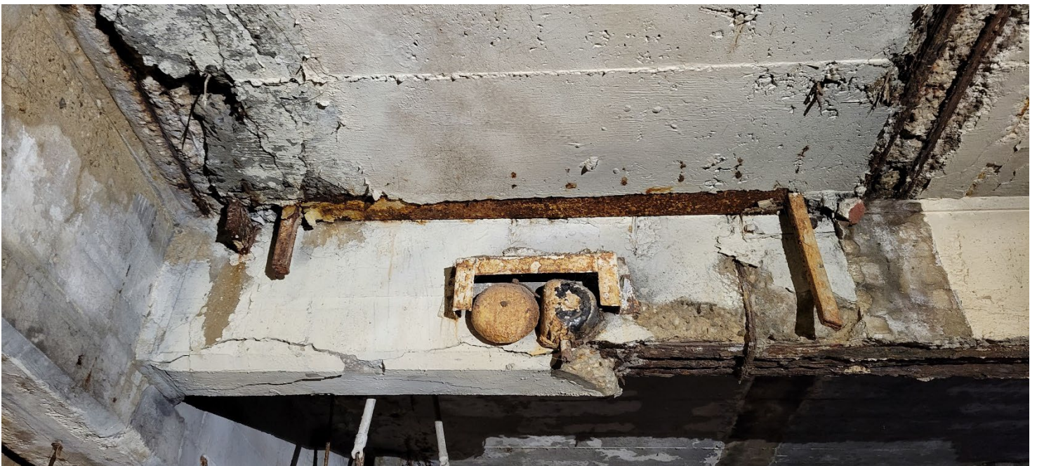
Photograph 4: Facing south to ceiling with remnants of alarm system mounted on poured concrete steel reinforced beam in Vault B.
