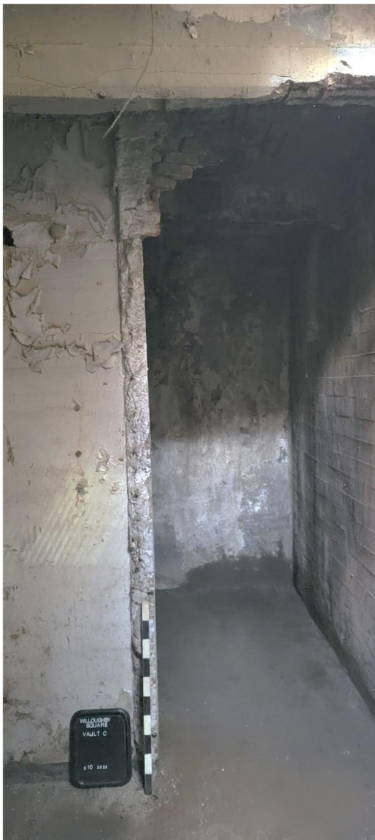
Photograph 15: Facing south to poured concrete dividing wall in north half of Vault C (foreground) and poured concrete south wall in south half of Vault C (background). Note: formerly bricked in opening at right removed as part of this project.
