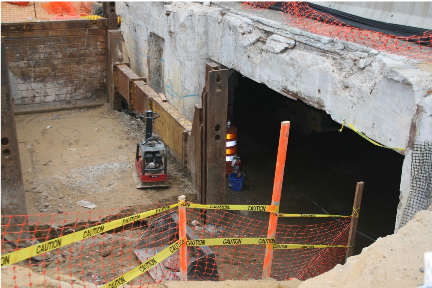
Photograph 6: Facing southwest to bricked in entrance (left) and formerly bricked in entrance (right) to Vault A.
