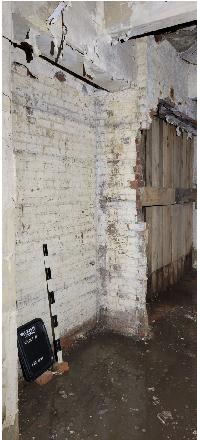
Photograph 5: Facing southeast to northeast corner of Vault B with bricked in former passageway (foreground). Note: formerly bricked in opening (background) was removed and replaced with wood as part of this project.
