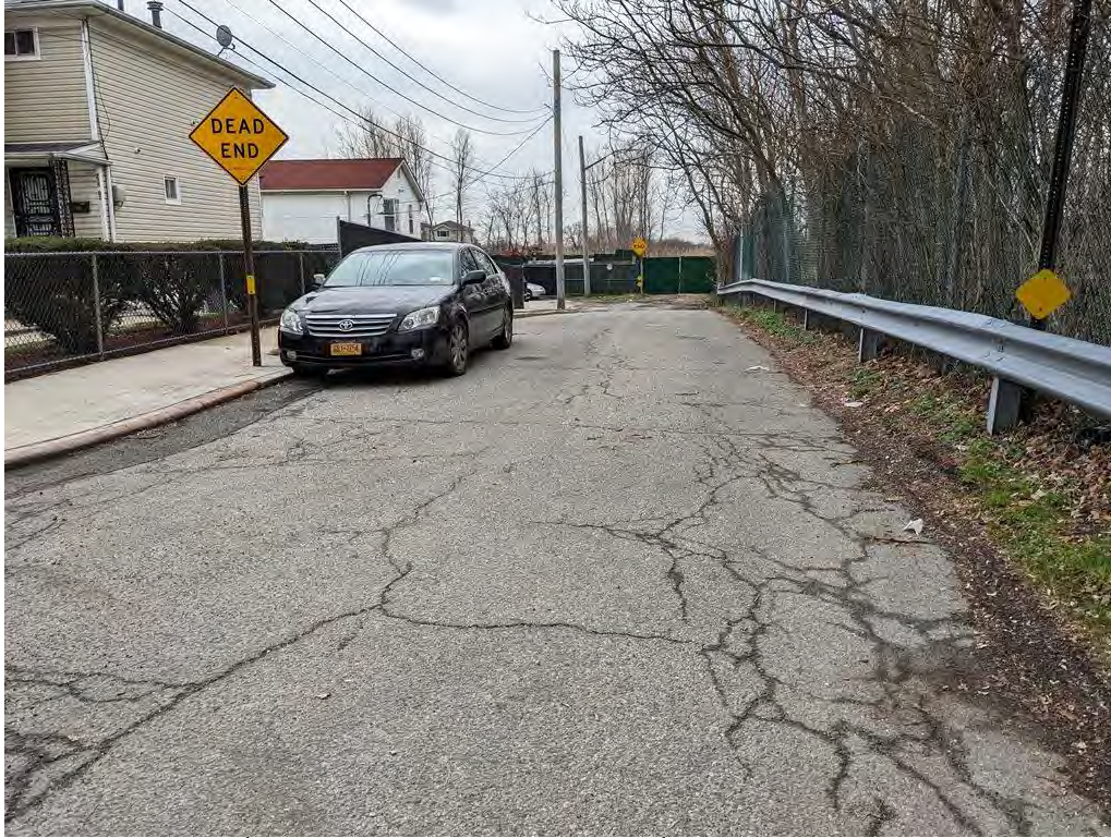
Photograph 19. 235 th Street looking southeast from 148 th Avenue. BMP #1 is on the right.
