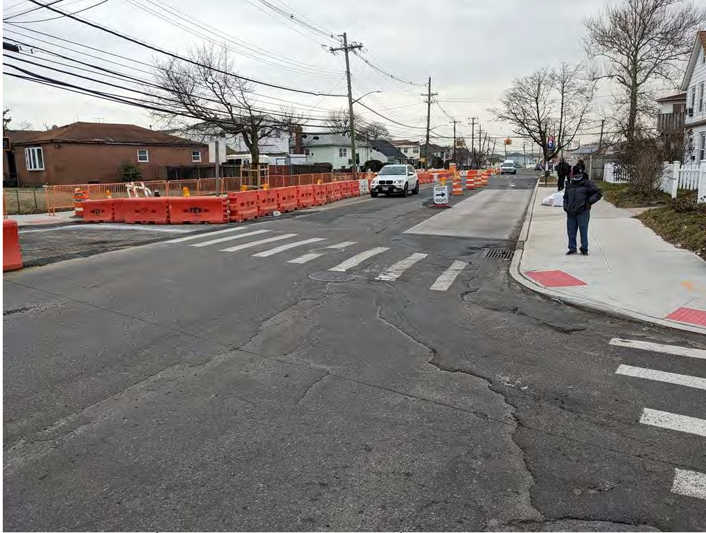
Photograph 33. 147 th Avenue looking west from 230 th Place, with road construction marked by barriers.
