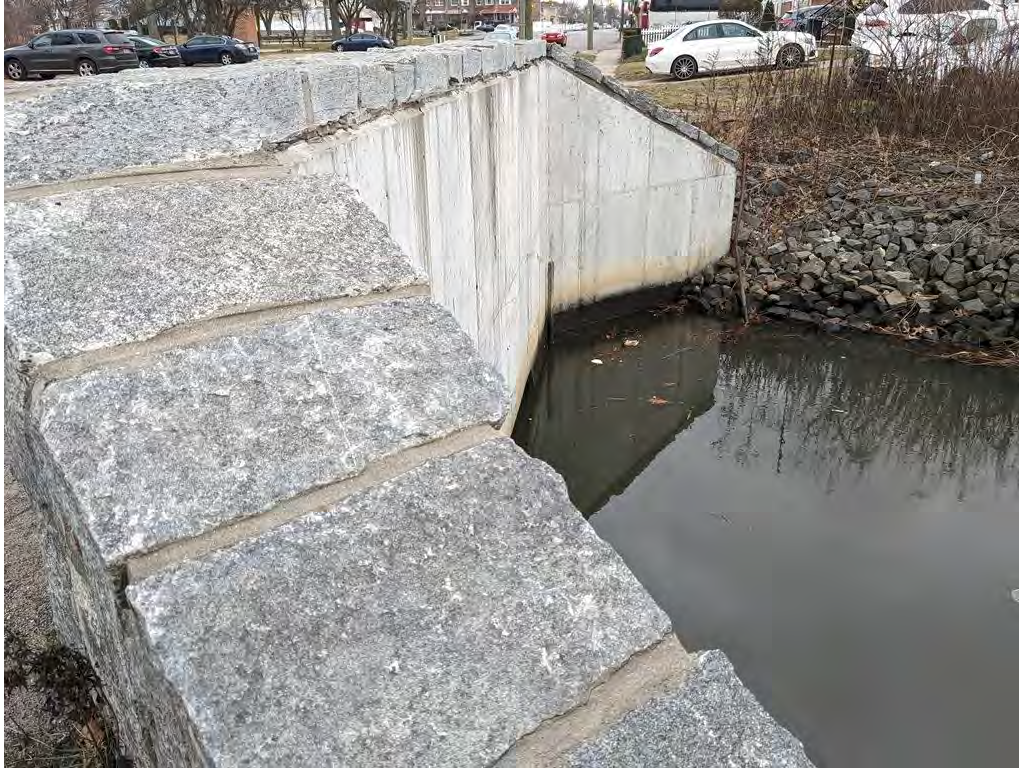
Photograph 25. Detail of the area on the downstream side of Conselyea's Creek where the new outfalls will be activated, looking northeast.
