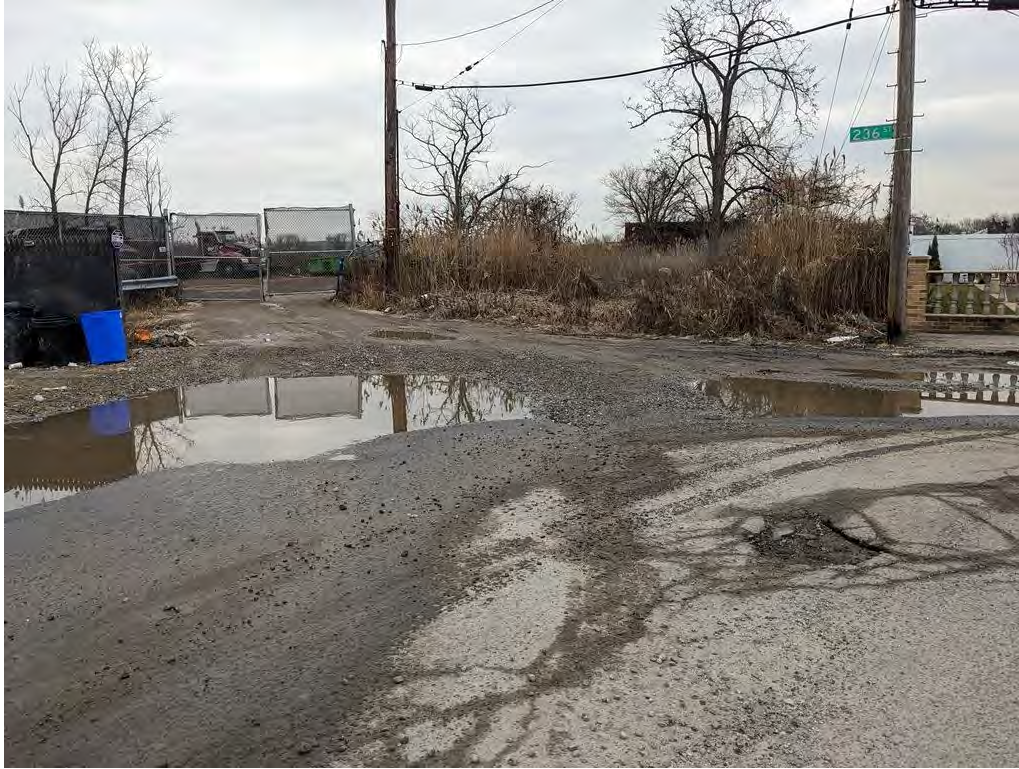
Photograph 45. The gate leading into the elevated portion of BMP #2. View looking west from 148 th Drive and 236 th Street.
