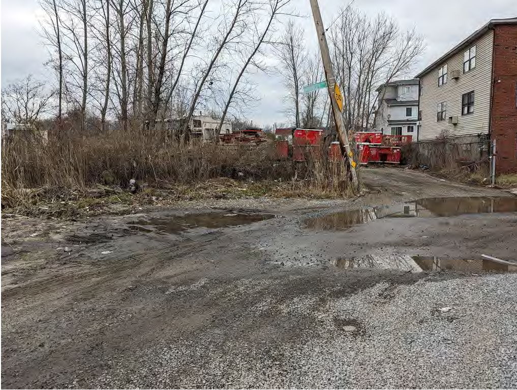
Photograph 43. BMP #2 showing the terminus of Bentley Road where a new outfall will be located. View looking northwest.
