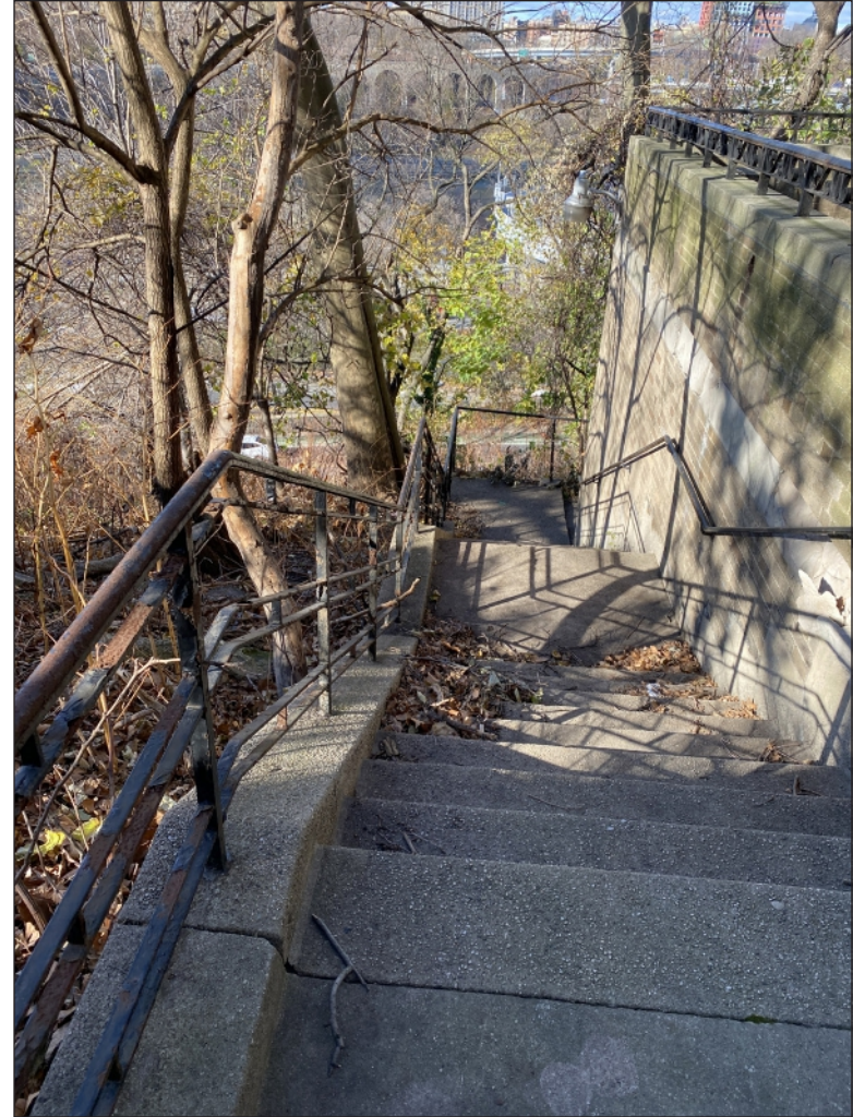
Stairs leading down the steep hills in the southern portion of the Project Site 8
