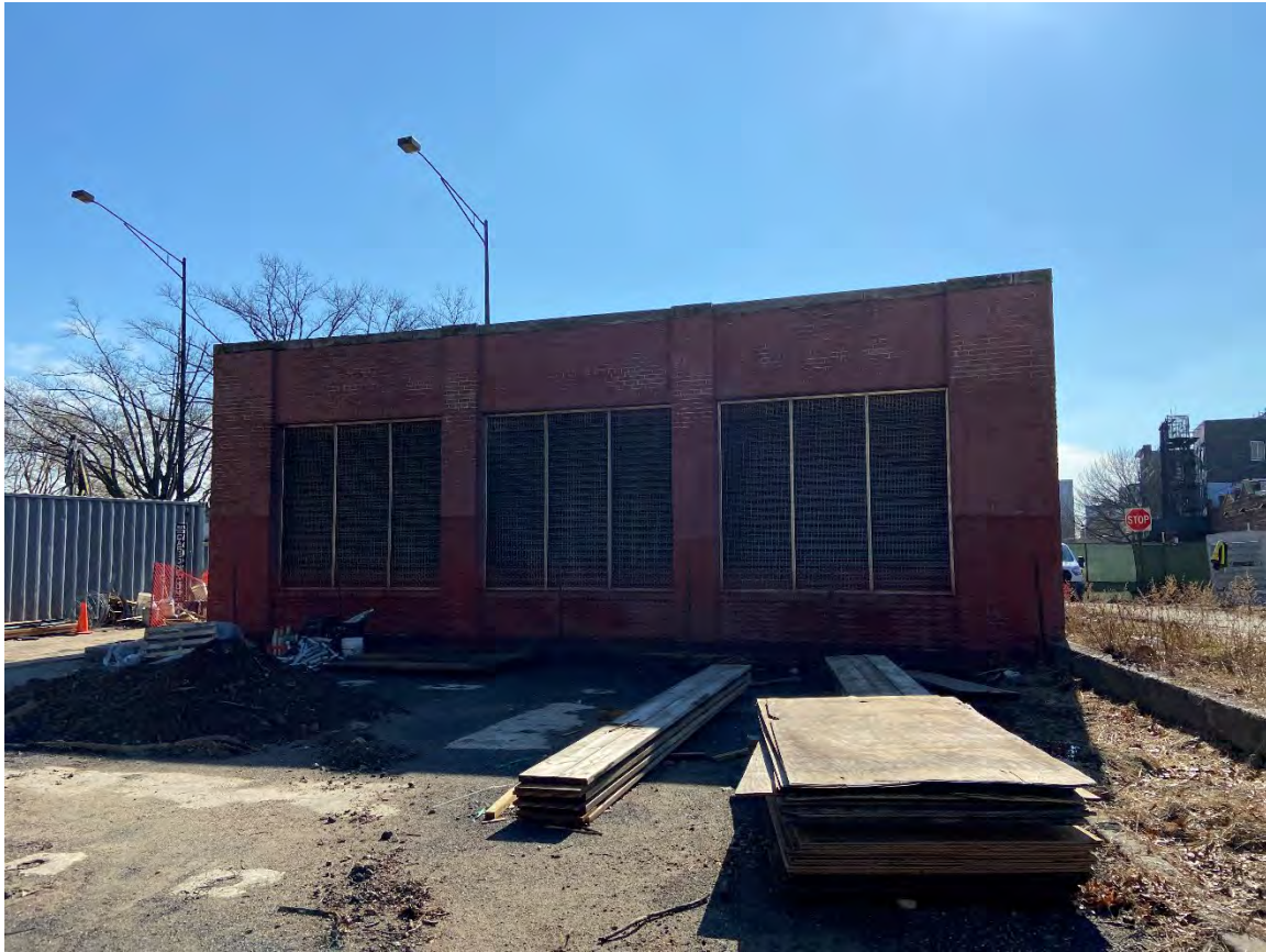
Photograph 8: Facing south in the Callahan-Kelly Playground, under construction, to the location of a proposed new Comfort Station and the extant MTA Vent Building, with Sackman Street within the Park at right.
