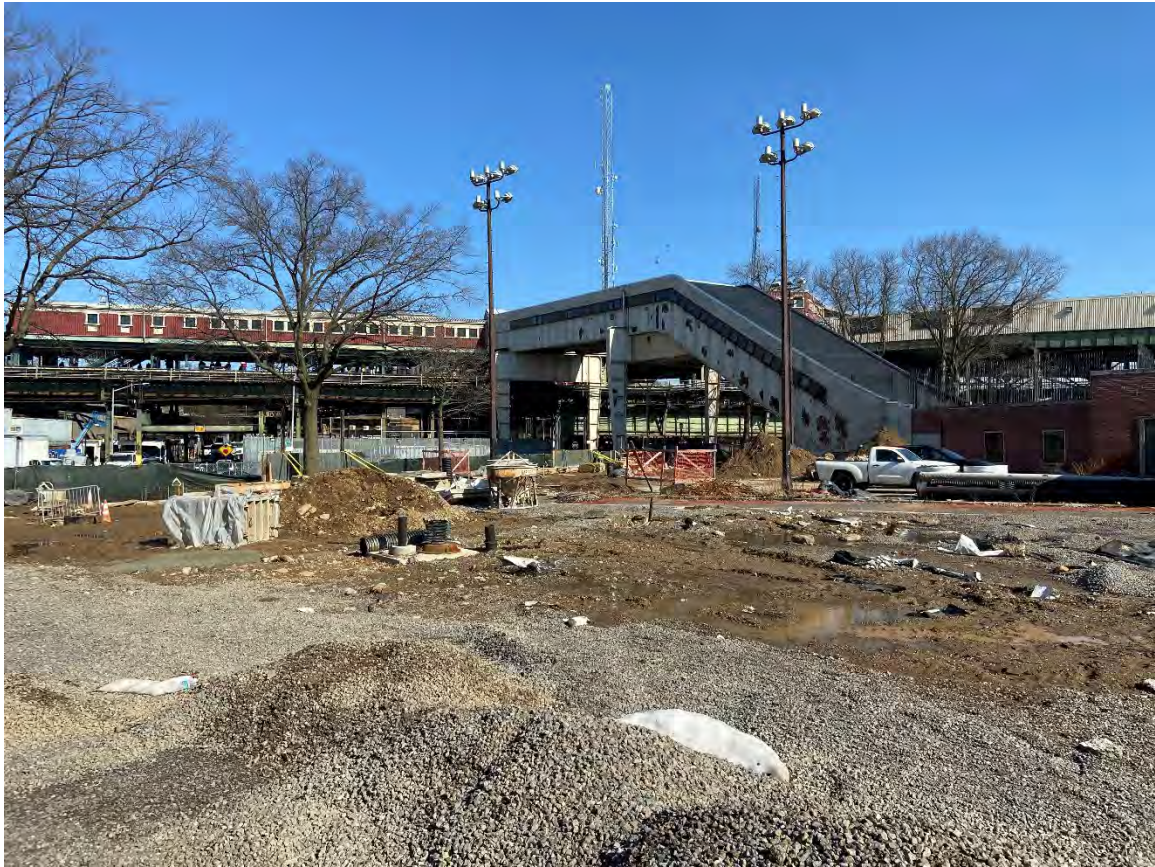
Photograph 10: Facing northeast from the Callahan-Kelly Playground to the Control House at center right and the escalator over Truxton Street to the J/Z Line over Broadway.
