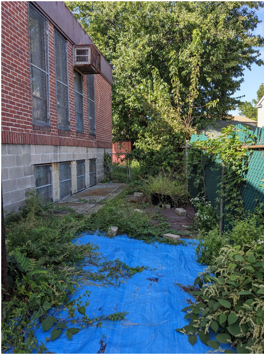
Photograph 22: Facing northwest from east side of church to overgrown area adjacent to addition at north end of building.
