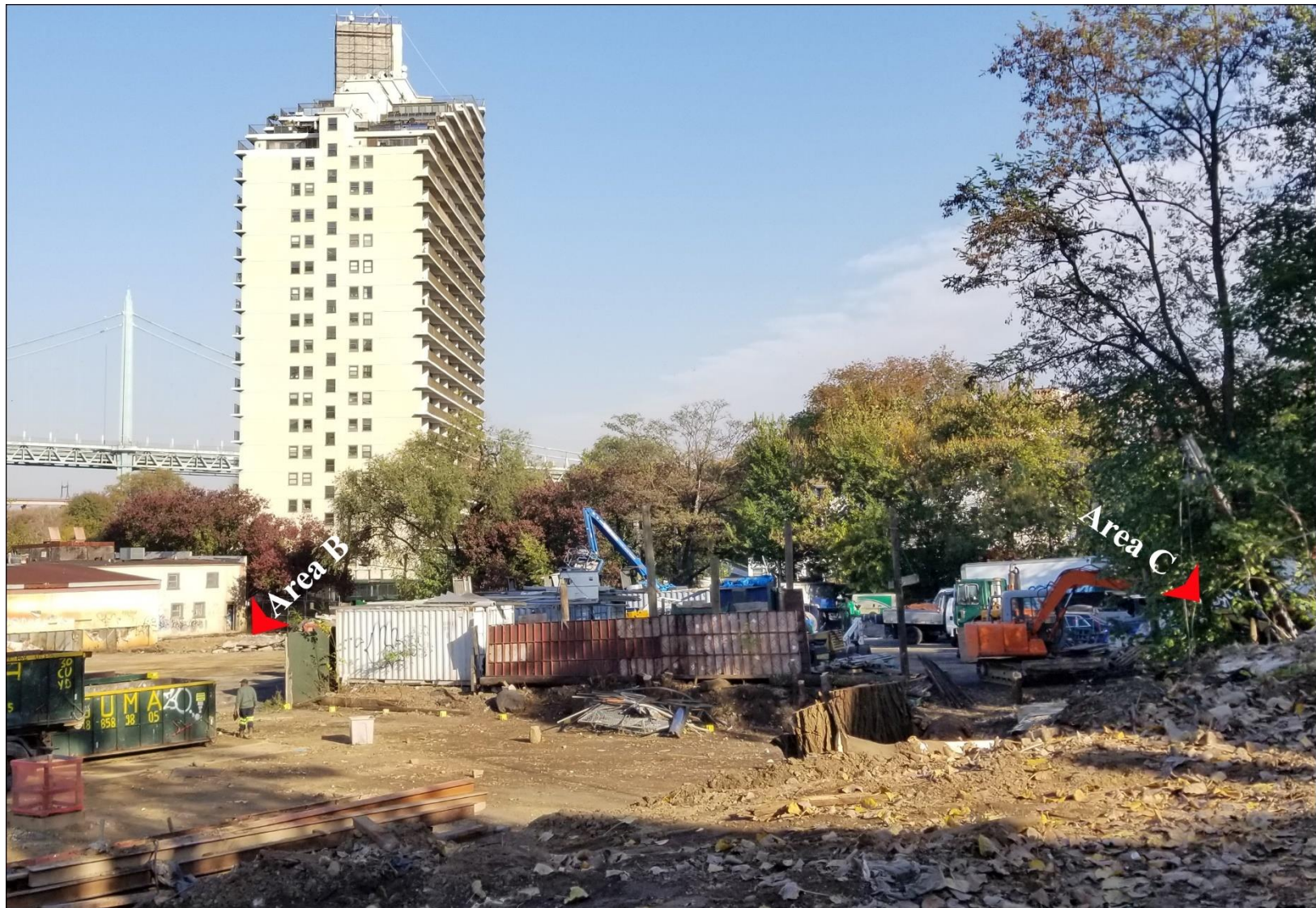
Fig. 27. AREAS B & C - View of Areas B and C from the northwestern edge of the hilltop, looking east.
