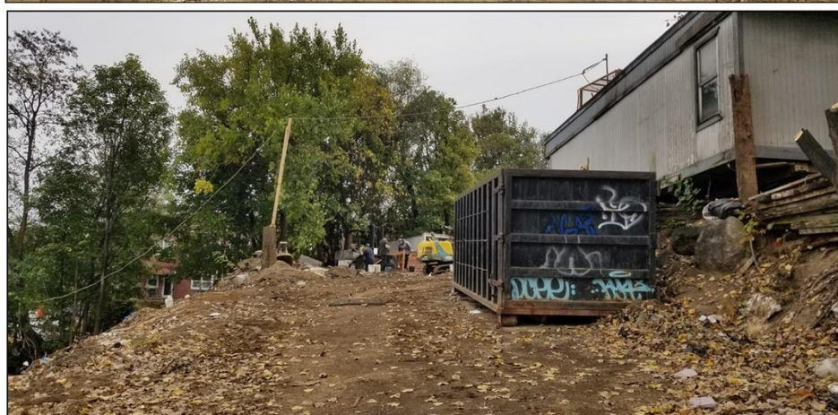
Fig. 12. (top) AREA H – Peripheral area not tested south of the Irregular Construction Fence, looking west.
