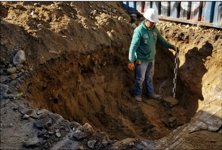
Fig. 18. (top) AREA R - View of the excavation with 27 th Avenue at the top (south).
