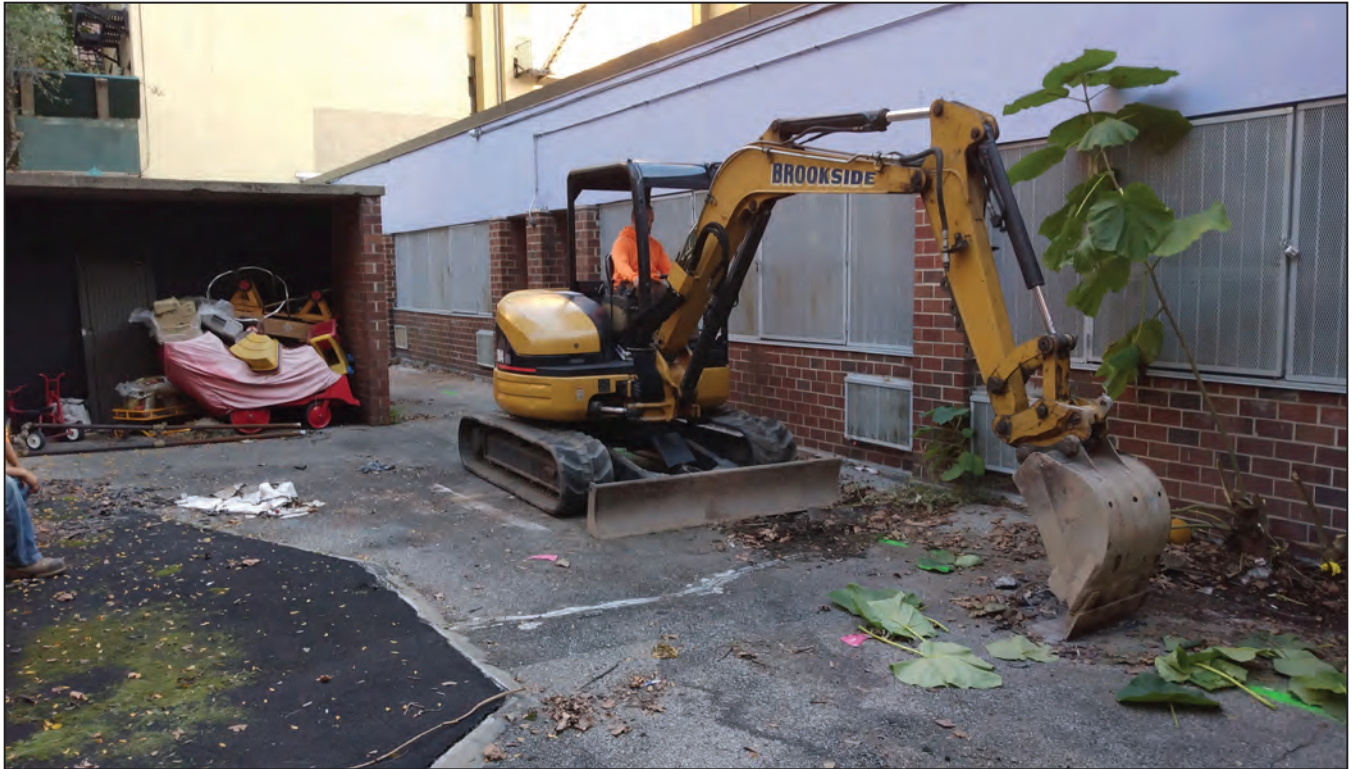
Facing northwest towards Trench 3, which was excavated adjacent to the 1-story brick building 11
