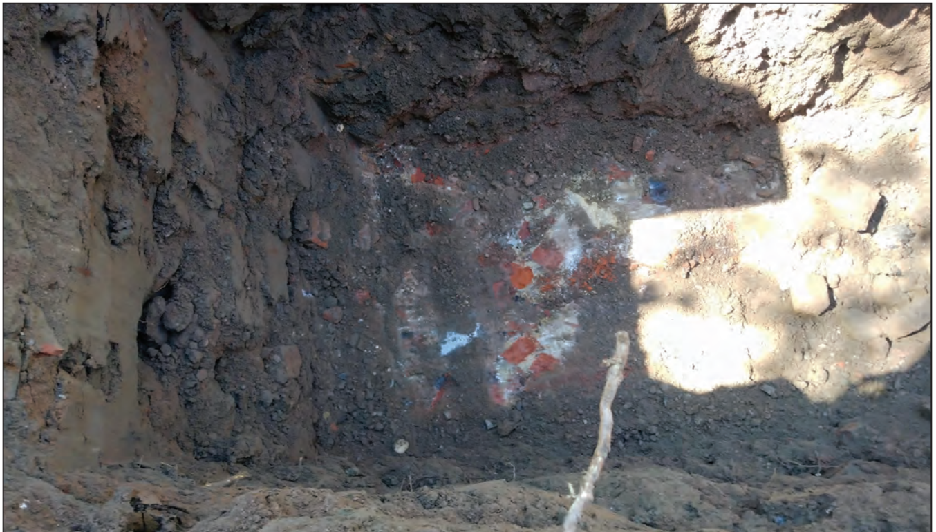
Detail of the floor of Trench 2 showing a concrete and brick foundation floor encountered at a depth of 6.5 feet below ground surface. The overlying soils consisted of loose sandy urban fill and brick demolition debris 10
