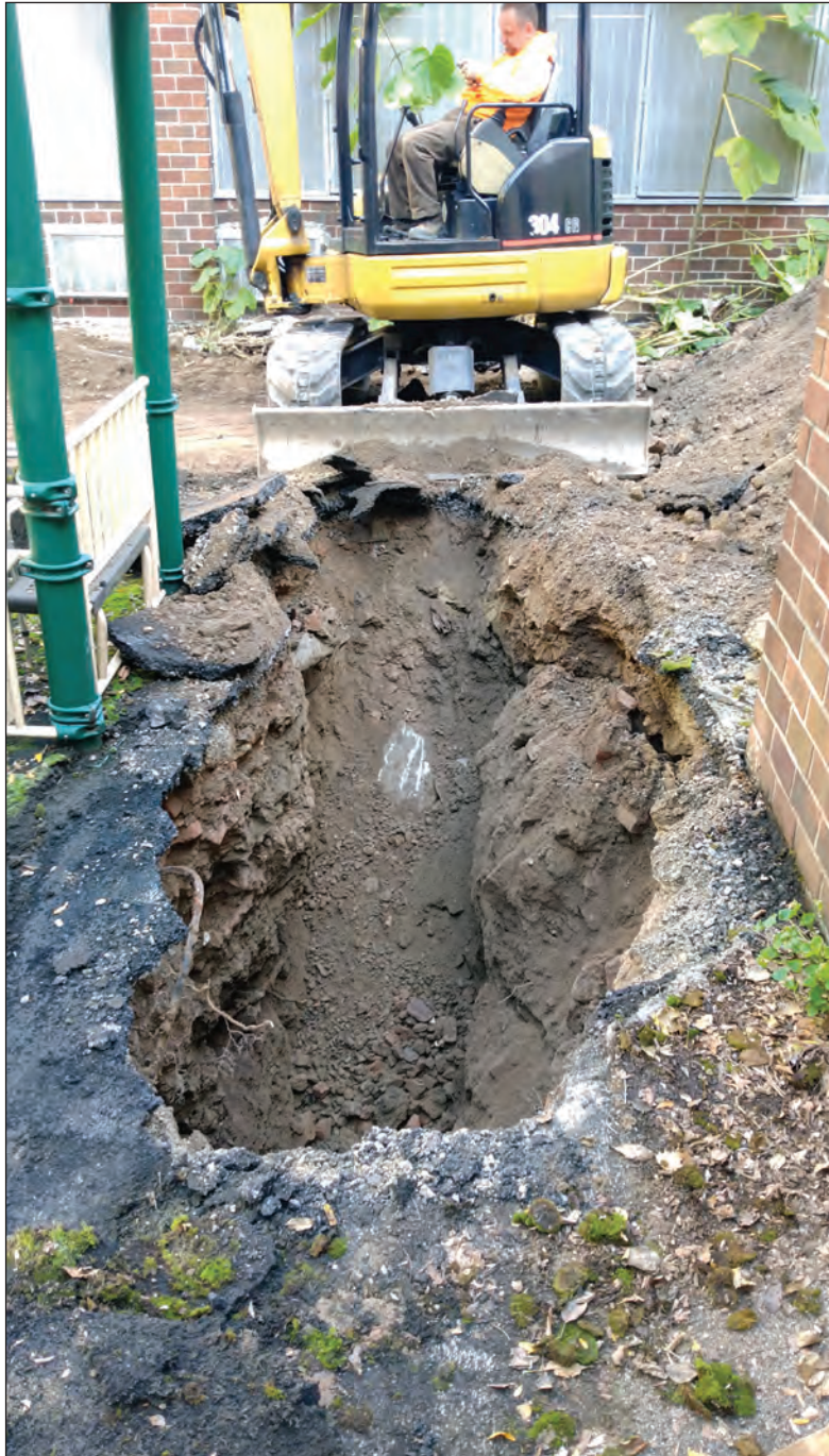
Facing northeast showing excavation of Trench 4. Note collapsing trench walls consisting of loose urban fill and brick demolition debris. A foundation was encountered at a depth of approximately 8 feet below ground surface in this trench though it was immediately obscured by collapsing walls. 15
