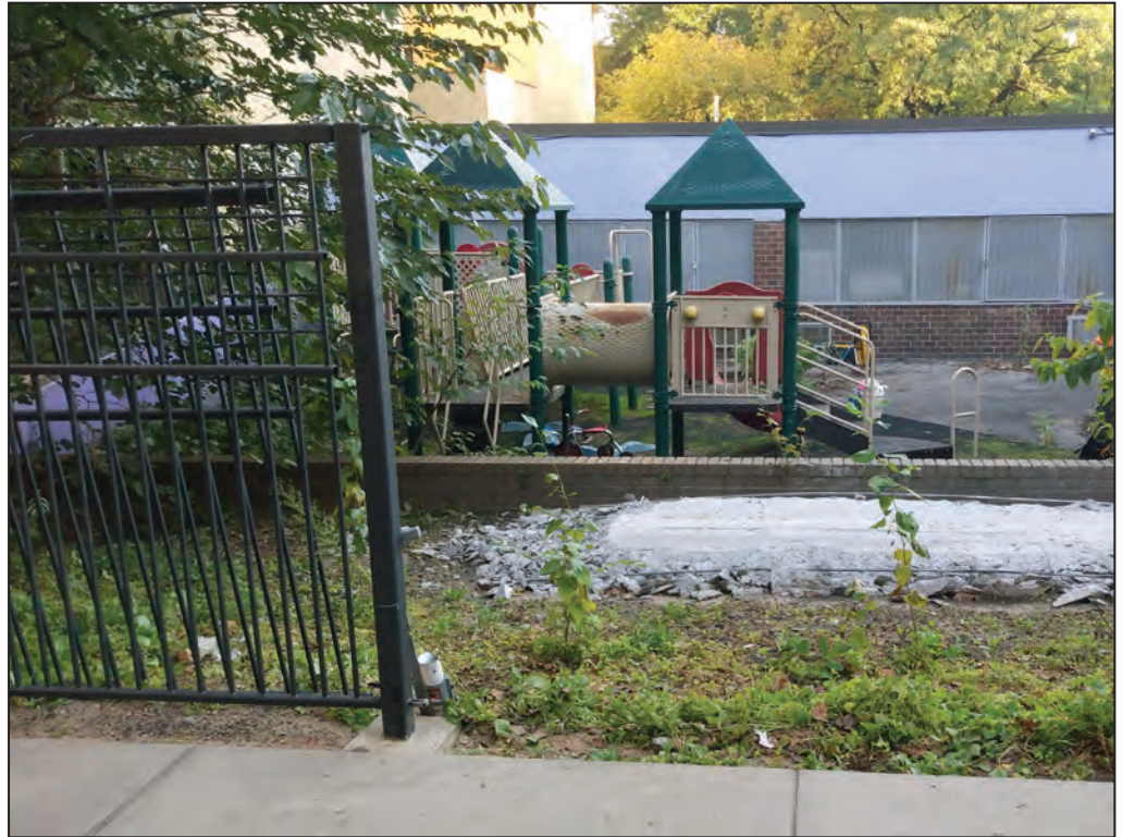
Facing northeast from public walkway toward rear yard of 145 Broome Street. Note higher elevation area in foreground and retaining wall and then drop in elevation of three feet, closer to the 1-story brick building 1
