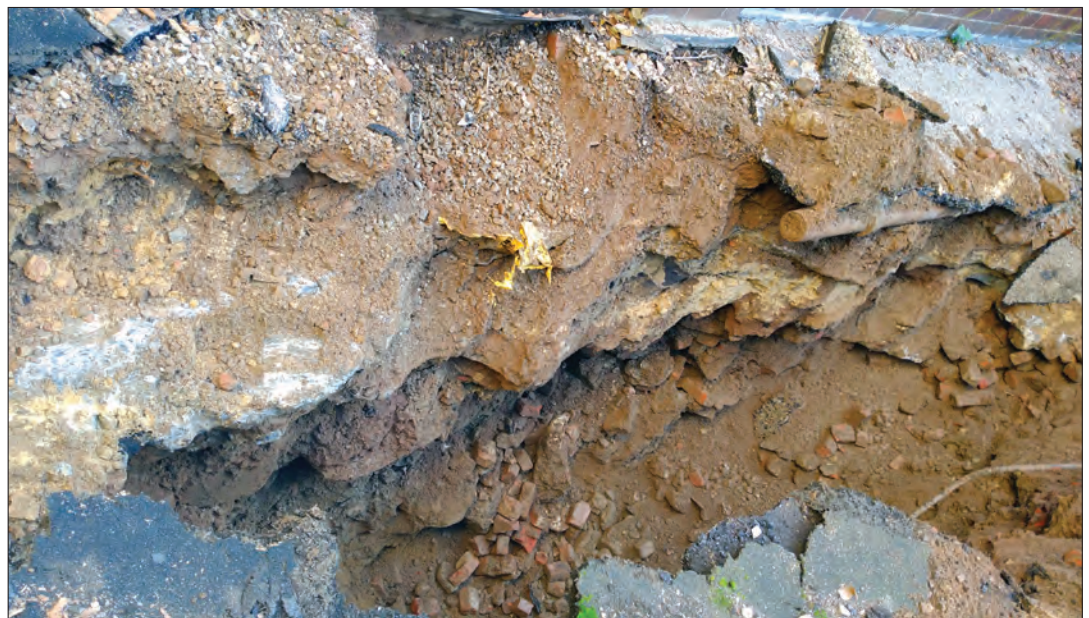
Detail of the north wall of Trench 1 showing collapsing soils undercutting the adjacent building's foundation
