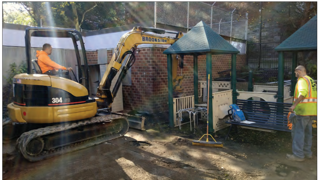
Facing south towards location of Trench 4, which was excavated adjacent to the rear wing of the 1-story brick building
