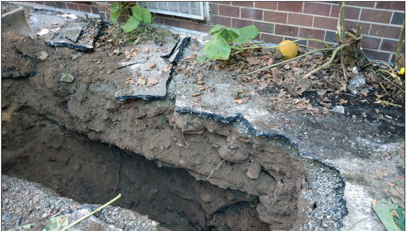
Facing northwest towards Trench 3 showing drainage line approximately 1.5 feet below ground surface and loose sandy urban fill and brick demolition debris 12
