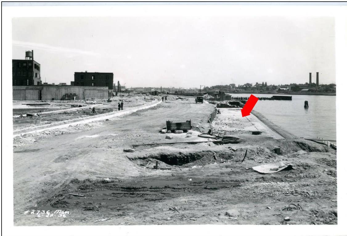
Photo 13. General view N from point on center line of E 100 St. showing roadway construction and a relieving platform (arrow). (No. 2736 6-22-36)
