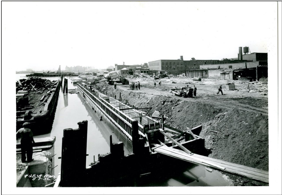
Photo 9. View S from pier at the end of E 107 th St. pouring concrete for bulkhead and also in the area of the roadway (No. 2838 8-7-1936)
