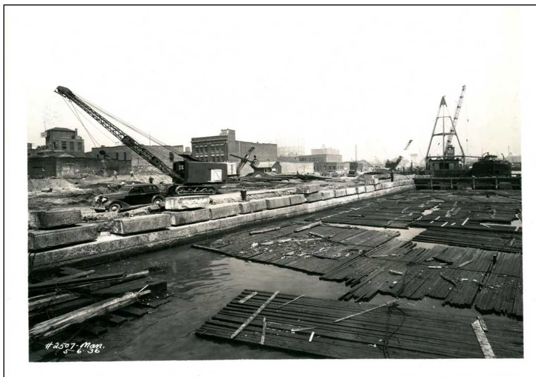
Photo 8. East River Drive. Bulkhead N of E 103 St. showing displaced top cord of granite block in original bulkhead. (No. 2505 5-6-1936)
