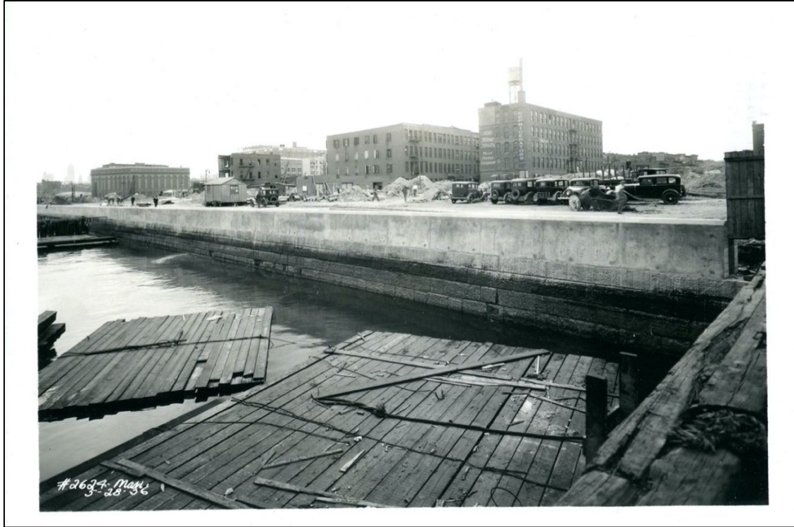
Photo 11. View S from a point on pier at E 103 St. showing new concrete bulkhead in place over old granite bulkhead. (No. 2624 3-28-1936). This can be seen today in some areas of the seawall.
