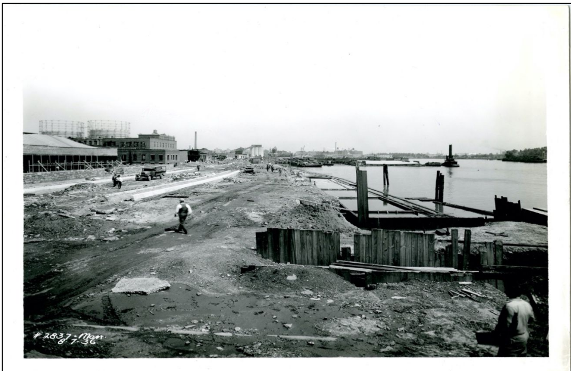
Photo 14. View N from a point on line of E 104 St. showing granite curbs and relieving platforms placed for bulkhead. (No. 2837 8-7-1936)
