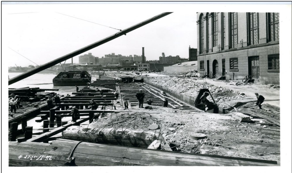
Photo 12. General view S along bulkhead from point on center line of E 96 St. (No. 2731 6-22-1936). The Metropolitan Power House is to the right.
