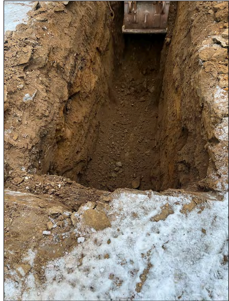
Same view after excavation to a depth of 10 feet below the ground surface 2
