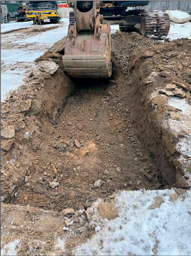
Looking east at the excavation in the southeast yard of the church, showing natural soils emerging approximately 3 feet below a layer of rubble 1
