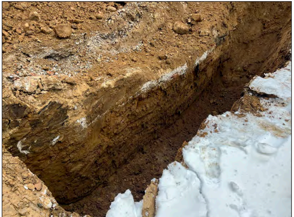
Looking southeast at the former foundation wall, showing disturbed soils adjacent to the wall
