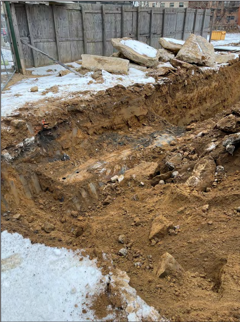
Looking northwest across the excavation at the southwest corner of the former church, showing the utility obstruction in the center and natural soils to the east (bottom right) and north (top right) 3
