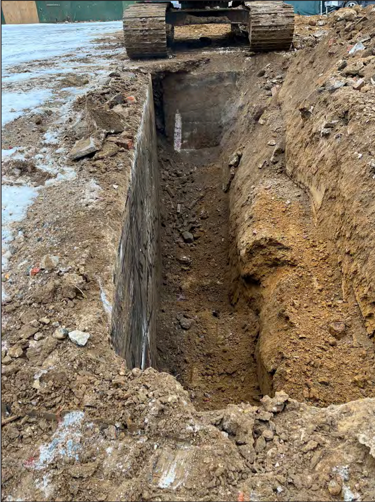
View south of the excavation between the foundations of the former church and gymnasium, with foundation walls visible in the east (left) and south (top) walls of the excavation 7
