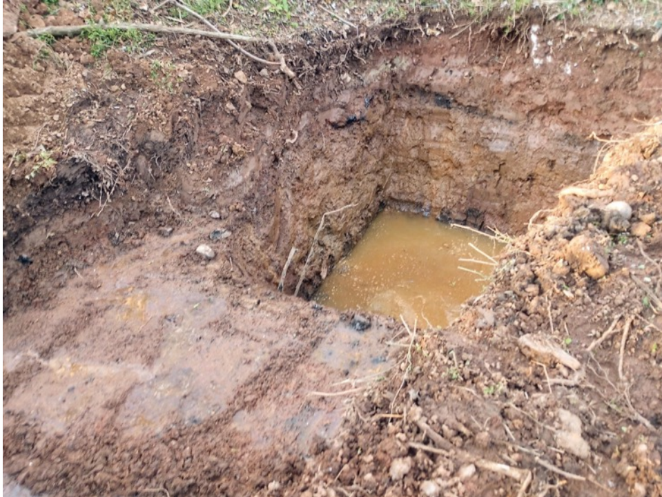
Photograph 12. Overnight groundwater intrusion in southwestern half of Trench 2.
