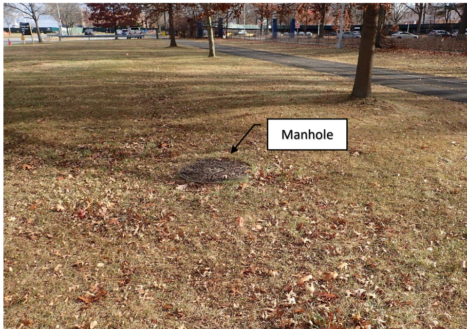
Photograph 10. View of a "NYC Electrical" manhole near ST 12. Facing east. (LC 12/3/2024)
