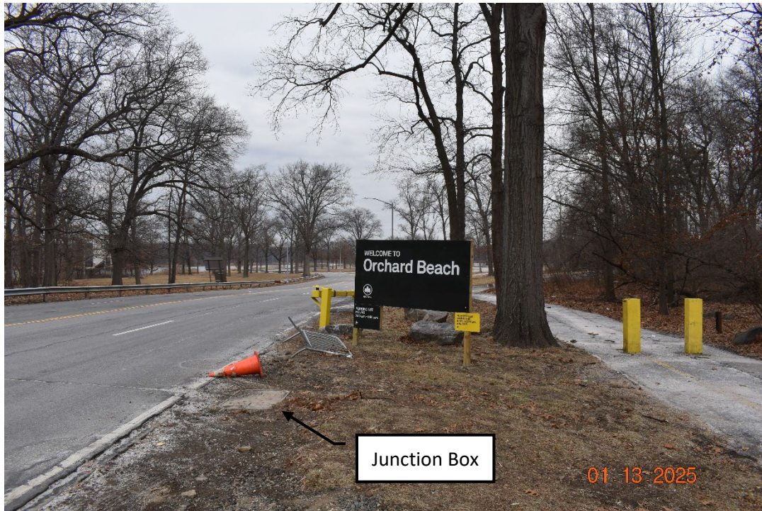
Photograph 18. View of a junction box near ST 36 location. Facing north (NC 1/13/2025).
