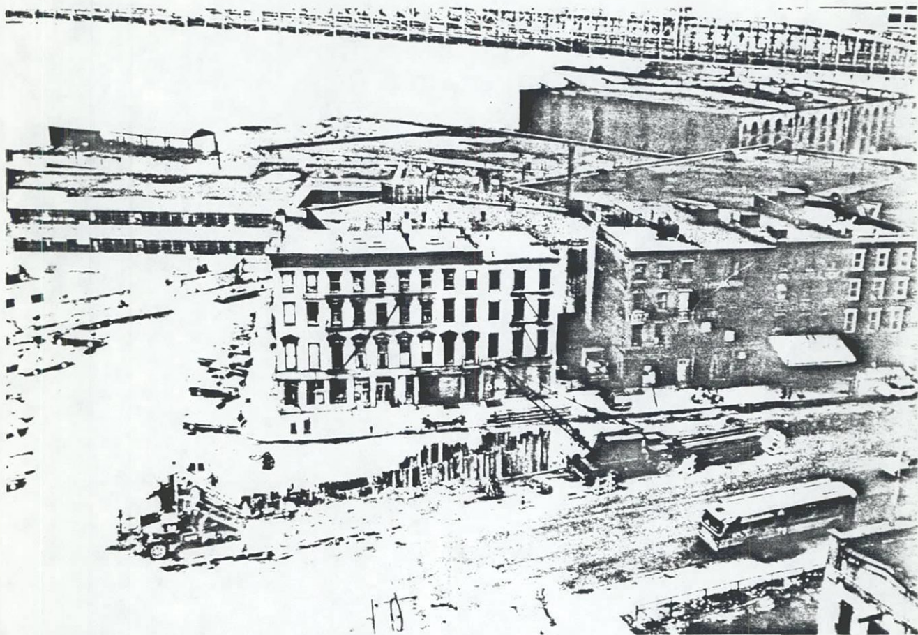
Figure 3. The Fulton Street sewer excavation. Looking north with the Brooklyn Bridge in the background.
