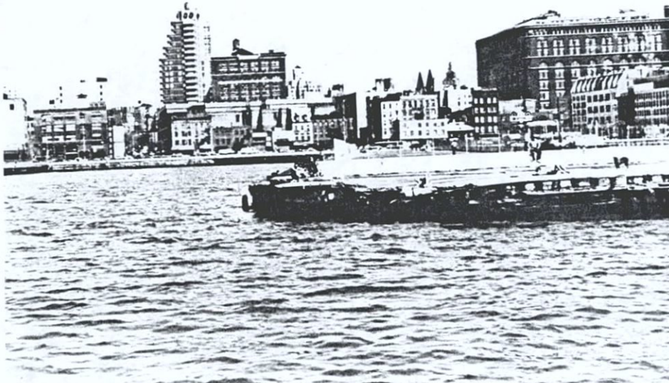
Bulkhead, Pier 45 Note condition of pilings. View from the Hudson River facing east 4/27/89
