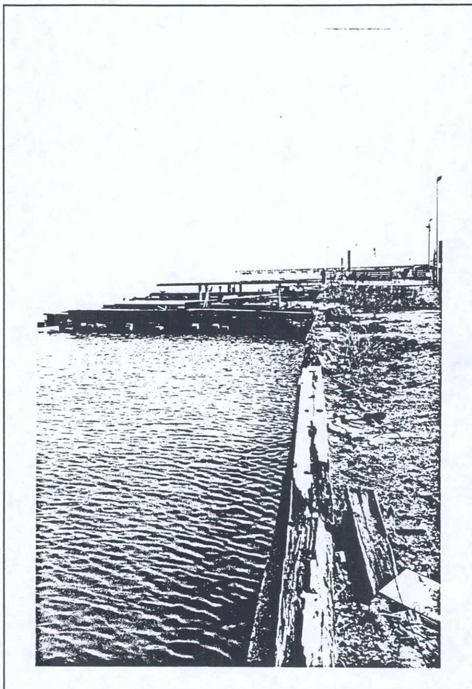
85. Piers 67 and 68, and 28th Street Floatbridge West Street between West 27th and 29th Streets View North of Floatbridge Approach and Remains of Piers New York County
