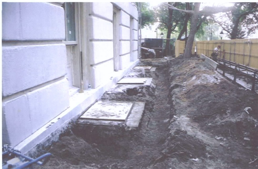
Photo 10. View east of trench monitoring along the south wall of the courthouse (east corner).
