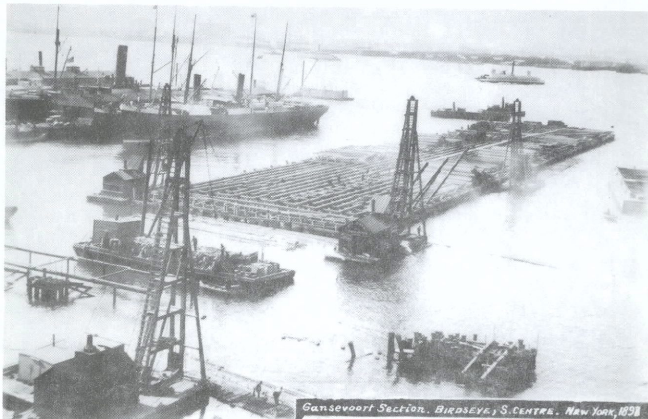
FIGURE 70. Construction of pier 48, W. 11th Street, Gansevoort Piers, 1897-98 (Collection of the South Street Seaport Museum).
