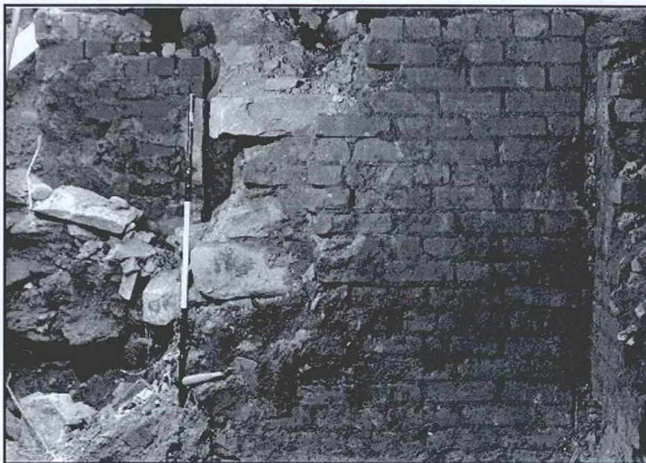
Plate 7. Structure 1, north-south portion of the brick wall at the intersection with the east-west portion of the wall. Looking west.
