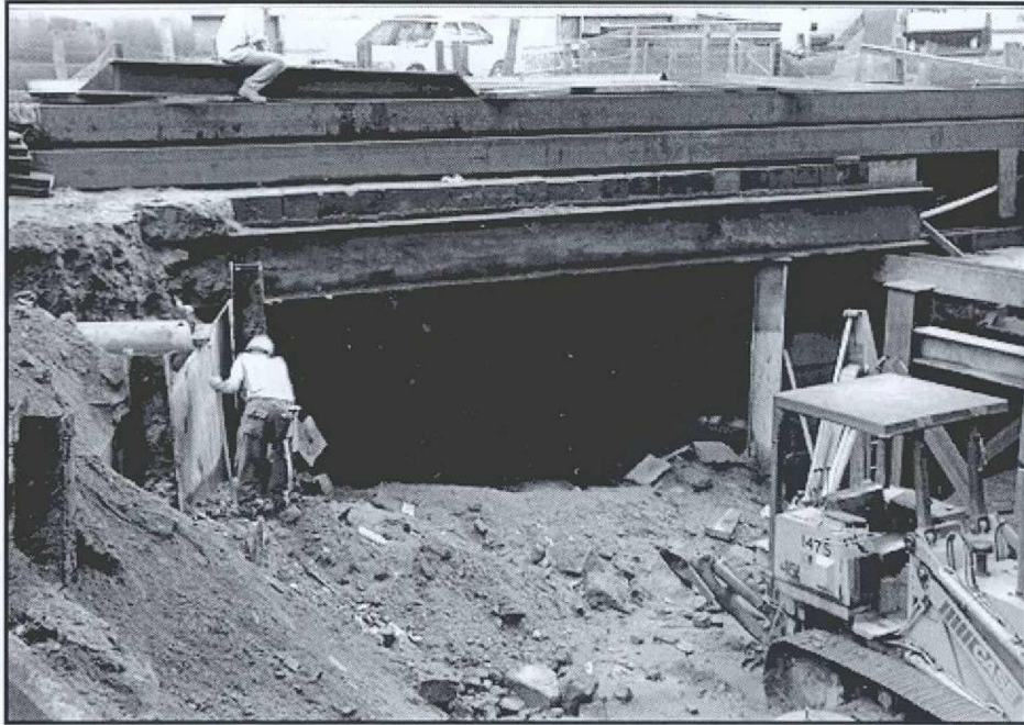
Plate 3. Entrance to the tunnel excavation under Pearl Street early in the project. Looking north.
