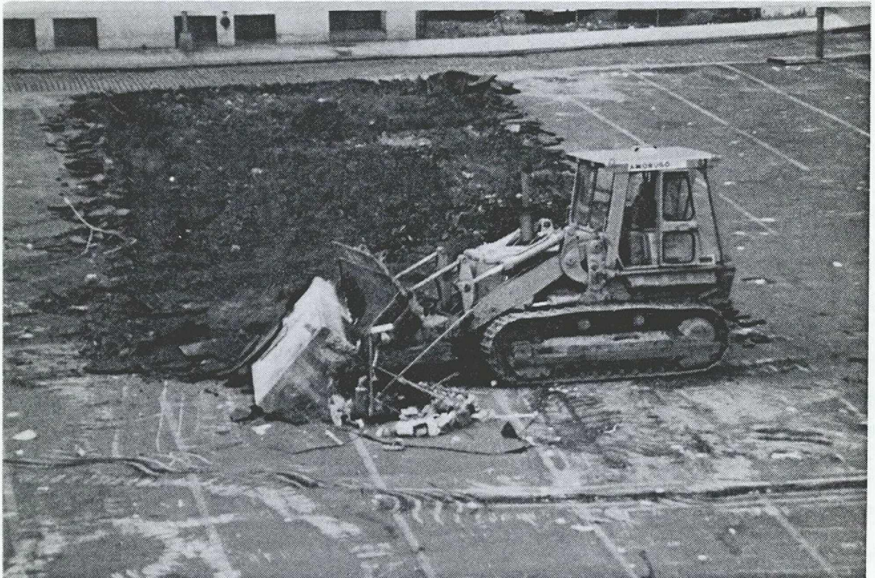
Plate 3.1: Parking lot surface broken by a 977 loader and operator in preparation for archaeological investigation of the 175 Water Street block (Block 71). Asphalt removal began on October 28, 1981.
