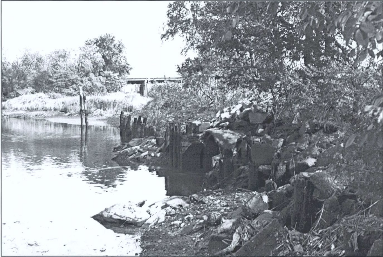
Figure 28. Long Island Railroad embankment bulkheading and culvert, facing east. Flushing Bay Ecosystem Restoration Project, Queens County, New York (Pickman 2002).
