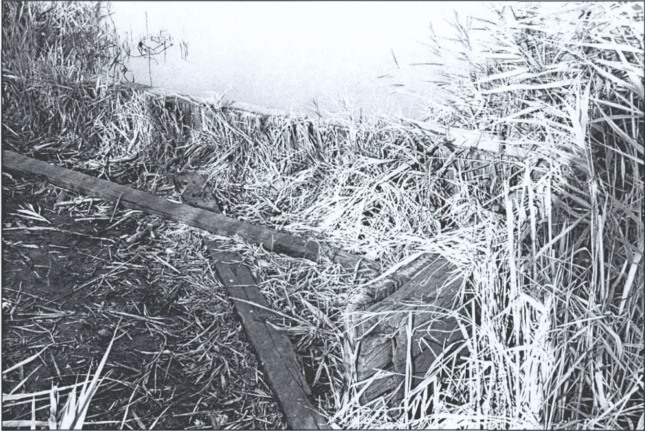
Figure 75. Remains of wooden wharf at the northwestern end of Willow Lake, facing northeast. Flushing Bay Ecosystem Restoration Project, Queens County, New York (Pickman 2001).
