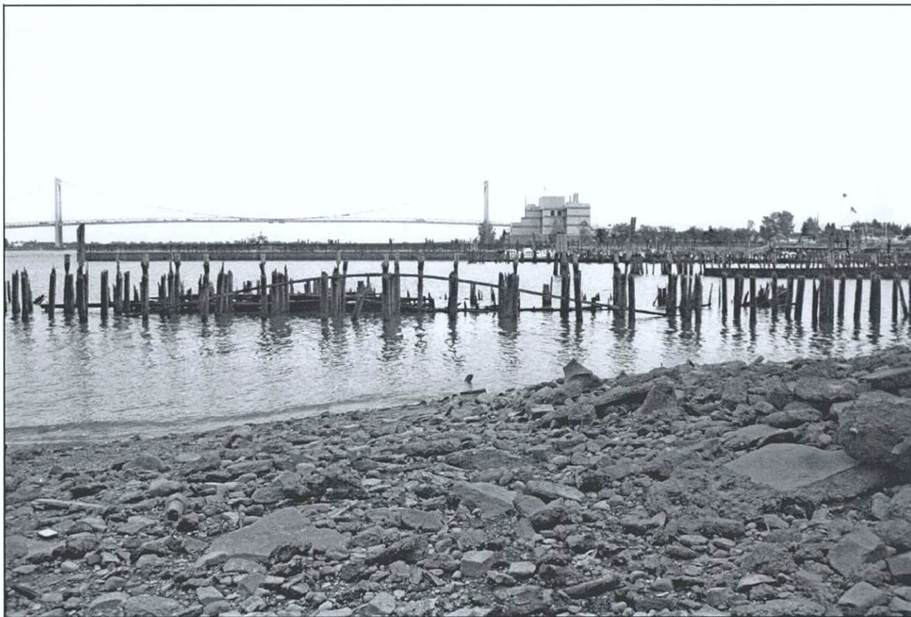
Figure 111. Northern end of Shipyard Feature H; Feature I behind Feature H, Feature F in background at right, facing east. Flushing Bay Ecosystem Restoration Project, Queens County, New York (Pickman 2002).
