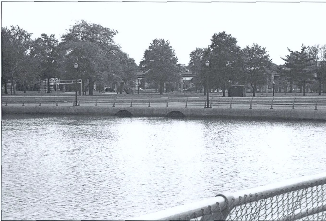
Figure 53. Culverts entering south side of Flushing Meadow Park, facing southeast. Flushing Bay Ecosystem Restoration Project, Queens County, New York (Pickman 2002).
