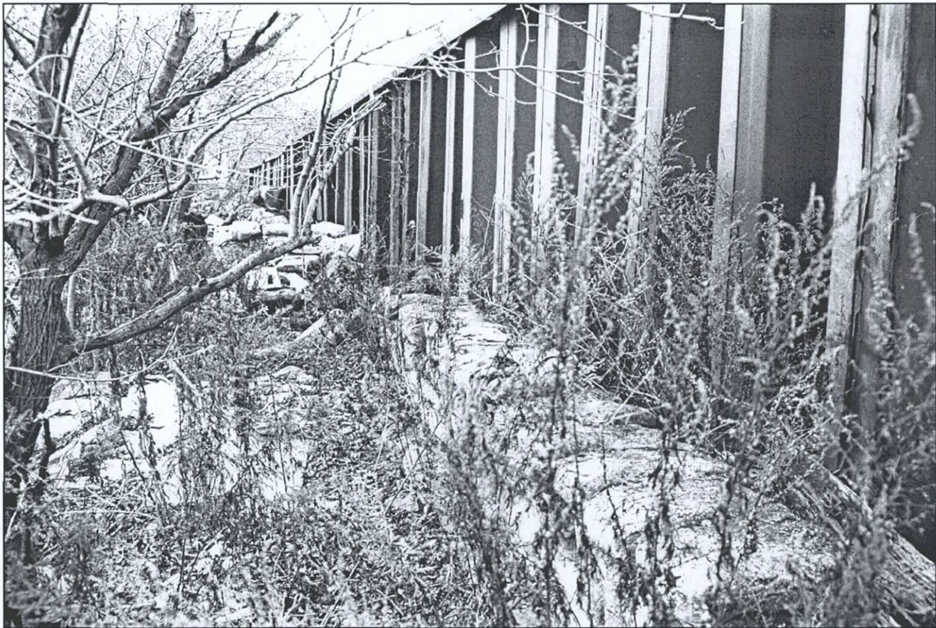
Figure 79. Stone wall and steel bulkhead in western portion of LaGuardia Airport South Shore, facing west. Flushing Bay Ecosystem Restoration Project, Queens County, New York (Pickman 2001).
