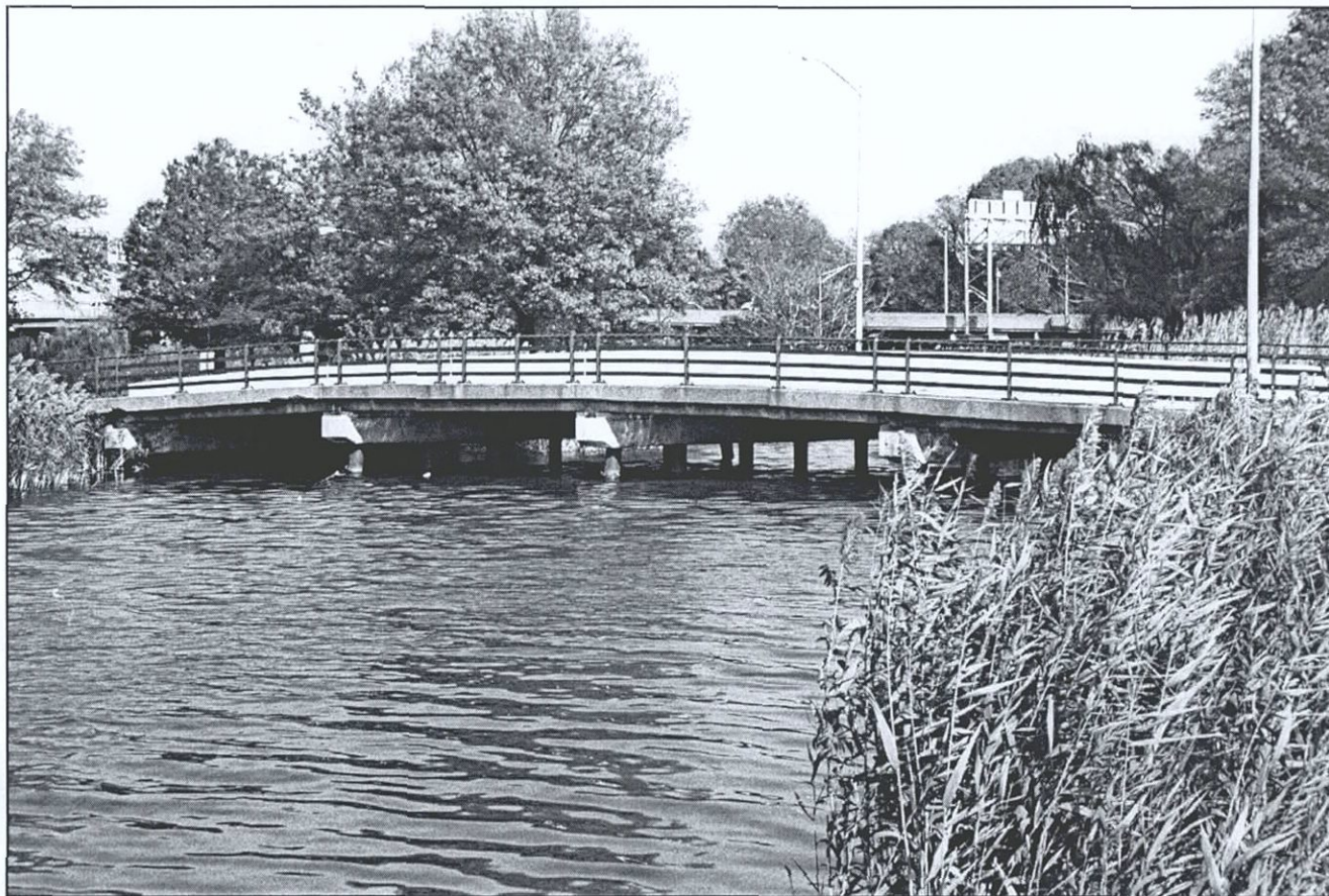
Figure 73. Bridge over Meadow Lake outlet stream, facing northwest. Flushing Bay Ecosystem Restoration Project, Queens County, New York ( Pickman 2001 ).
