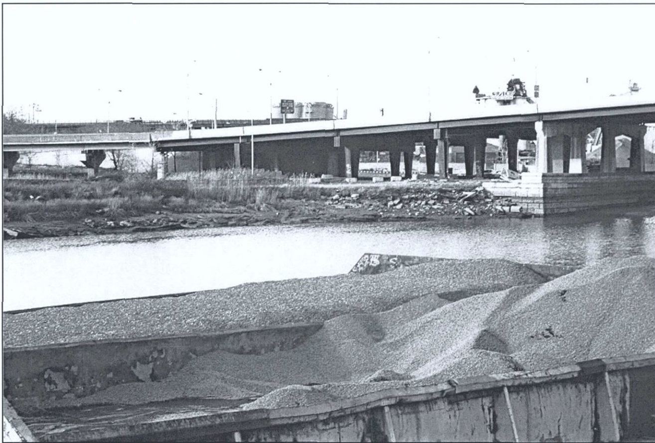
Figure 20. Close-up of pier on west side of Northern Boulevard Bridge, facing northwest. Flushing Bay Ecosystem Restoration Project, Queens County, New York (Pickman 2001).
