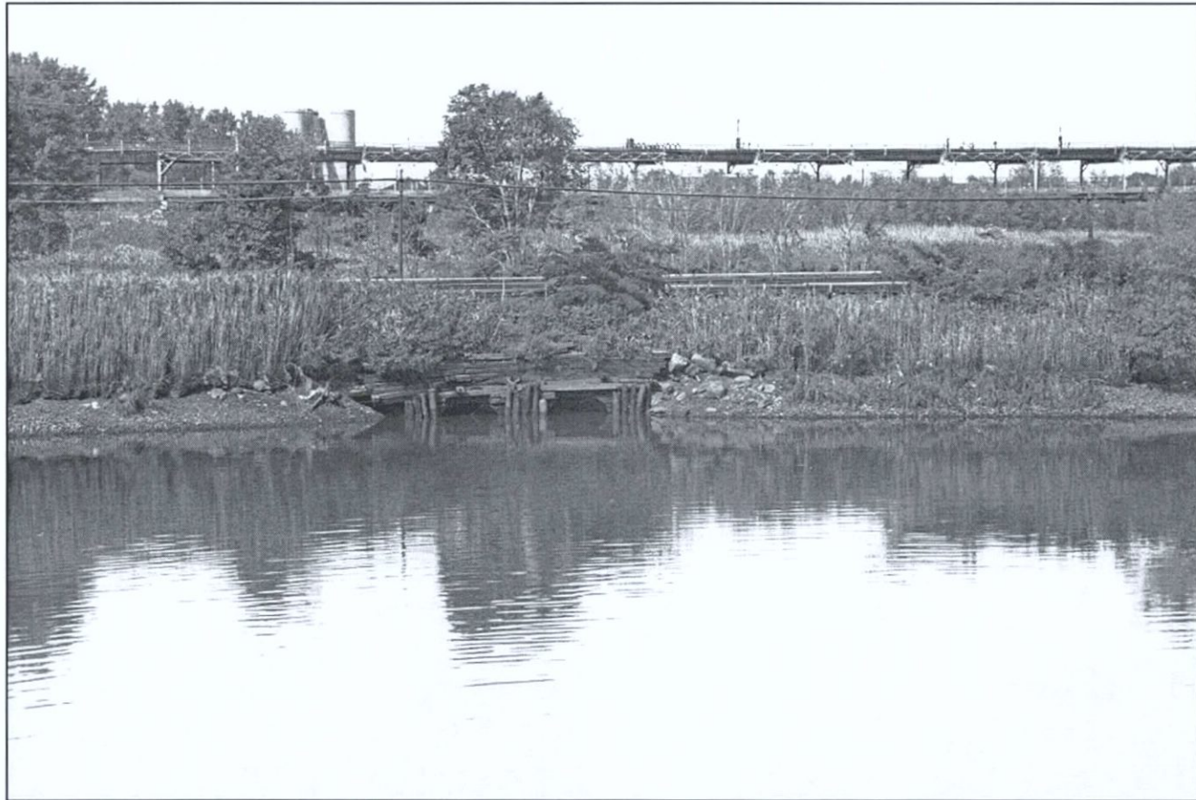
Figure 27. Long Island Railroad embankment and culverts under embankment, Roosevelt Avenue Bridge in background, facing northwest from east bank of Flushing Creek. Flushing Bay Ecosystem Restoration Project, Queens County, New York (Pickman 2002).
