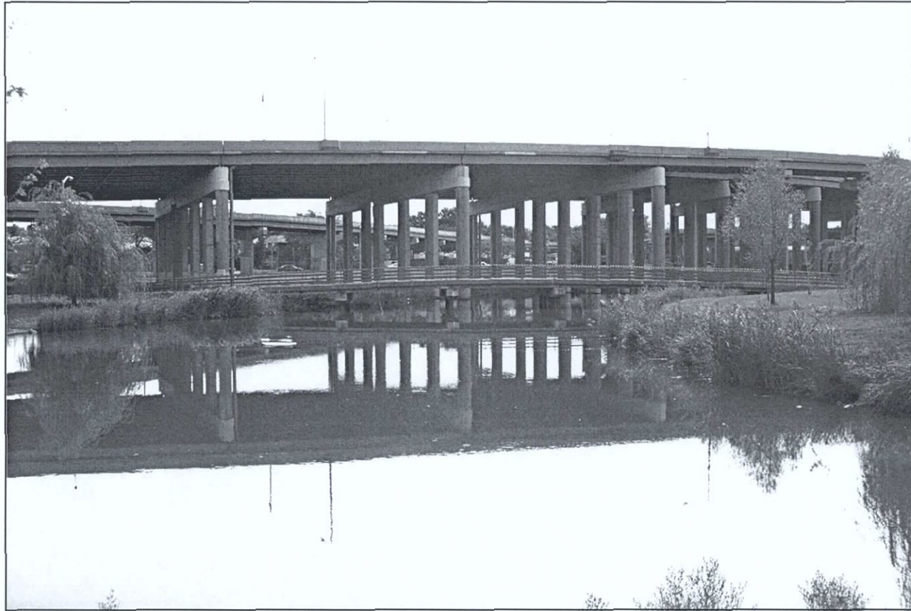
Figure 54. Bridge over Flushing Creek immediately north of Long Island Expressway Park, facing south from southern end of Daylighting project area (Pickman 2002).
