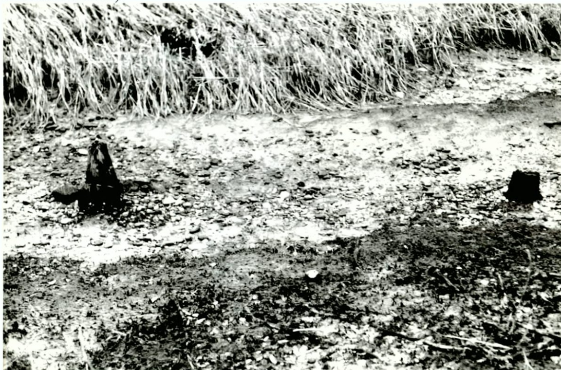
Figure 120. Decayed pilings on north shore of Motts Point, facing north. Jamaica Bay Restoration Project, Kings, Queens and Nassau Counties, New York (Pickman 1999).
