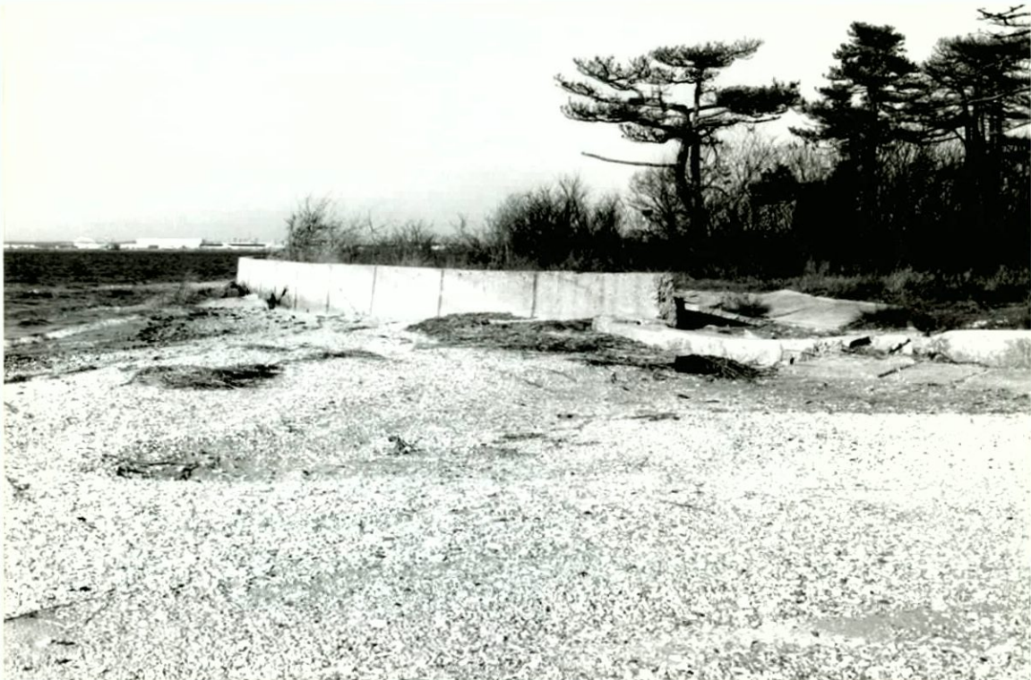
Figure 114. Remnants of concrete seawall at Motts Point, facing northeast. Jamaica Bay Restoration Project, Kings, Queens and Nassau Counties, New York ( Pickman 1999 ).
