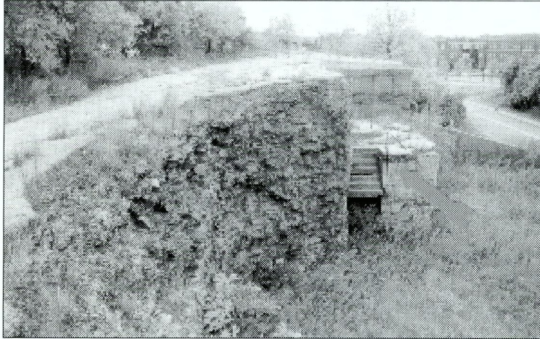
Figure 6.107 Detail of Duane showing extensive crumbling of concrete and the establishment of vegetation throughout. Arrow identifies ruins of handrail and stair.
