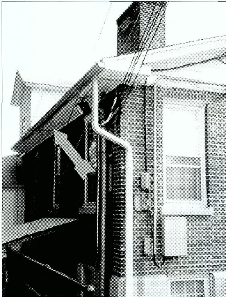
Figure 6.119 Utility wires, control boxes haphazardly mounted, northwest corner. Arrow identifies peeling paint; signals poor water drainage from roof. Extensive reporting of chimney and rust staining seen on foundation wall.
