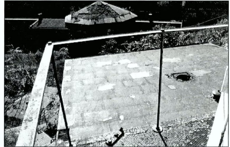
Figure 6.38 View of sheet-metal roof on the lighthouse showing general poor condition and rusting of ferrous metal surfaces.
