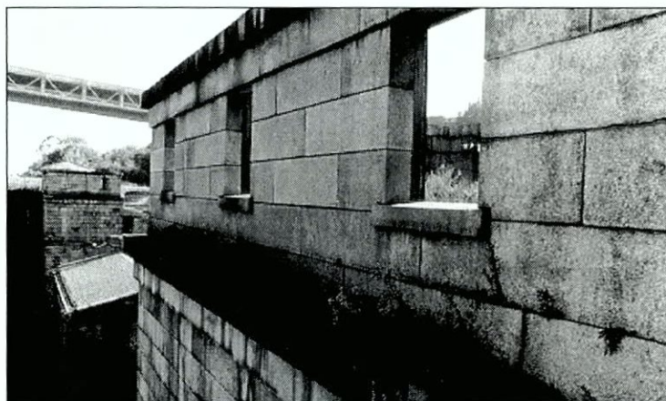
Figure 6.21 North magazine showing vegetation growing out of deteriorated joints. Magazine interiors exposed to the elements due to lack of roofs or window units.
