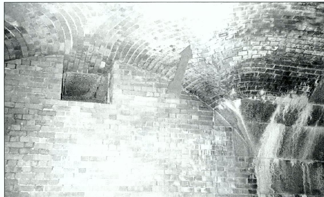
Figure 6.29 Original brick vault at south magazine showing major efflorescence (arrow) and calcite leaching through granite joints. Extensive loss of mortar from brick joints.
