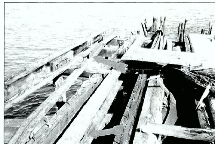
Figure 6.48 Detail of dock end showing deteriorated and unsafe condition of decking. Arrows identify extensive corrosion of I-beams.
