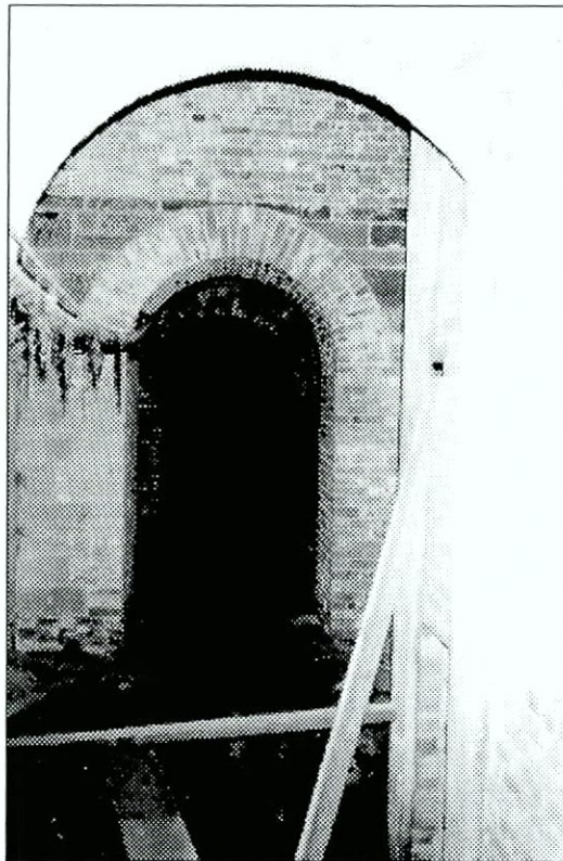
Figure 6.97 View through counterscarp gallery showing dismantled plank flooring and suspended electric cable.
