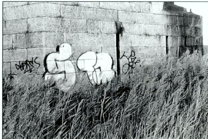
Figure 6.14 Spray-paint graffiti at southeast corner of Battery Weed
