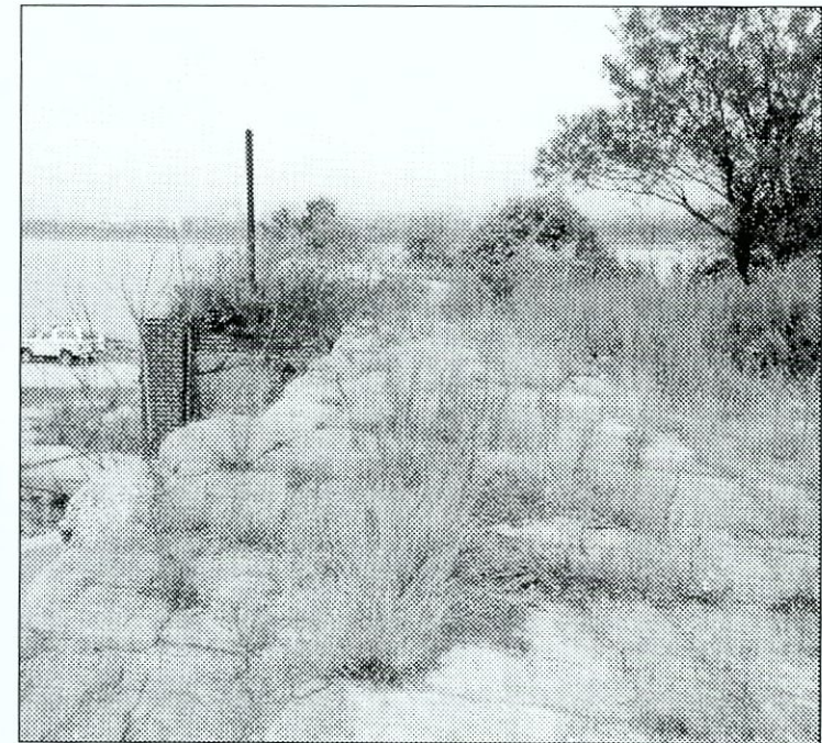
Figure 6.108 Detail of unwanted vegetation growing out of cracks in concrete at top of battery. Wall edge is very unstable.
