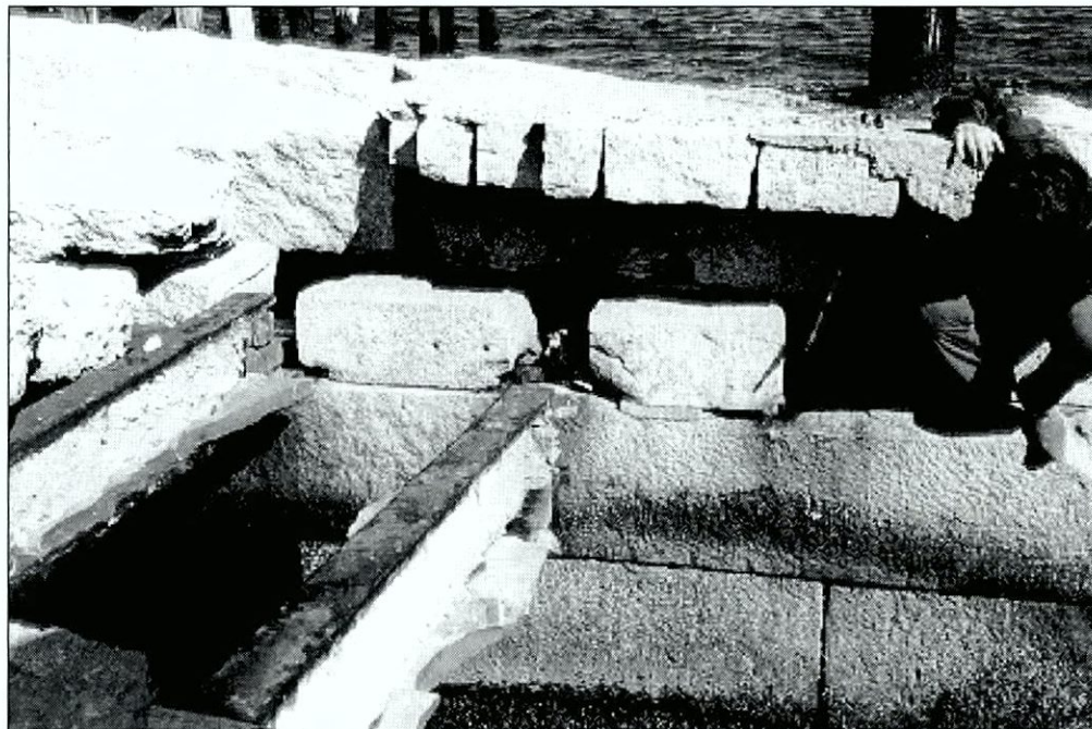
Figure 6.46 Detail of dock showing failure of steel I-beam and granite shelf connection caused by the gradual movement of the wall towards the water. Note corrosion of I-beams.
