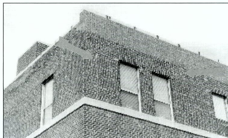
Figure 6.148 Detail of southwest corner showing earlier rebuilt parapet with bitu-mastic repairs made to coping-stone joints. Arrows identify structural cracking (and subsequent filling).
