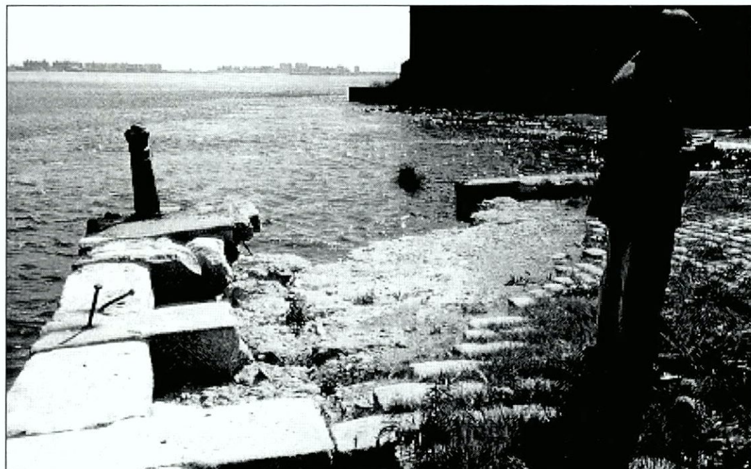
Figure 6.47 North dock at northeast corner showing area where granite pavers have been removed. End blocks are gradually slipping into the ocean.
