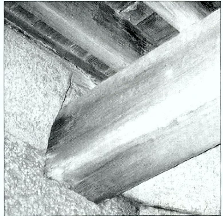
Figure 6.31 Detail of wood beam and stone pocket located near south magazine; presence of wood rot and formation of water-borne deposits originating from the granite masonry.
