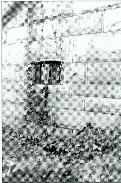
Figure 6.83 Unwanted ivy growing on granite facade and cast-iron shutters of Fort Tompkins counterscarp. Light green biological growth evident to the left of the window (arrow).
