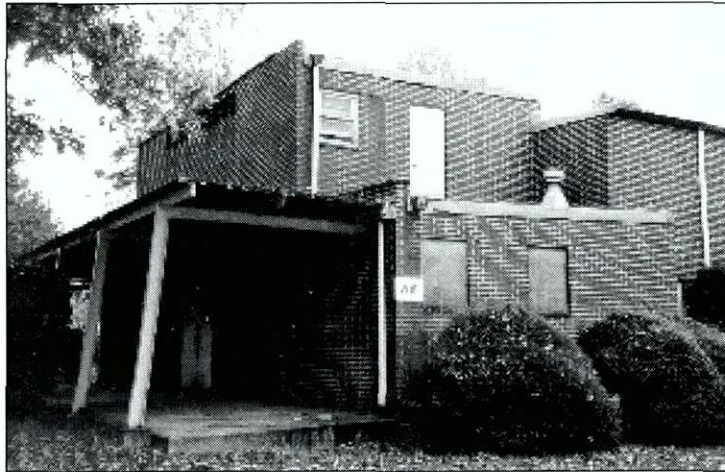
Figure 6.178 North and east (main) facade showing boarded windows, rusting porch and faulty downspouts.
