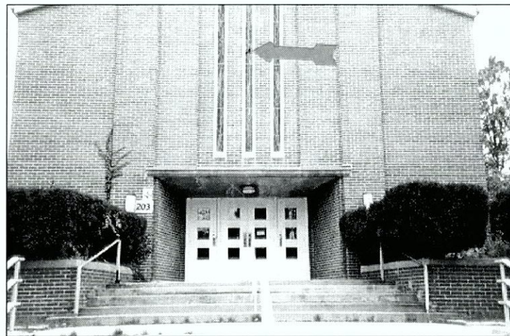
Figure 6.174 Main entrance. Note cracking in the concrete canopy caused by water infiltration through the faulty roof. Note vegetation growing out of sidewalk and step joints. Arrow identifies broken colored glass in window.
