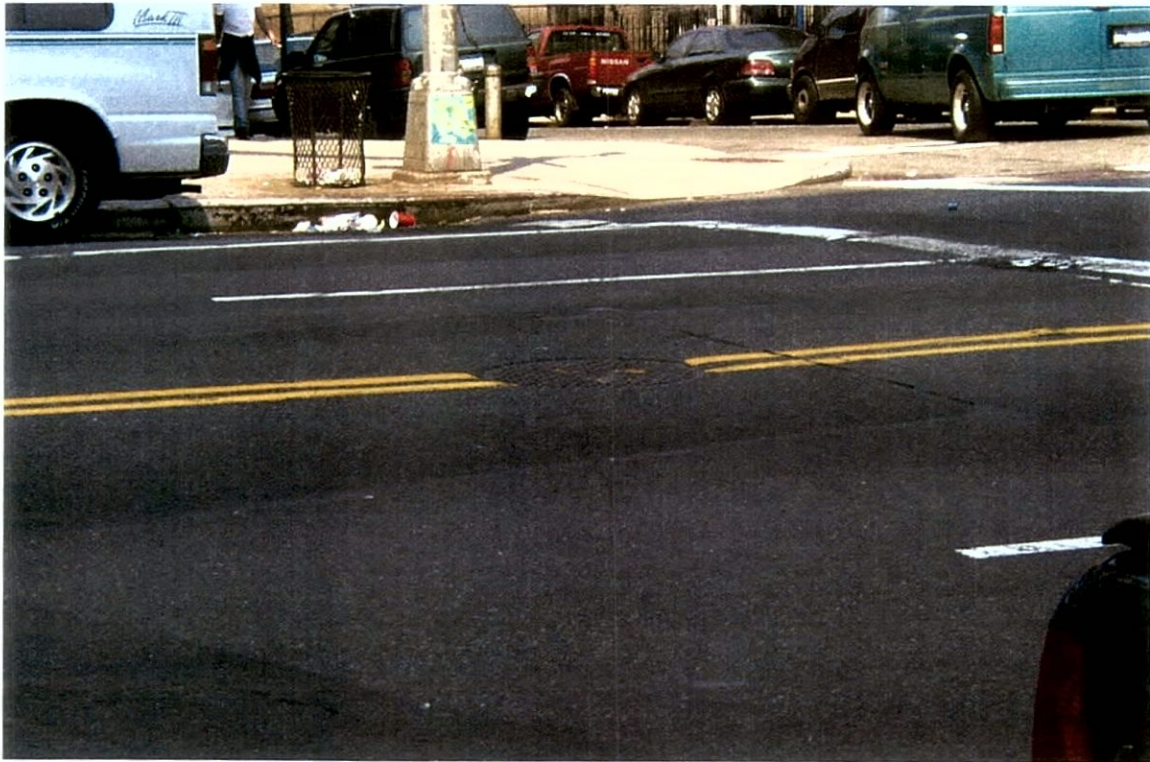
Photograph 29-1: Looking west toward the centerline of Amsterdam Avenue between 156 th and 157 th Streets—Shaft Site 29.
