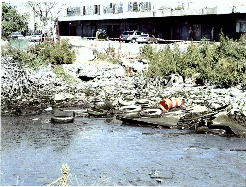
Photograph 16: Eastern end of Slip 5, with deteriorated bulkhead and trash. View looking northeast.
