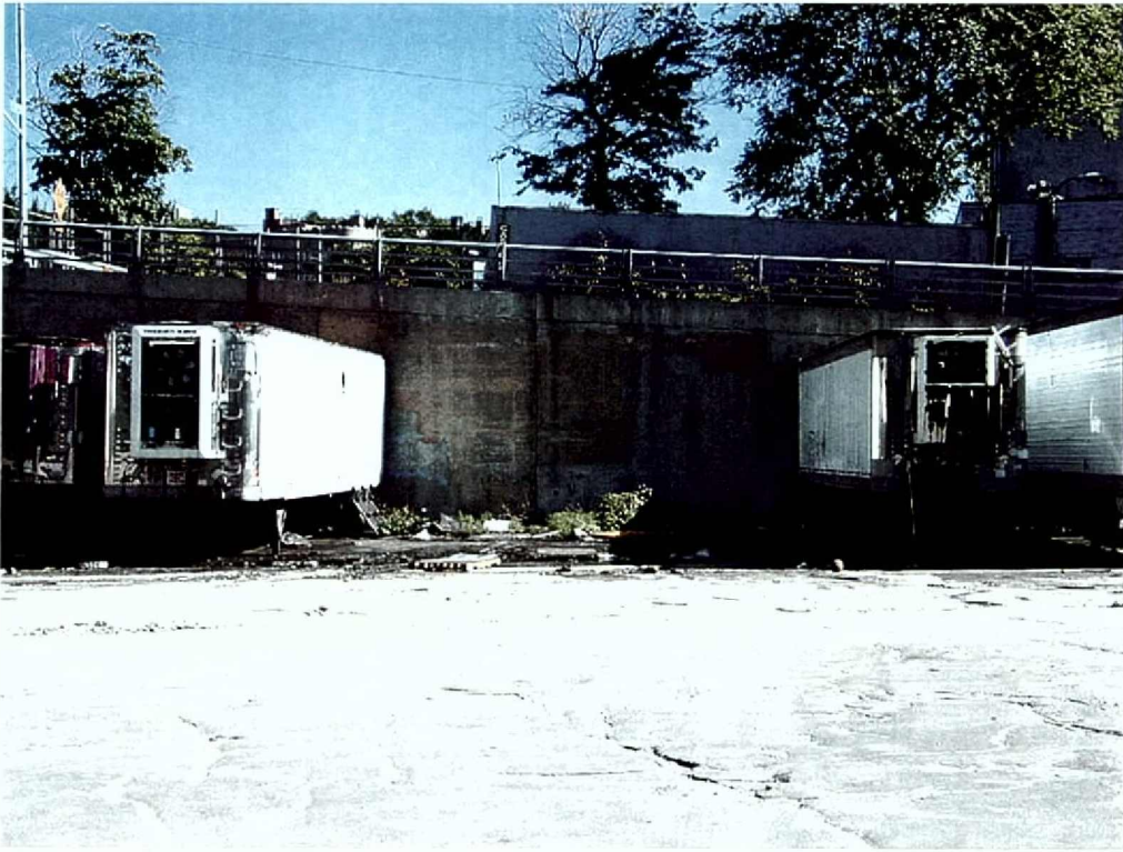
Photograph 11: Concrete retaining wall supporting Cromwell Avenue just north of the Bronx House of Detention. View looking southeast with the parking lot east of Building B in the foreground.
