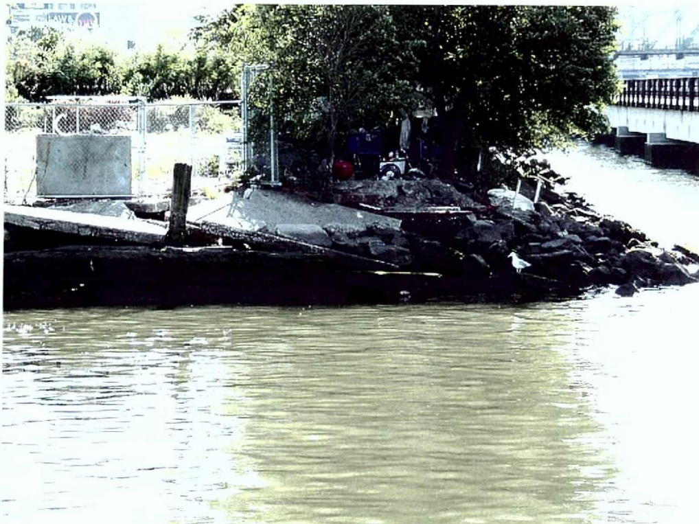
Photograph 15: Western end of Pier 2, with deteriorated bulkhead and trash. View looking southwest.
