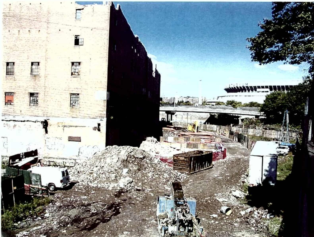
Photograph 12: Building A being demolished and disturbed ground surface. View looking northwest with Yankee Stadium in the background.
