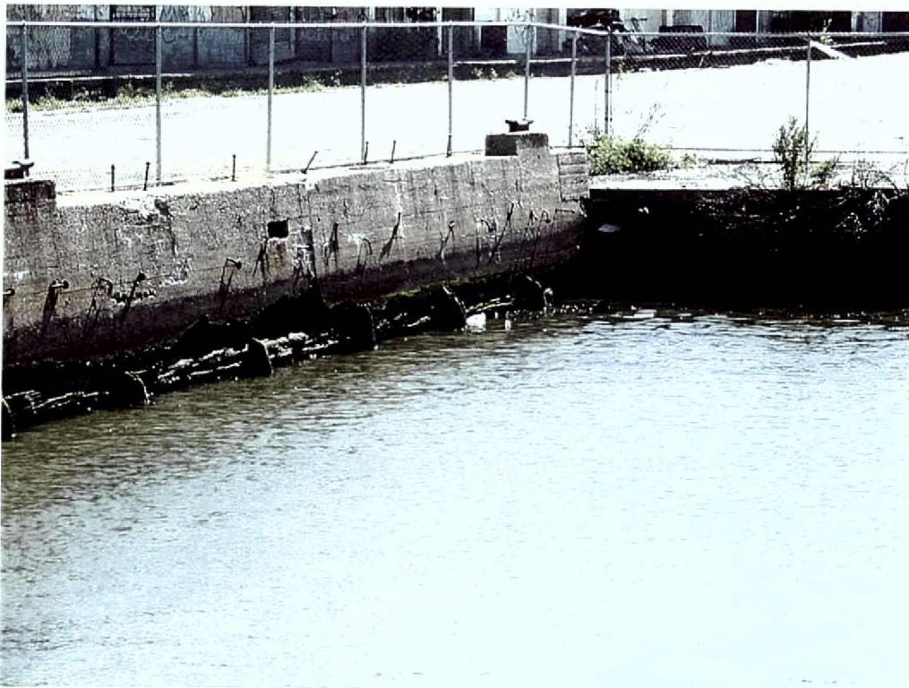
Photograph 14: Pier 2, with wooden elements at water line and concrete elements above. View looking southeast.
