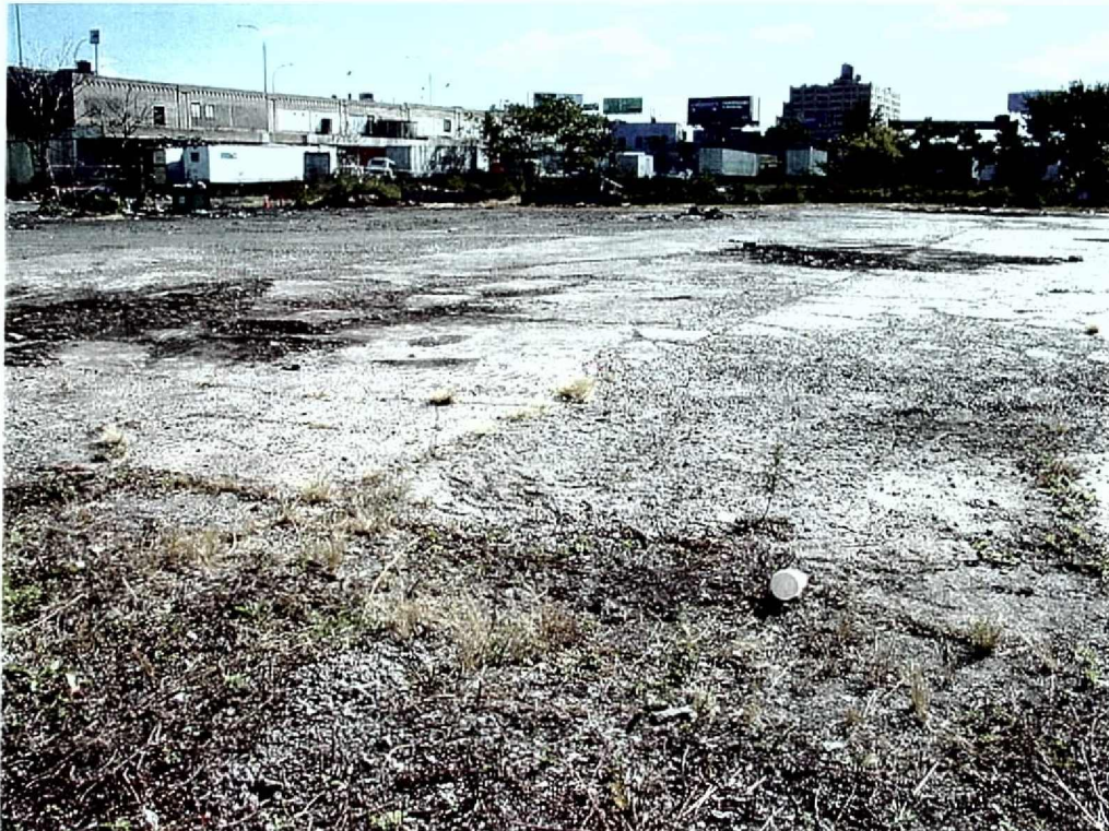
Photograph 17: Surface of Pier 4, showing uneven surface. View looking southeast with Building F in the background on the left.
